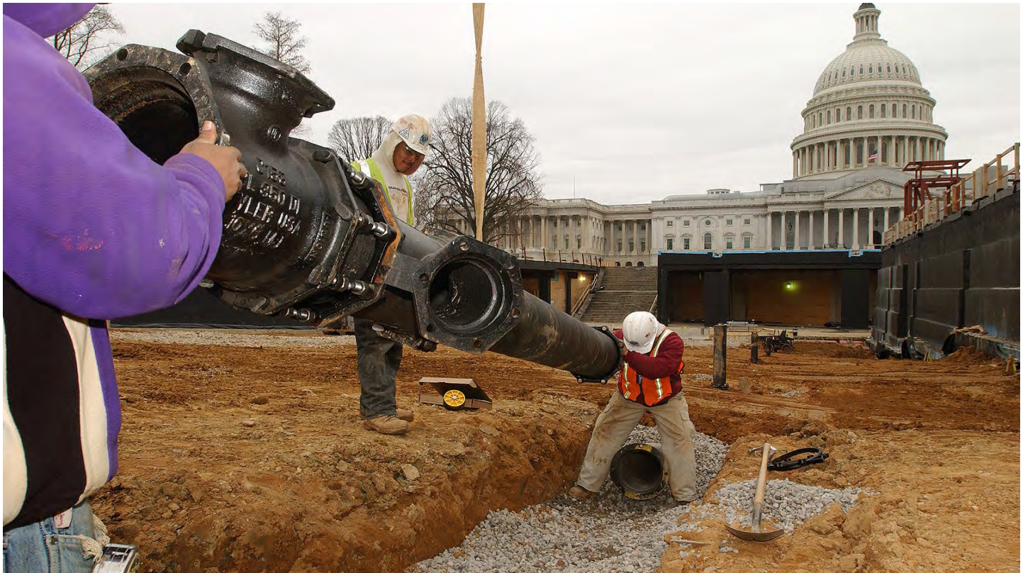
Workers install a storm drain pipe in the sloping ground leading to the CVC entrance on the south side of the site. The pipe is part of an elaborate drainage system that will intercept water before it reaches the CVC entrances and monumental stairs at the base of the slope (center right).
