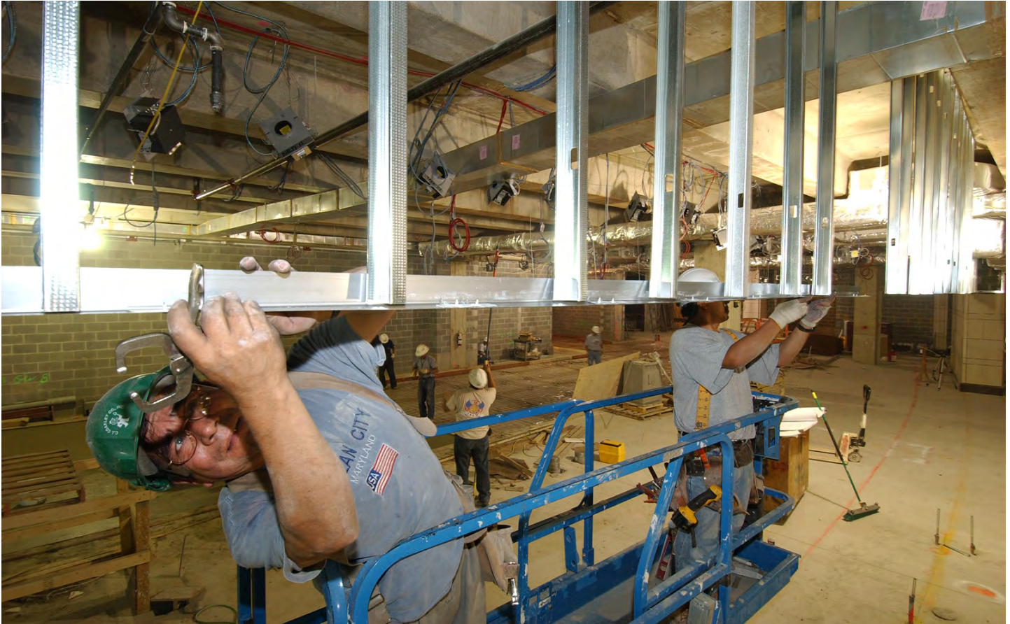
Workers install metal framework that will help support a portion of the ceiling grid inside the CVC food services area.
