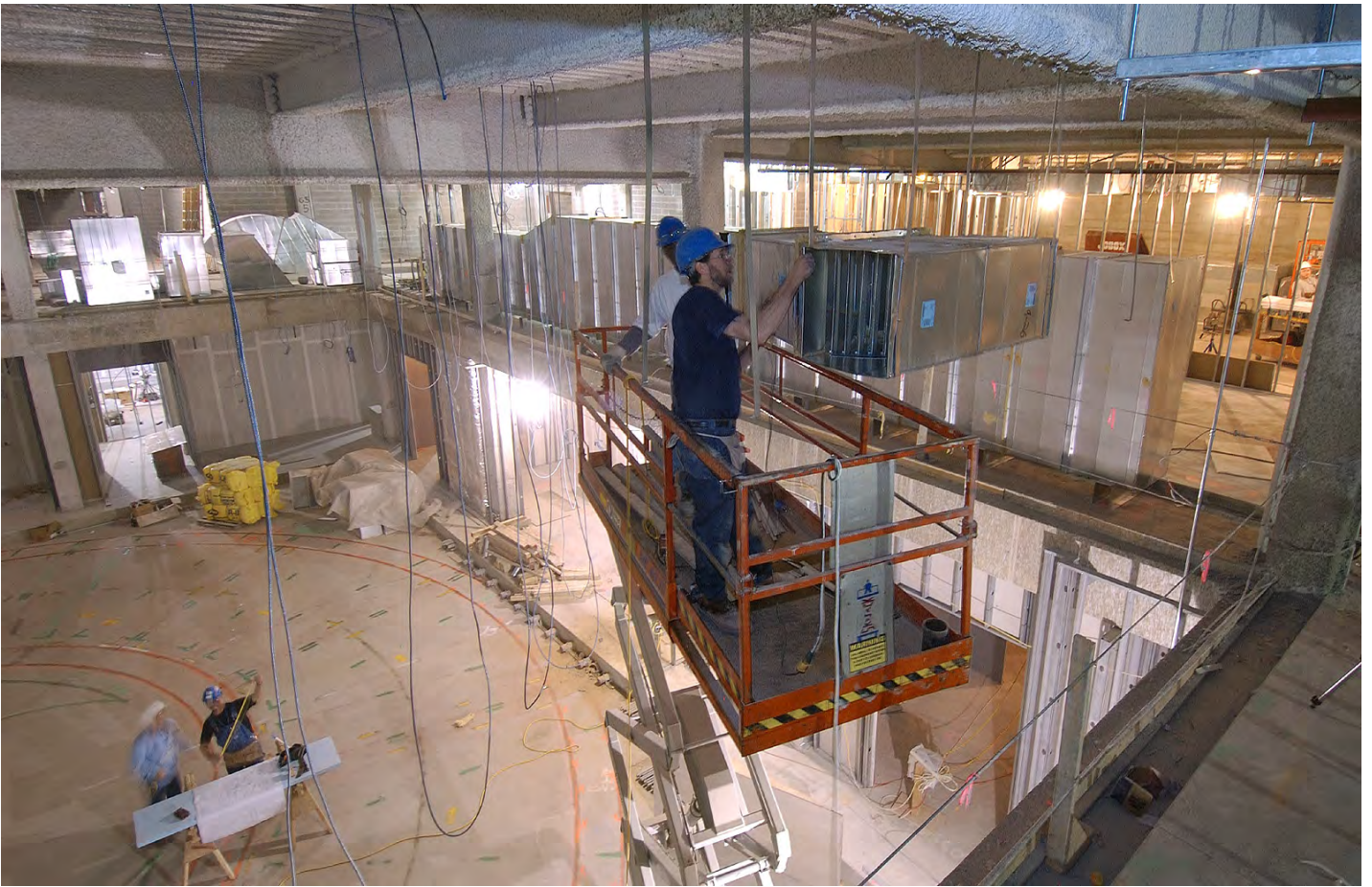
Workers in the House expansion space position a segment of air duct into place in the ceiling of a new committee hearing room. The curving lines visible on the floor will be used to help guide the construction of the ceiling structure, which will support a series of concentric curving vaults.
