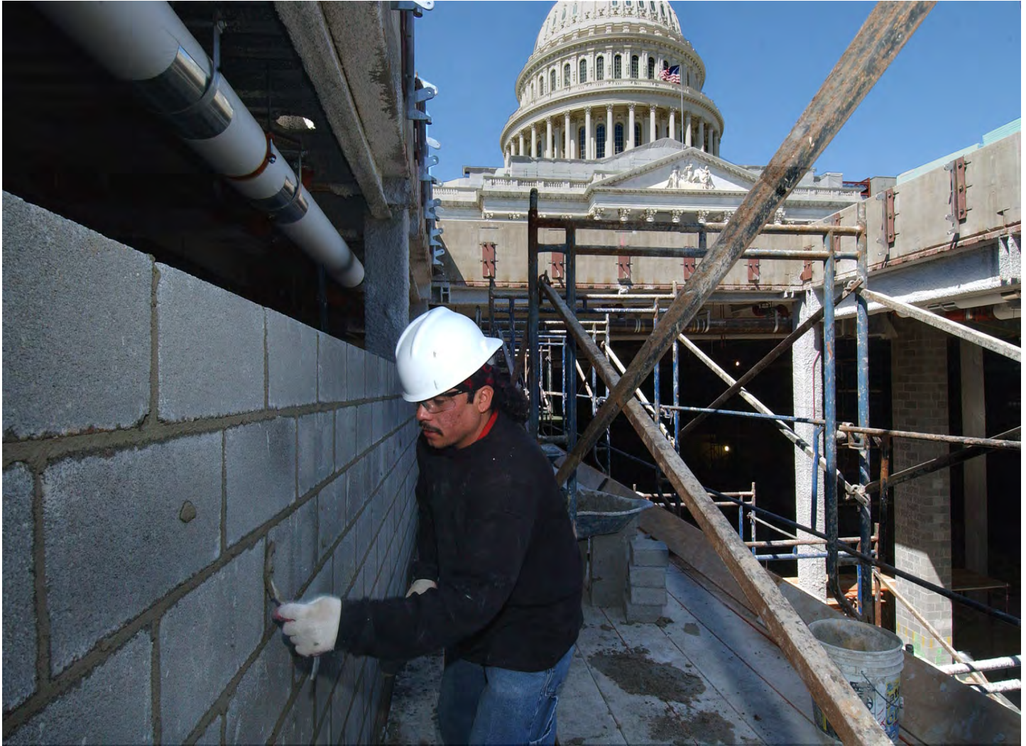
A CVC worker applies grout between masonry blocks at the south end of the Great Hall. An escalator bank will lie on the other side of the wall.
