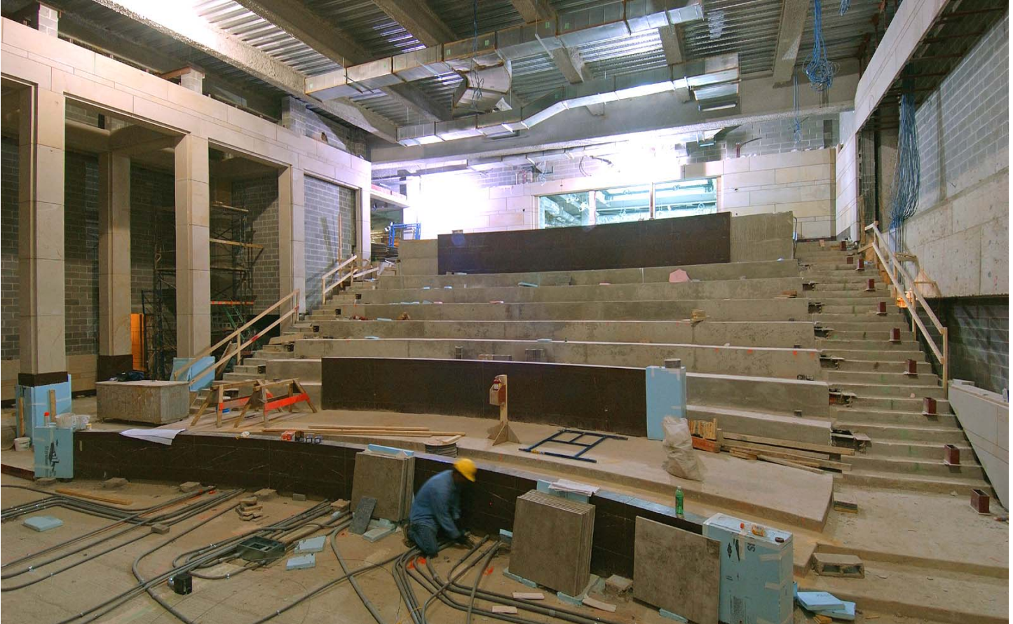
A worker lays electrical and communications conduit in the floor of the North Orientation Theater. The stone work is nearly complete inside the theater.
