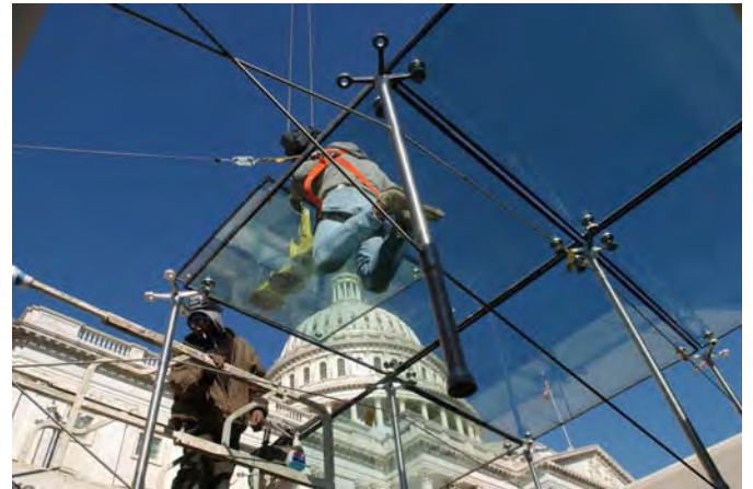
Workers have completed the installation of glass panes for the last of four skylights that lie along the East face of the Capitol.
