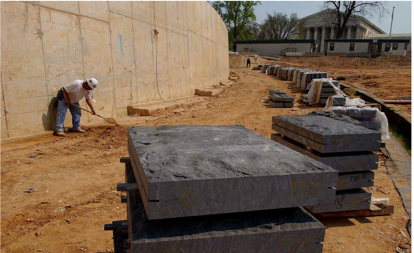
A worker prepares the ground at the base of the pedestrian ramp retaining wall on the north side of the CVC entrance zone. Stone masons are expected to begin installation of roughly cut granite blocks (center) to the wall later this week. The stones are intended to mimic the cut and color of the granite stones used by Frederick Law Olmsted in the late 1870s to build the low retaining walls along the perimeter of Capitol square.
