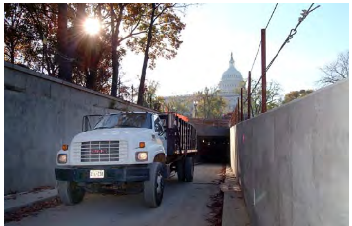
A truck exits the new truck service tunnel on the north side of Constitution Avenue. Between 50-60 trucks use the tunnel each week to deliver materials for the Sequence 2 contract (build-out and finishes).
