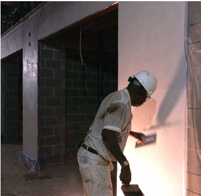
Plaster work continues to progress in the food services area and in the corridors near the Congressional Auditorium (above).
