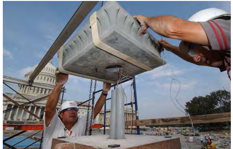
Stone masons guide a piece of stone into place for one of six historic lanterns in the center of the East Front Plaza near the CVC entrances.
