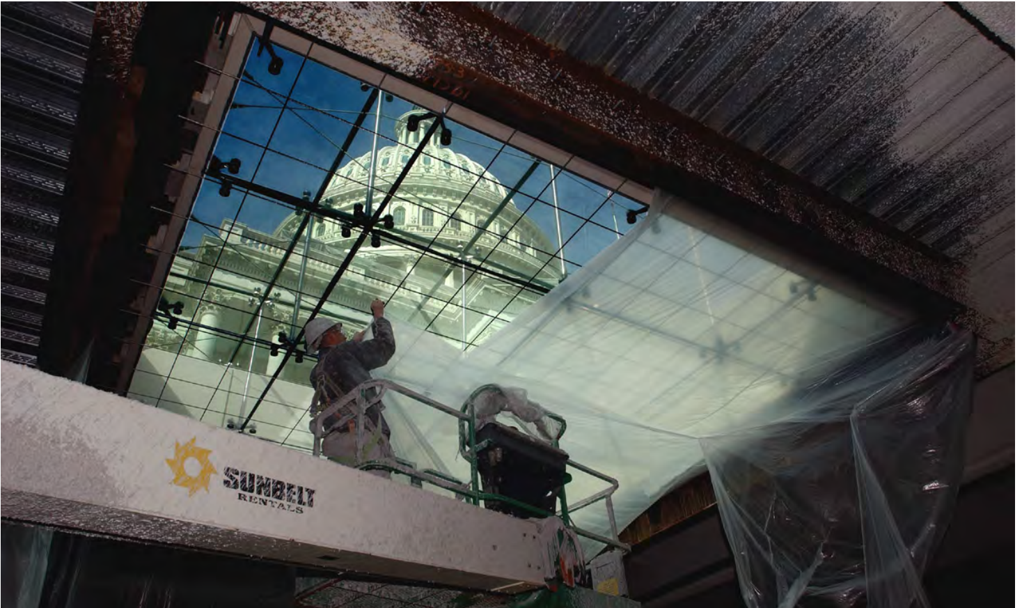
Workers secure a plastic tarp below a skylight to protect it from the fireproofing material that will be applied to the surrounding steel structure.
