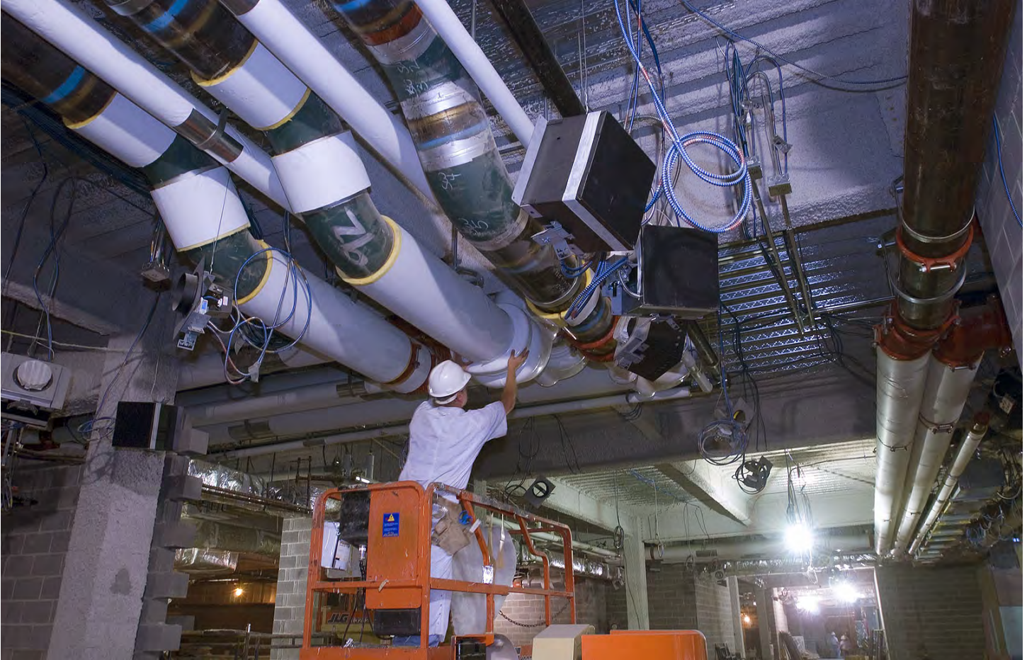
A worker installs insulation around a water pipe connection point in a corridor that lies between the Great Hall and House expansion space.
