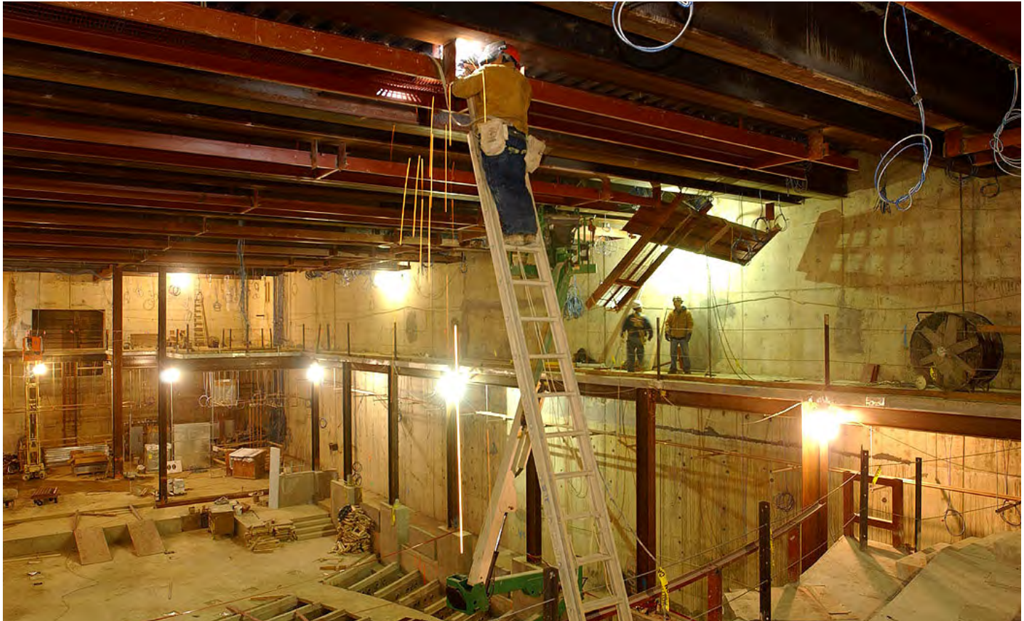
A worker welds a portion of a catwalk to a steel beam that supports the roof of the Congressional Auditorium.
