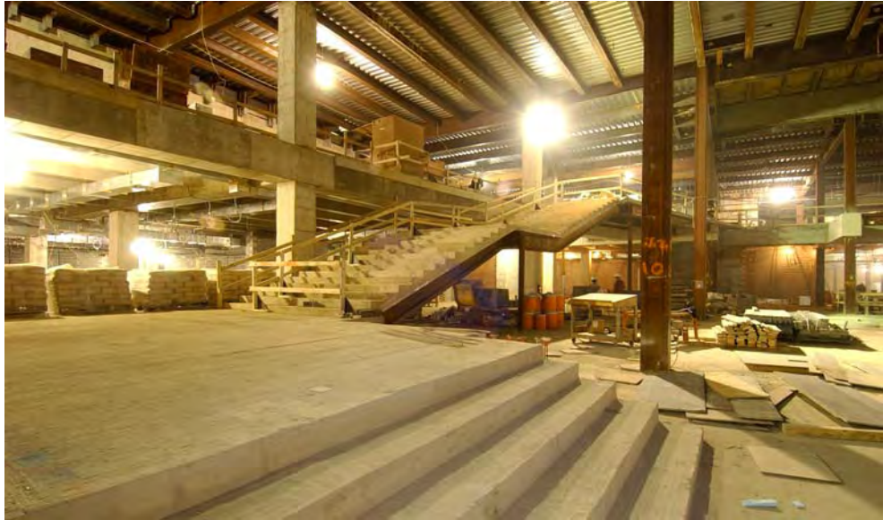
A view of the south staircase leading into the Great Hall. All major structural work is now complete.
