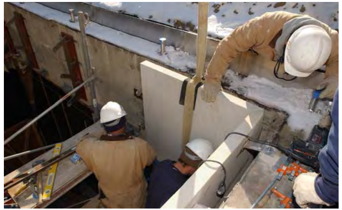
Workers secure sandstone to the walls of a skylight that is situated above a stairwell atrium located in the north end of the CVC.
