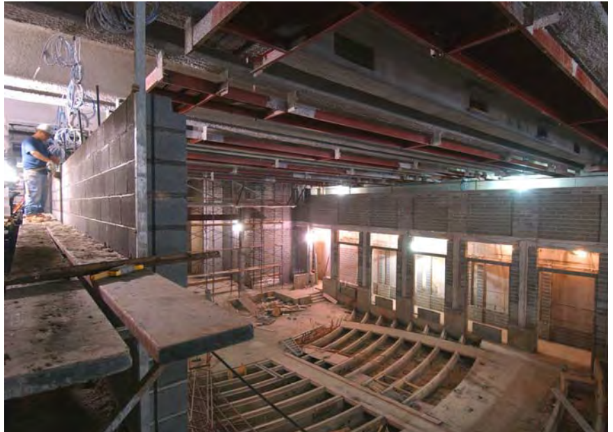
At left, a stone mason places a concrete masonry block to an upper wall inside the Congressional Auditorium. The facility will accommodate up to 450 people and will provide state-of-the-art audio/visual capabilities for presentations and briefings.
