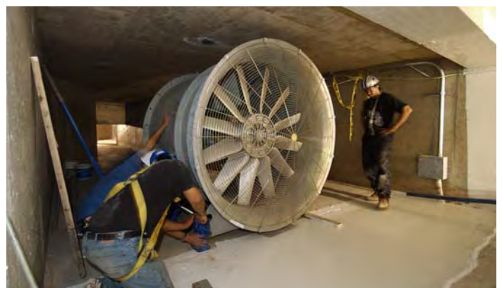
Workers secure a large fan unit to the floor of the CVC Service Level.
