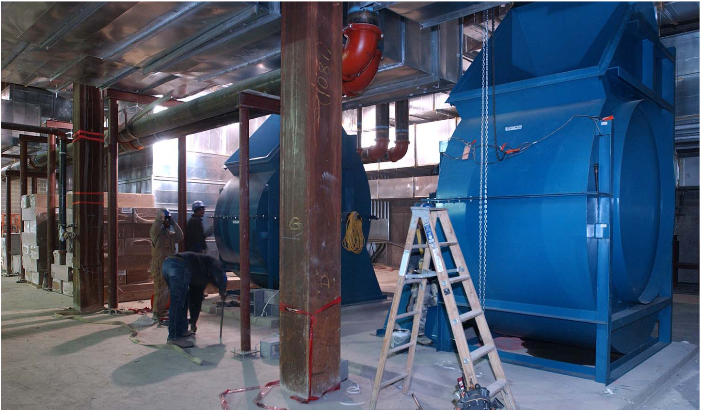
Large return fans, part of the CVC air handling system, are currently being installed in the service level.
