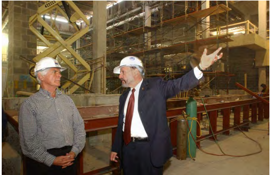
Architect of the Capitol Alan Hantman, right, discusses interior construction activities with House Appropriations Chairman Jerry Lewis (R-CA) during a CVC site walk on April 8, 2005.
