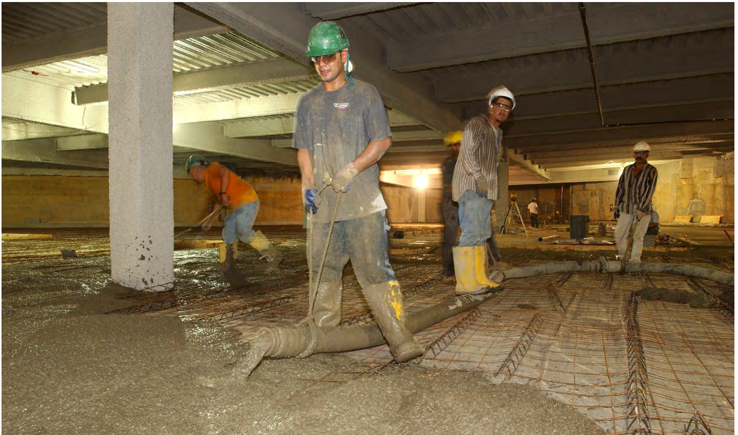
A construction crew places concrete for the floor topping slab on the upper level of the Senate expansion space.
