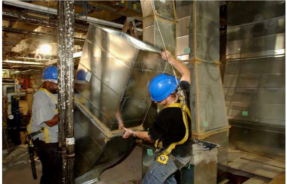
Workers maneuver a section of air duct into place in the CVC service level.
