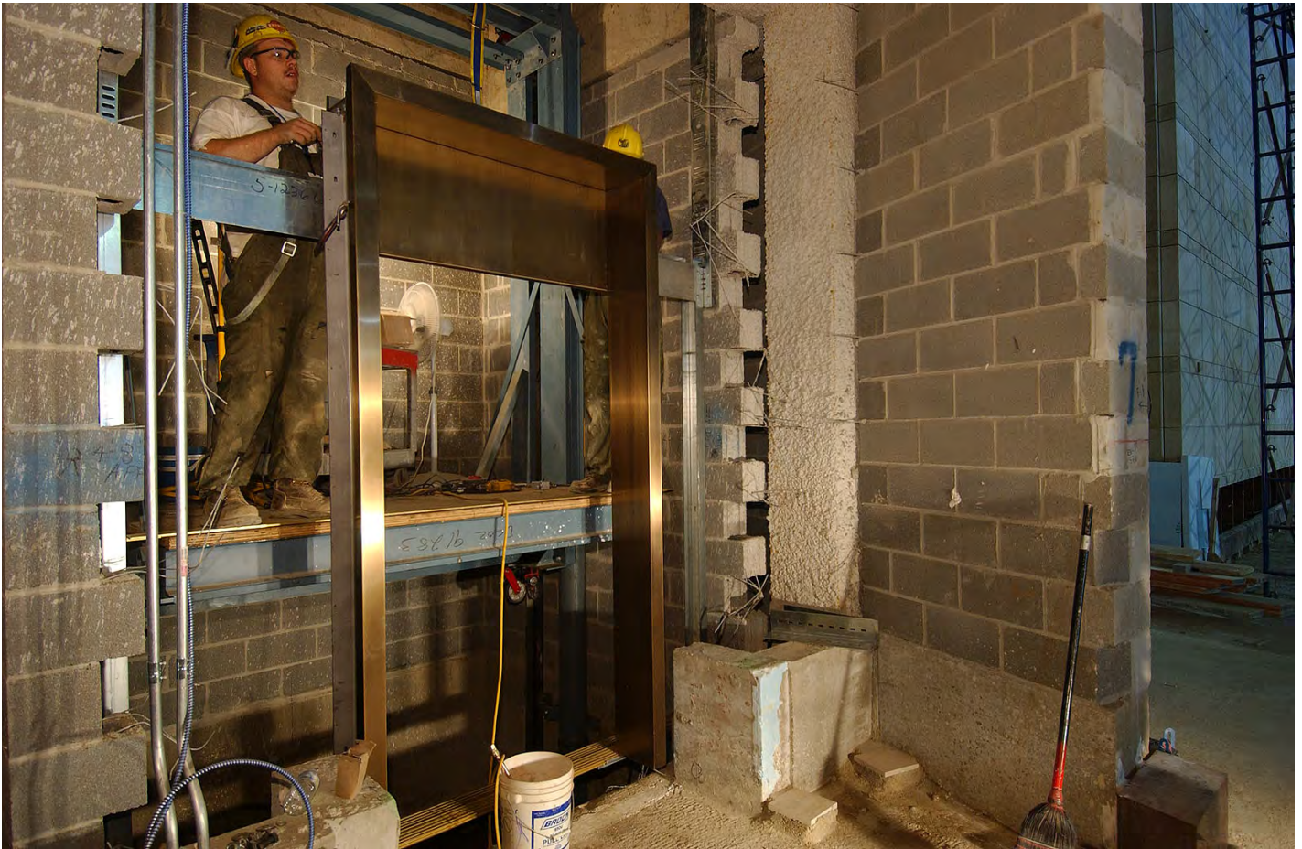
Near the Great Hall, a technician works on the installation of one of the CVC's 23 elevators. The facility also includes six escalators.
