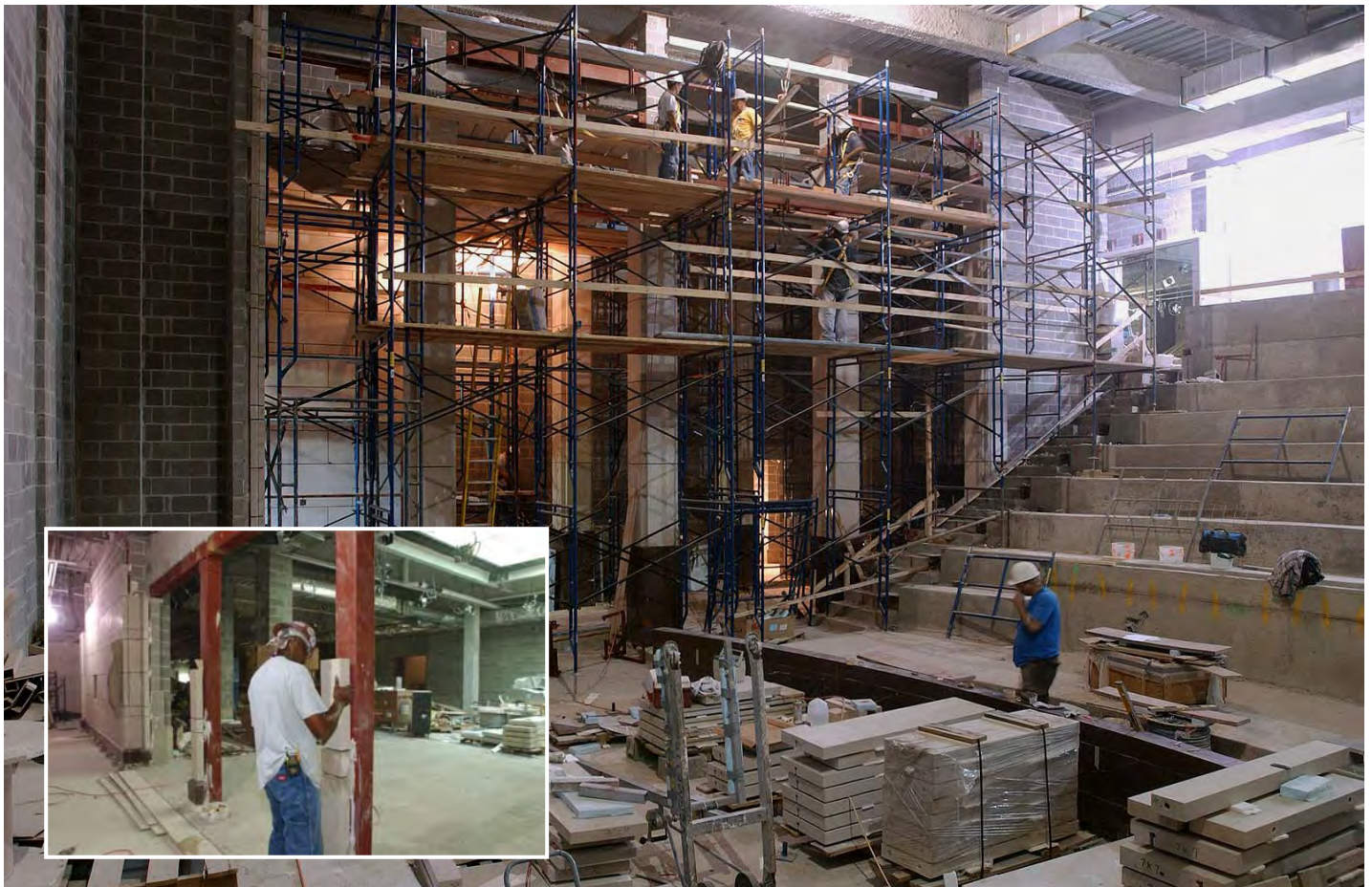
On a scaffold, a mason crew secures stone to the columns inside the north orientation theater as sunlight from an adjacent skylight illuminates the area. Inset: A mason sets a small sandstone block to the door framework at the upper level of the north orientation theater.
