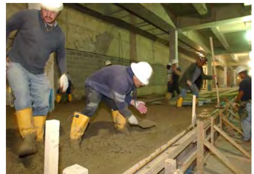
Workers level off a concrete slab after a recent concrete placement in the Exhibition Gallery.
