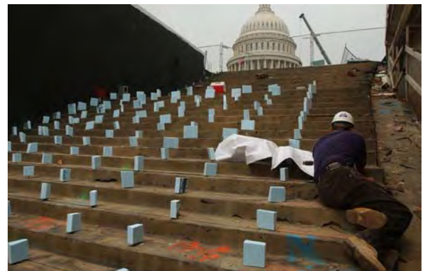
A worker sets dowels in the steps near the north entrance to the CVC. The dowels will help support and anchor the granite blocks that will be positioned on the steps.
