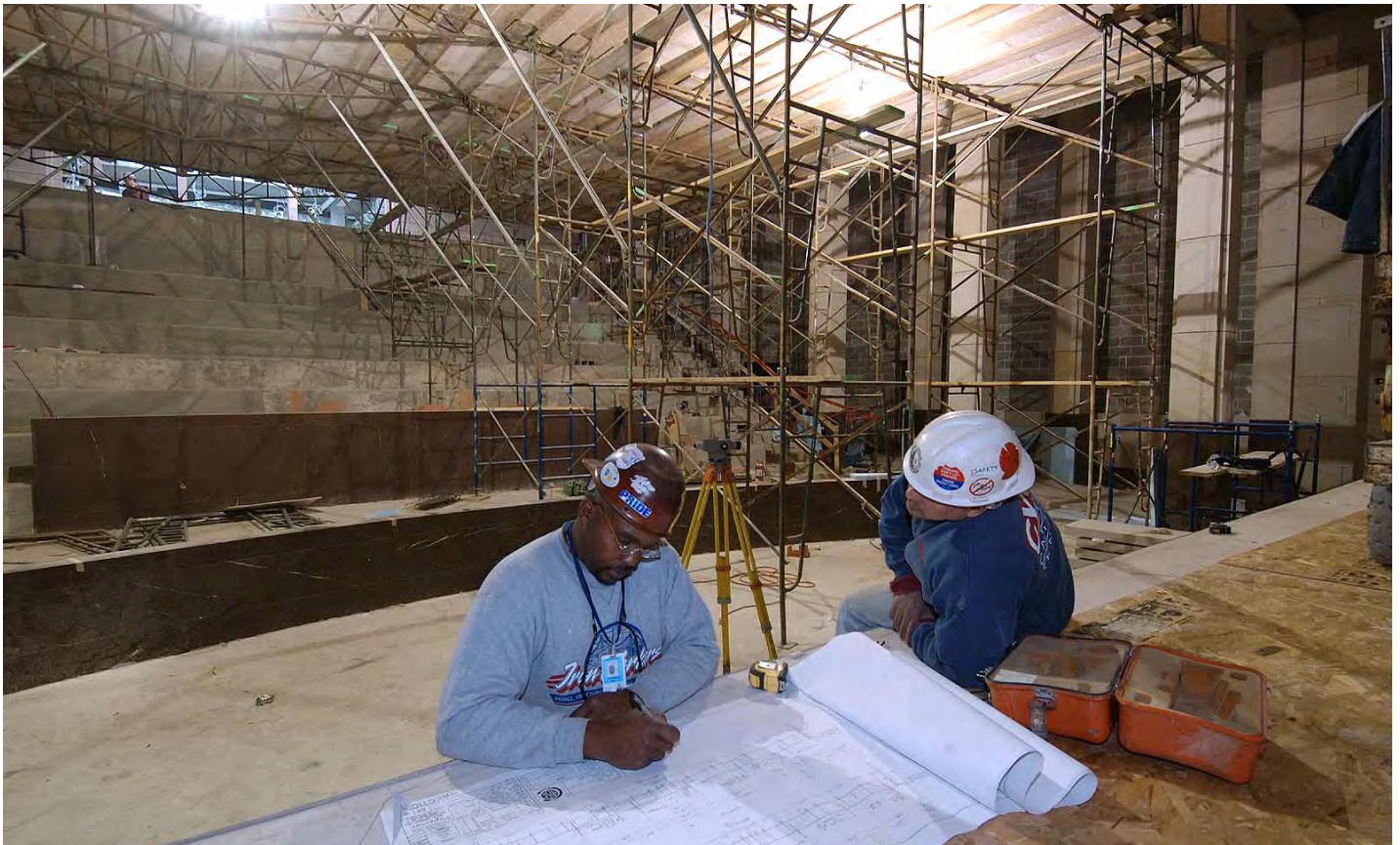
Workers review mechanical drawings in the south Orientation Theater. The scaffolding in the background provides a platform for ceiling work.
