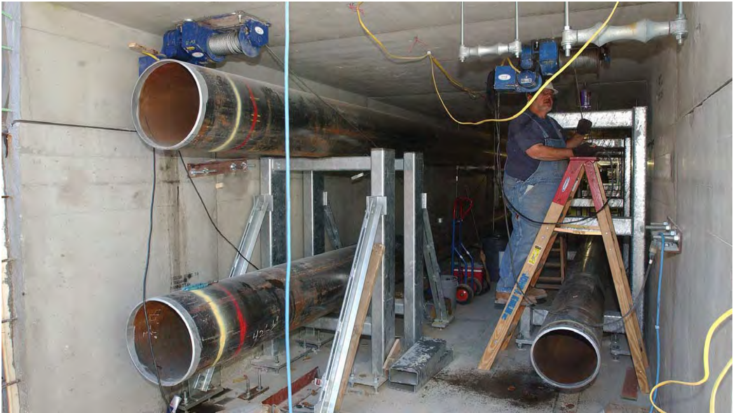
Pipes are in place inside much of the pre-cast concrete sections of the CVC utility tunnel below East Capitol Street.
