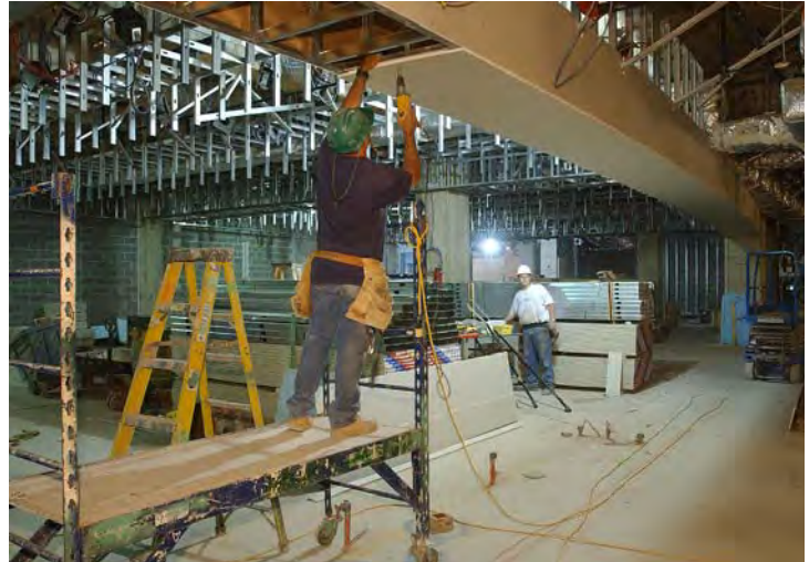
A worker installs sheetrock to a portion of the ceiling in the food service area on the lower level of the CVC. When completed, the dining space will be able to accommodate approximately 550 people.
