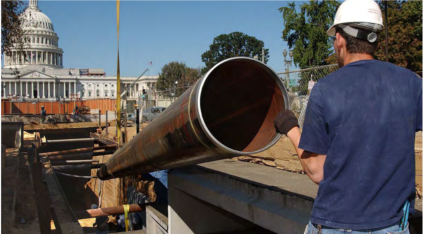
A worker helps guide a 40-foot steel pipe into place inside the CVC utility tunnel. Work on the tunnel will continue through the winter.
