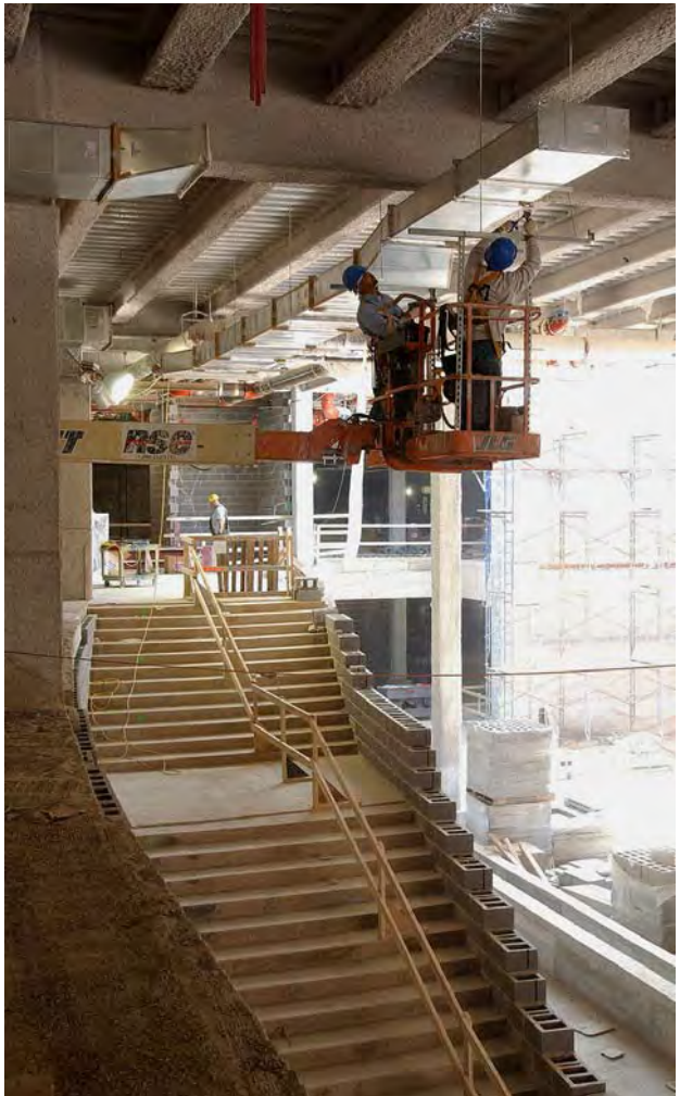
Sequence 2 workers install ductwork to the ceiling above a staircase at the eastern end of the Great Hall. At right, Sunlight pours in through the Great Hall's south skylight.
