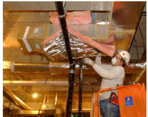
A worker installs thermal insulation around ductwork in the lower level of the CVC.
