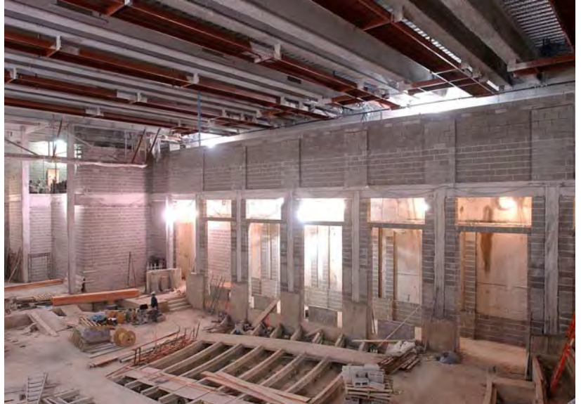
Blockwork continues to rise along the south wall of the Congressional Auditorium.
