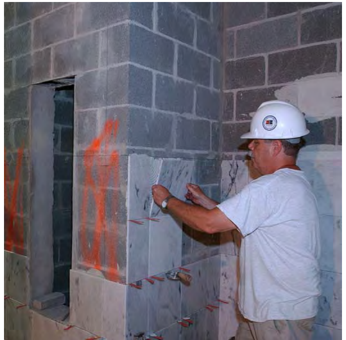
A worker sets marble tile to a wall inside a CVC restroom. Each of the CVC restrooms will be accessible for persons with disabilities.
