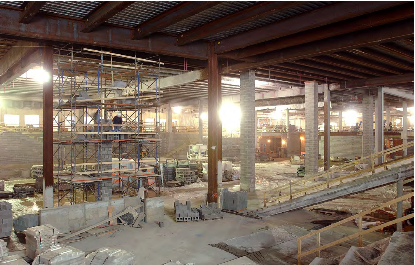
On a scaffold at left, masonry workers build a masonry block column adjacent to one of the steel columns inside the Great Hall of the CVC.
