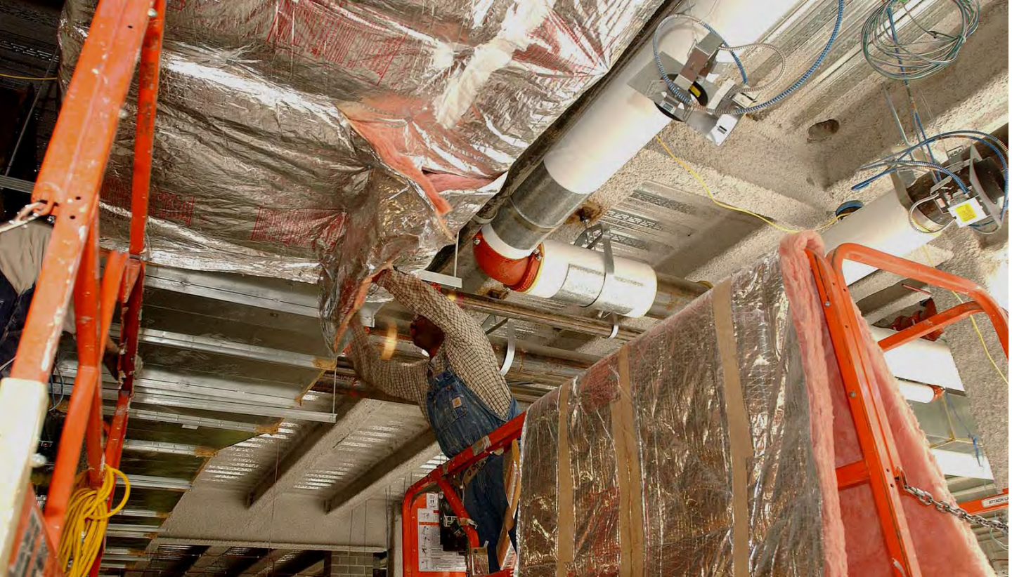
A worker wraps CVC air duct with insulation. In all, 20 large and sophisticated air handling units will control air flow throughout the CVC.
