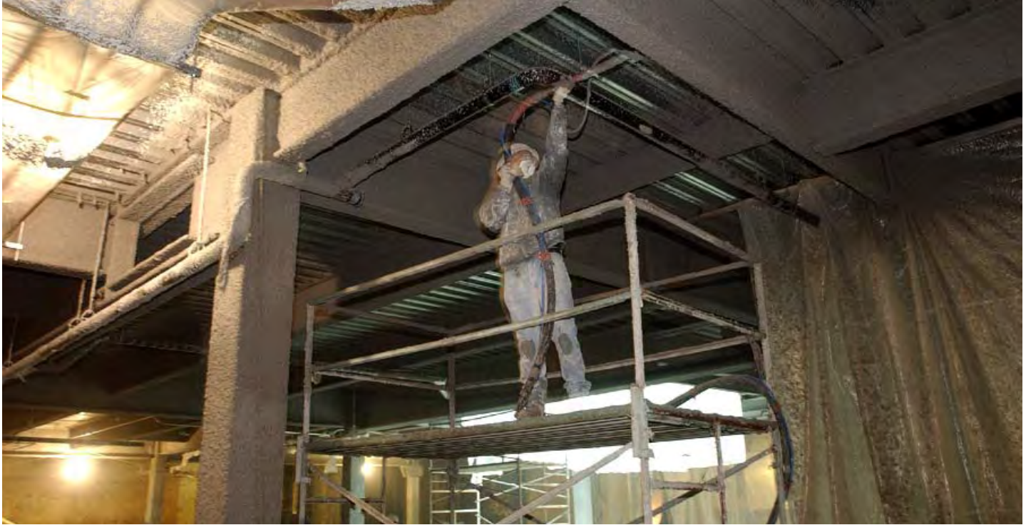
A worker applies a fireproofing material to the steel structural elements on the upper level of the CVC.
