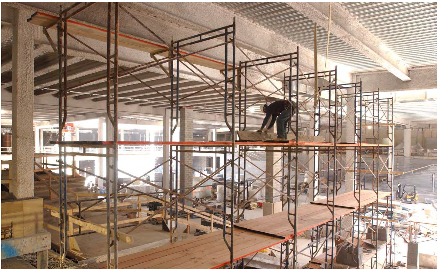
A worker prepares a scaffold for utility installation work that will occur along the ceiling within one of the CVC's two orientation theaters.
