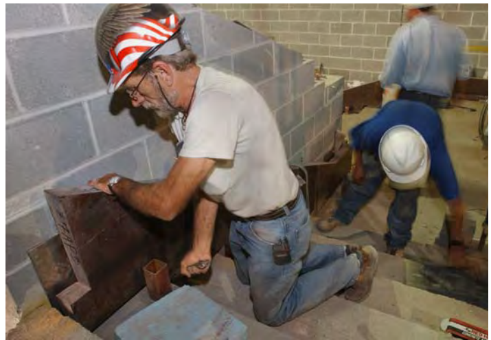
Stone masons set Tennessee Valley marble along the base of a stairwell near the south Orientation Theater.
