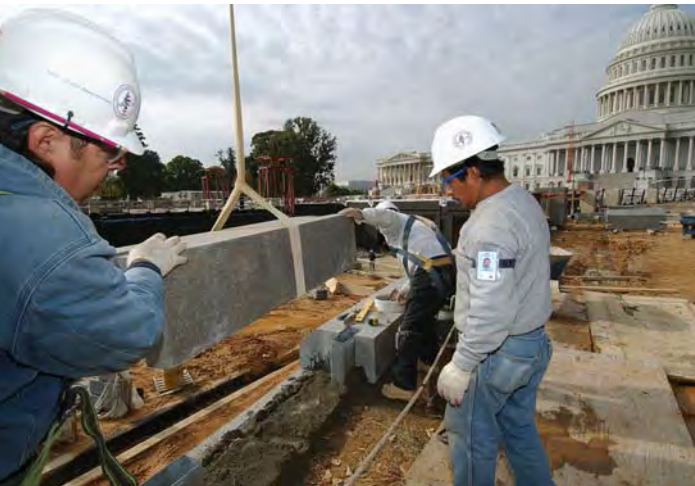
Stone masons set a cap stone atop a retaining wall in the northeast quadrant of the CVC site. A bronze railing will be installed later.
