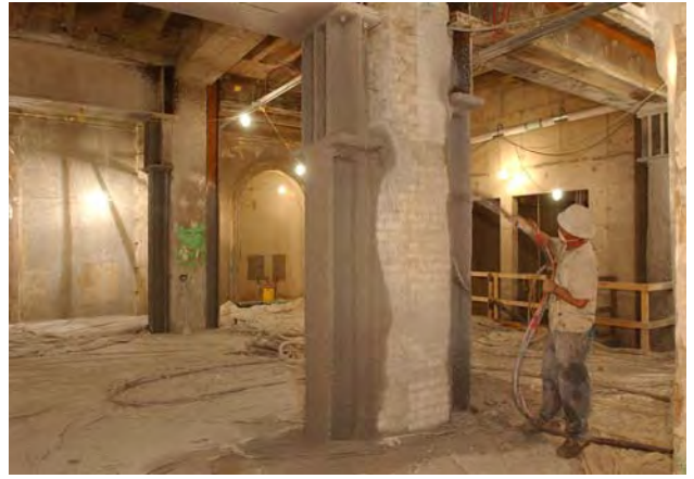
A Sequence 2 worker applies a fireproofing material to a steel column inside the East Front Extension.
