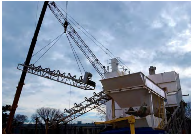
A crane continues to disassemble the concrete mixing plant on the south side of the CVC site. The on-site plant ensured the efficient delivery of concrete throughout the project area and kept approximately 30 cement trucks off the roads each day.
