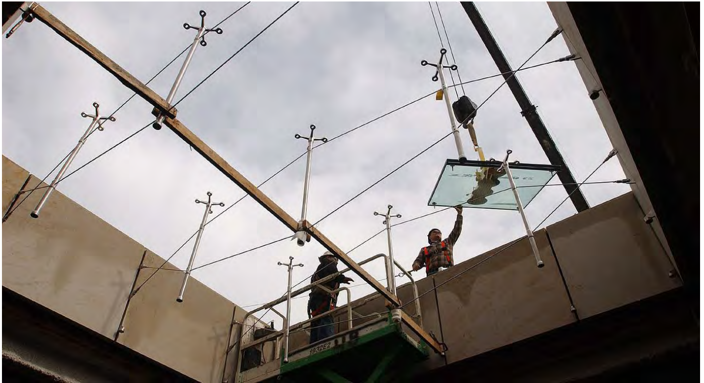
A glass installation crew guides a pane of glass into position for a skylight situated above a stairwell that leads to Senate expansion space.
