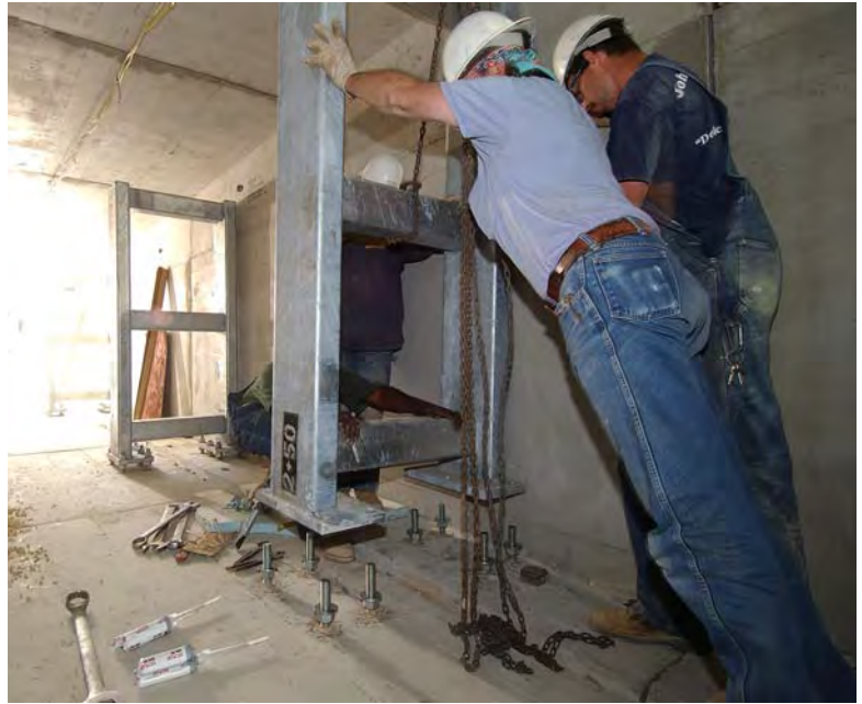
Workers position a steel pipe support inside a new utility tunnel for the CVC. The tunnel will accommodate new chilled water and steam lines.
