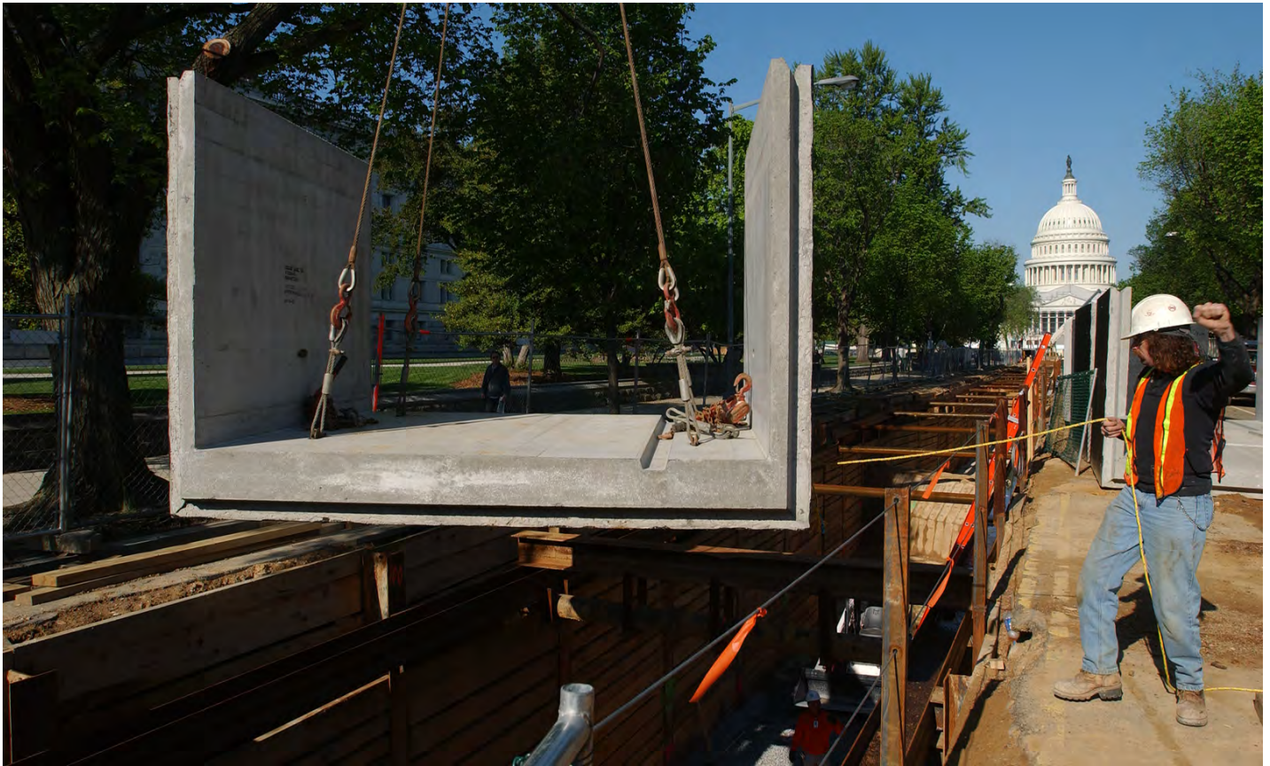
A worker guides a section of a pre-cast concrete tunnel into the trench for the CVC utility tunnel along East Capitol Street.
