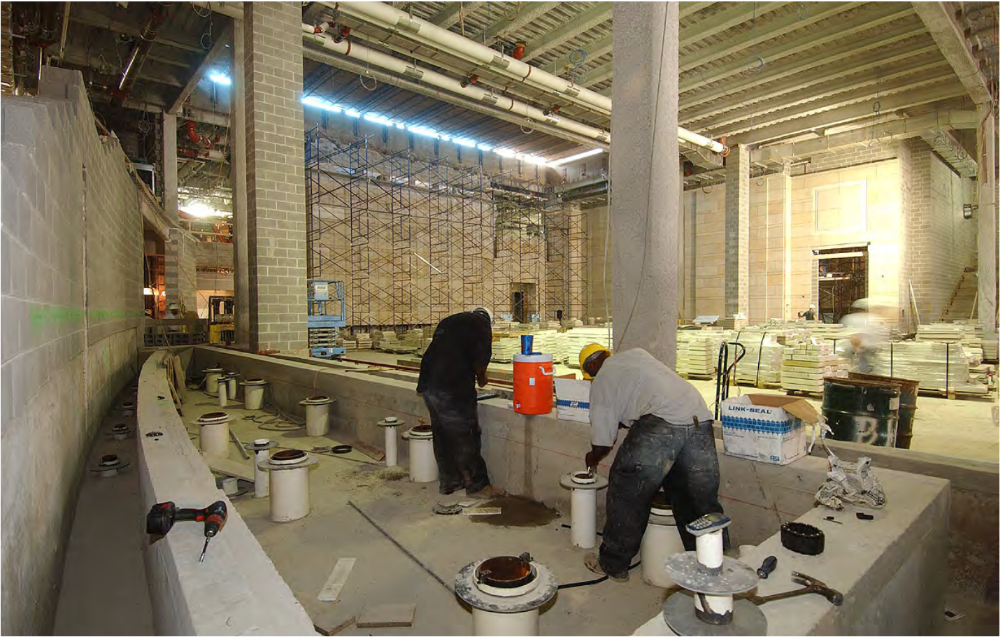
Workers prepare plumbing fixtures and conduit for a water feature near the stairs along the southeast corner of the Great Hall.
