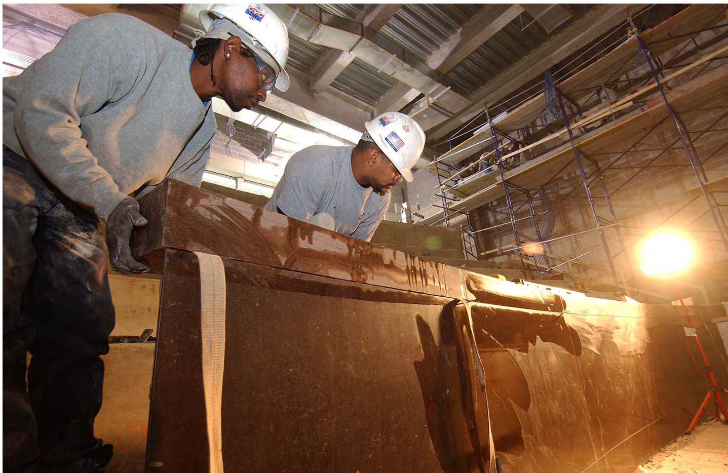
Stone masons position a piece of Tennessee marble into place on one of the two “modesty” walls in the south Orientation Theater.
