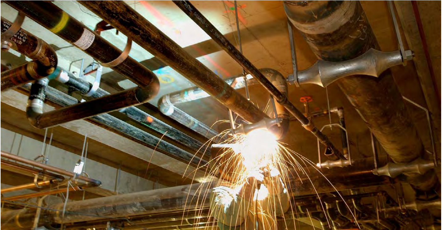
A worker welds the joint of a utility line in the CVC service level. Work on the primary CVC utility tunnel begins this Saturday, Jan. 22.
