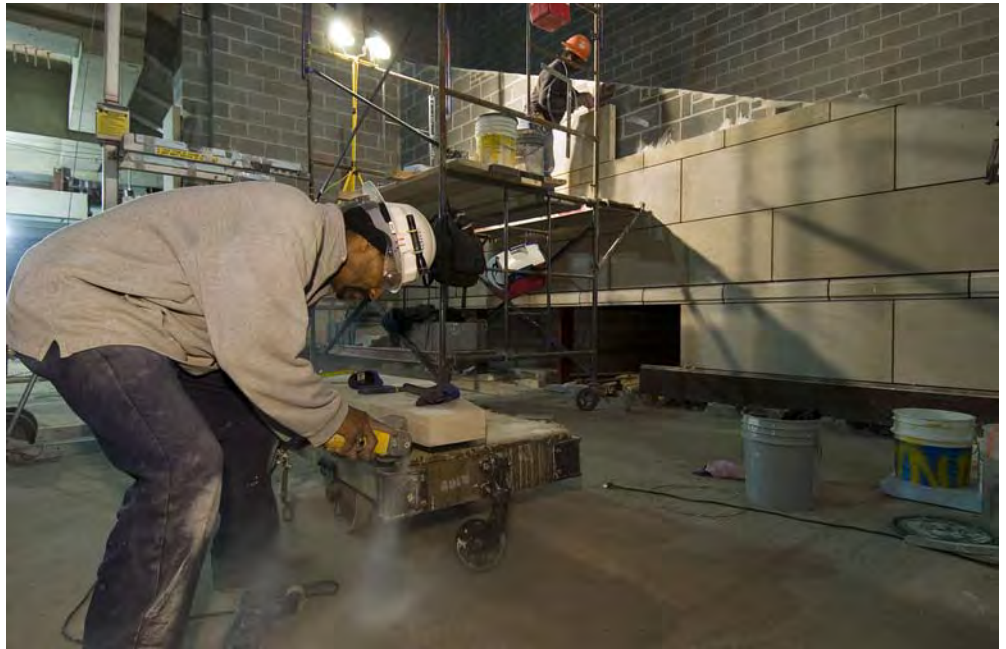
A stone mason trims a sandstone block to be set on a stairwell wall on the west side of the Great Hall.
