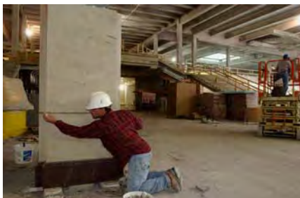
In the Great Hall, a stone mason applies grout between two sandstone blocks.
