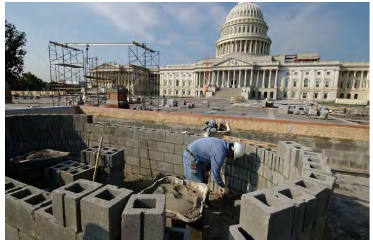
A worker applies mortar between the concrete masonry blocks that will support the elliptical granite tiers of the historic Olmsted fountain.
