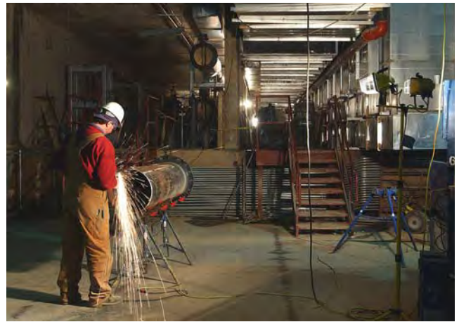
A worker grinds down a steel pipe in the CVC service level.
