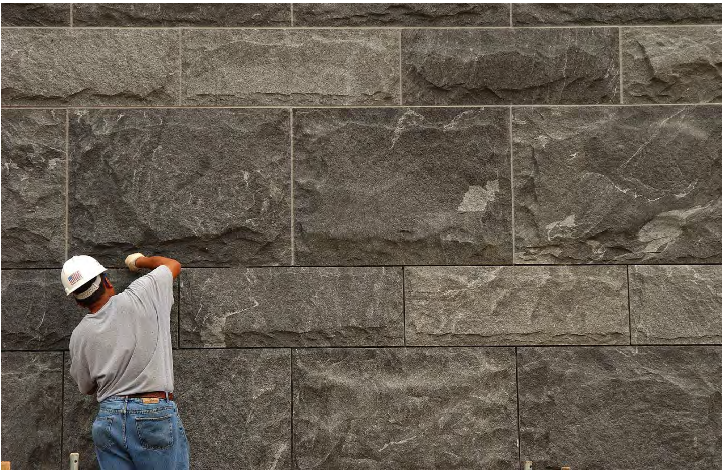
A stone mason applies grout between granite blocks on the retaining wall along the north pedestrian ramp that leads to the CVC entrance.
