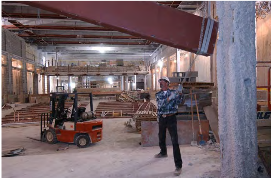
A worker helps guide a steel beam into place inside the Congressional Auditorium.
