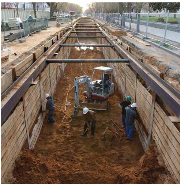
Along East Capitol Street, excavation work continues in a utility trench that, eventually, will reach a depth of 20 feet.
