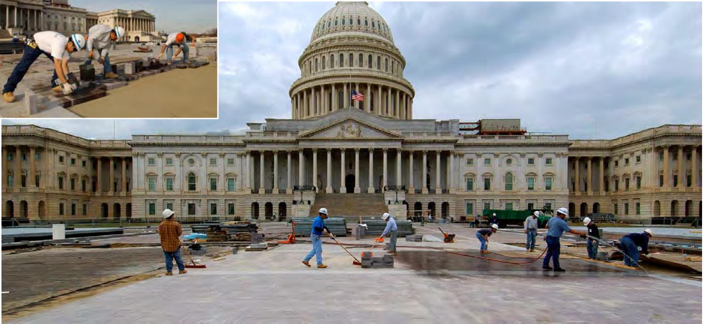
CVC crews continue preparing the East Front Plaza for the Inauguration next week. Inset: Stone masons install pavers in the middle of the Plaza.
