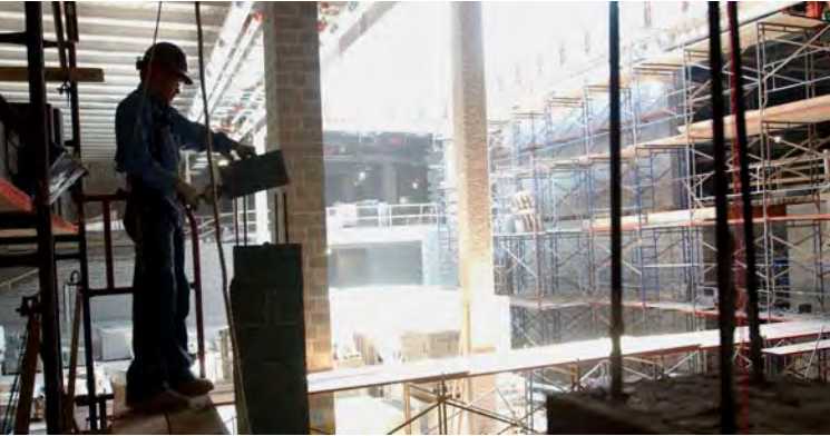
A Sequence 2 worker installs a concrete masonry block to a column inside one of the CVC’s two orientation theaters.
