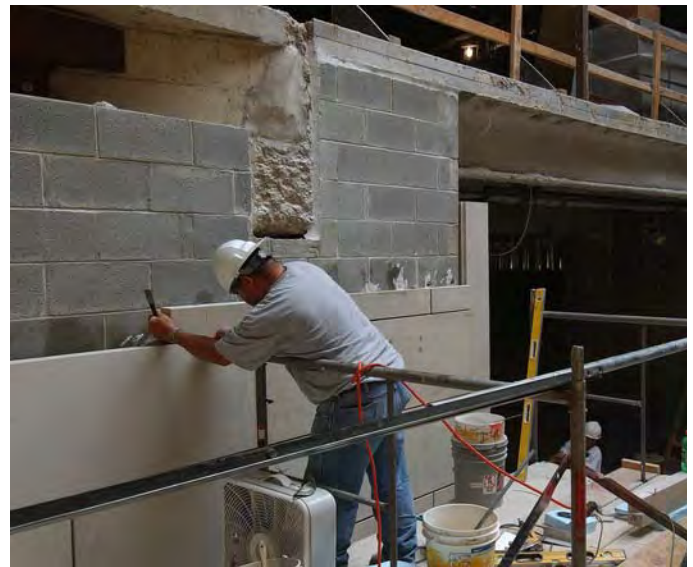
A stone mason sets a block of sandstone to the east wall of the CVC's Great Hall. Nearly 75 percent of the stone is in place inside the Hall.
