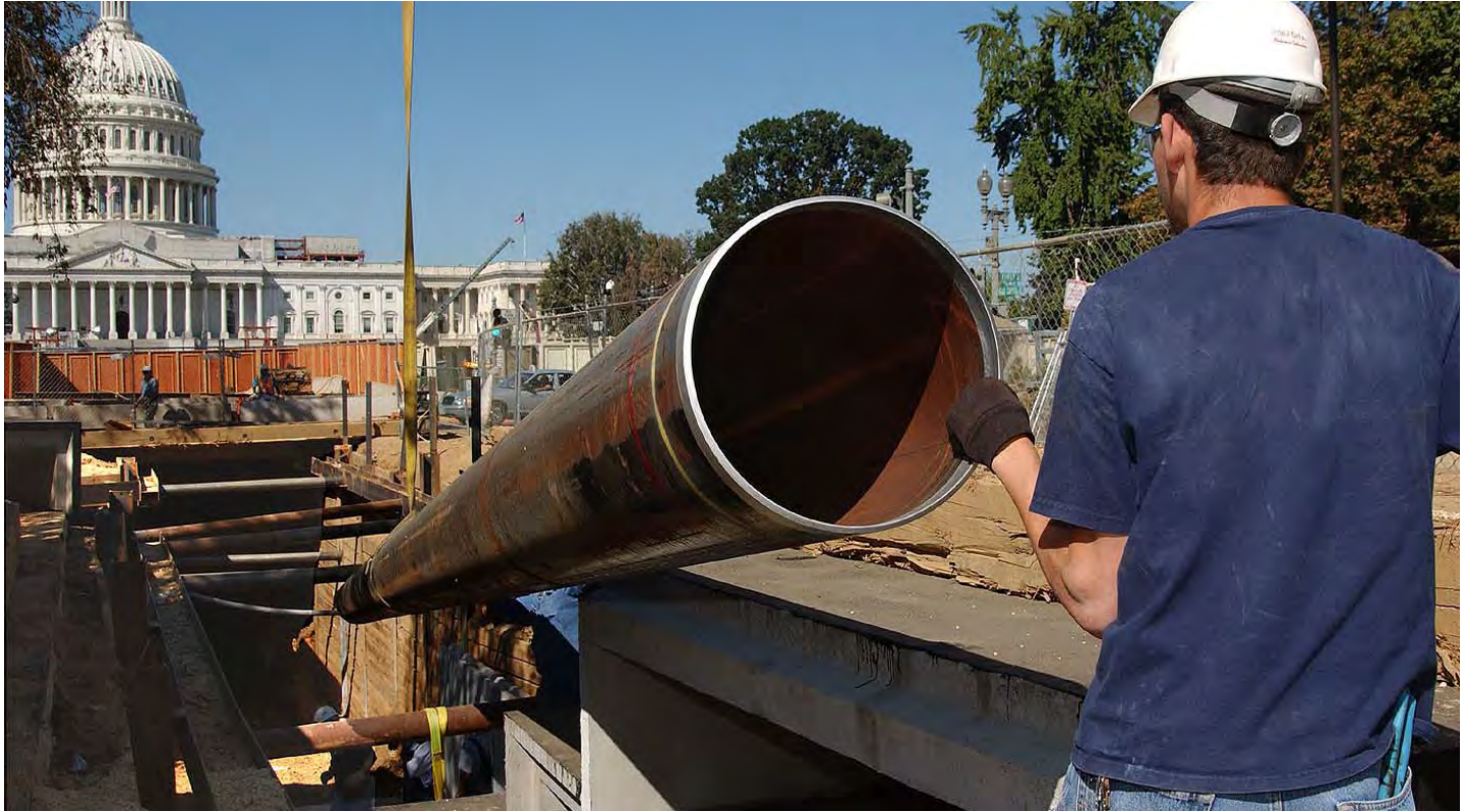
A worker helps guide a 40-foot steel pipe into place inside the CVC utility tunnel. Work on the tunnel will continue through the winter.
