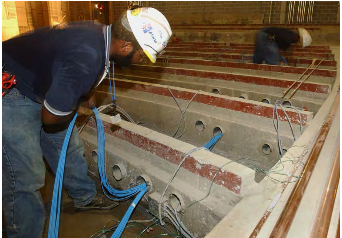
Workers inside the Congressional Auditorium pull telecommunications wires through openings that lie below the seating area within the facility. When completed, the Auditorium will feature state-of-the-art audio/visual technology and can serve as an alternate House or Senate Chamber if needed.
