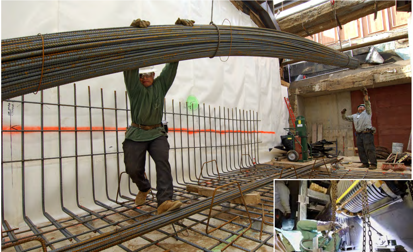
Workers lower a bundle of steel rebar inside the utility tunnel below East Capitol Street at the intersection with First Street. Inset: A worker welds together a utility line connection.
