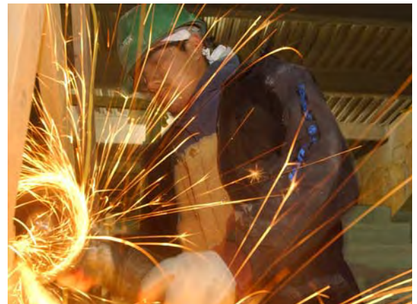
Sparks fly as a worker cuts through a steel plate in a stairwell wall on the north side of the CVC.
