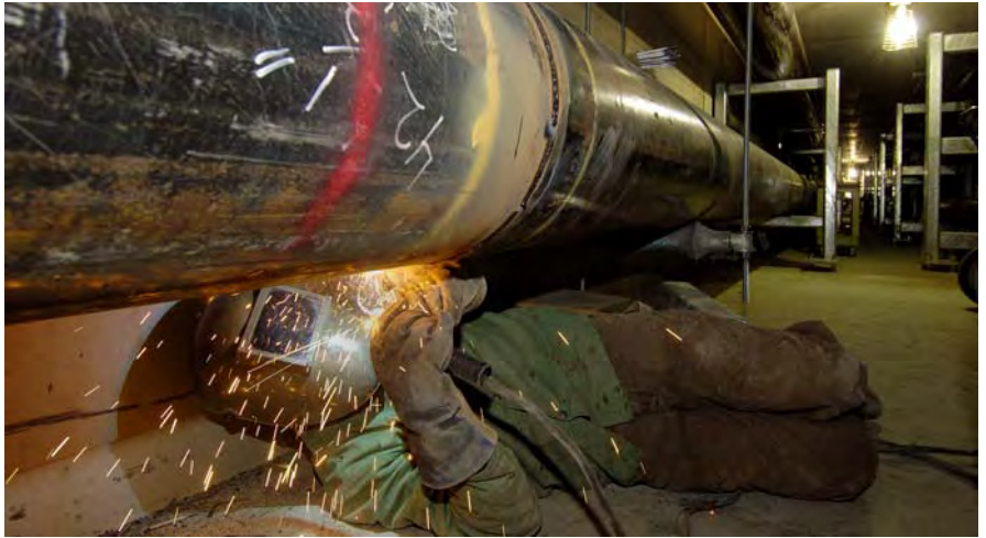
A worker in the CVC utility tunnel welds together two 40-foot-long steel water pipes.
