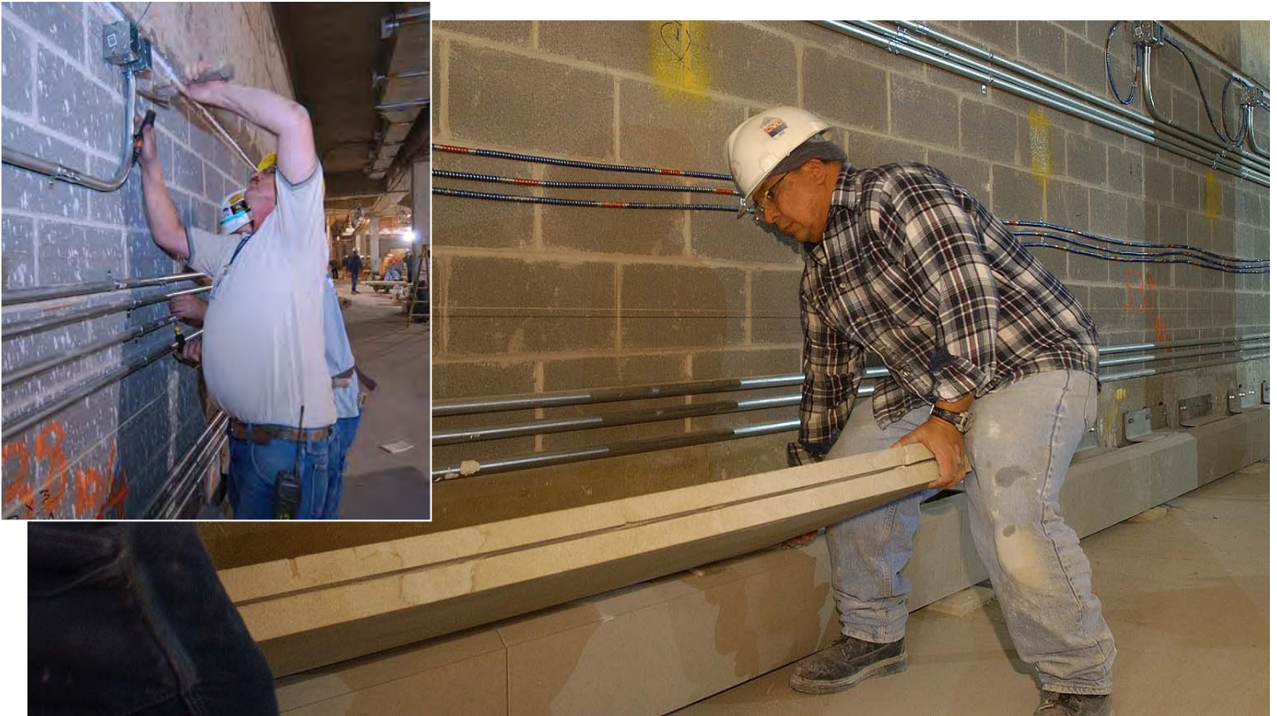
A stone mason sets a block of western Pennsylvania sandstone to a wall inside the Exhibition Gallery. Inset: Workers install electrical and telecommunications conduit for some of the 24 interactive computer stations that will be situated inside the Gallery.
