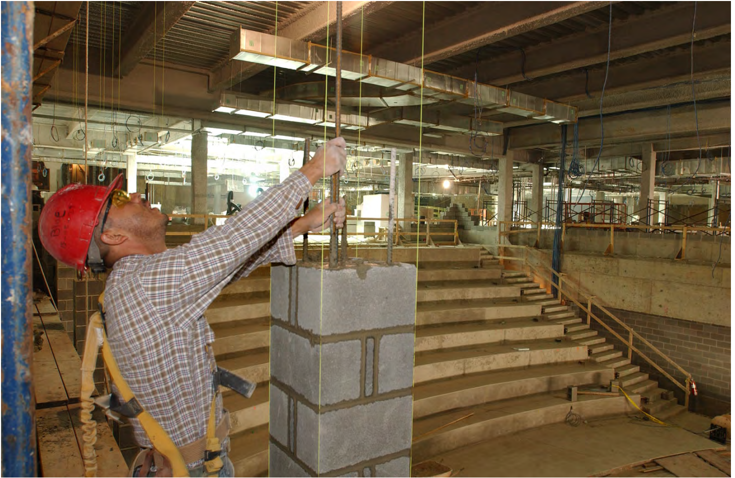
Inside one of the CVC's two orientation theaters, a worker aligns a steel support rod inside the blockwork of an interior column.
