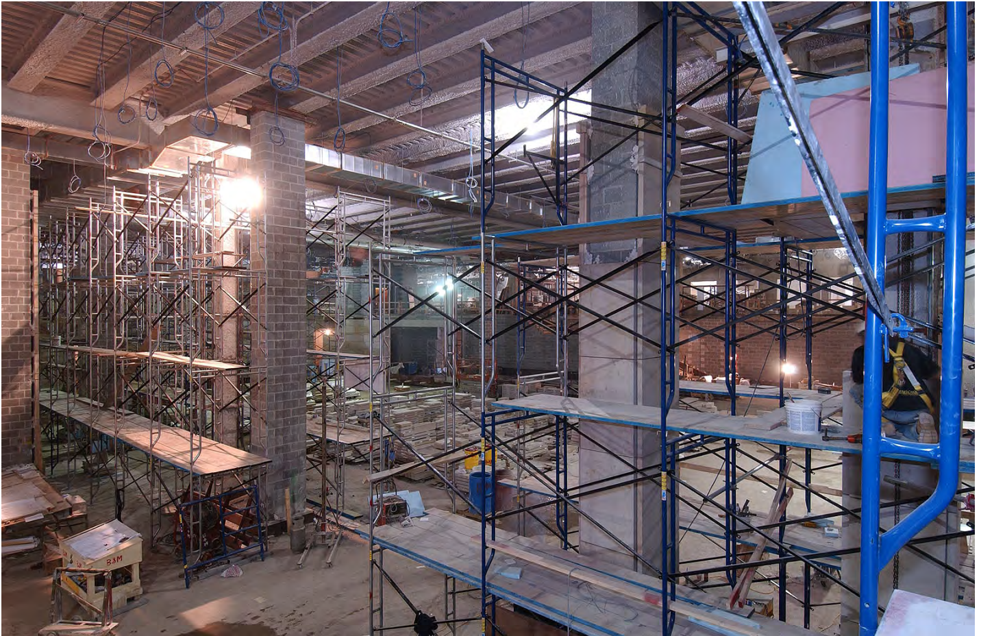
A stone mason (far right) sets stone to a column inside the Great Hall. Scaffolding will soon rise throughout the Hall to allow ceiling work to begin.
