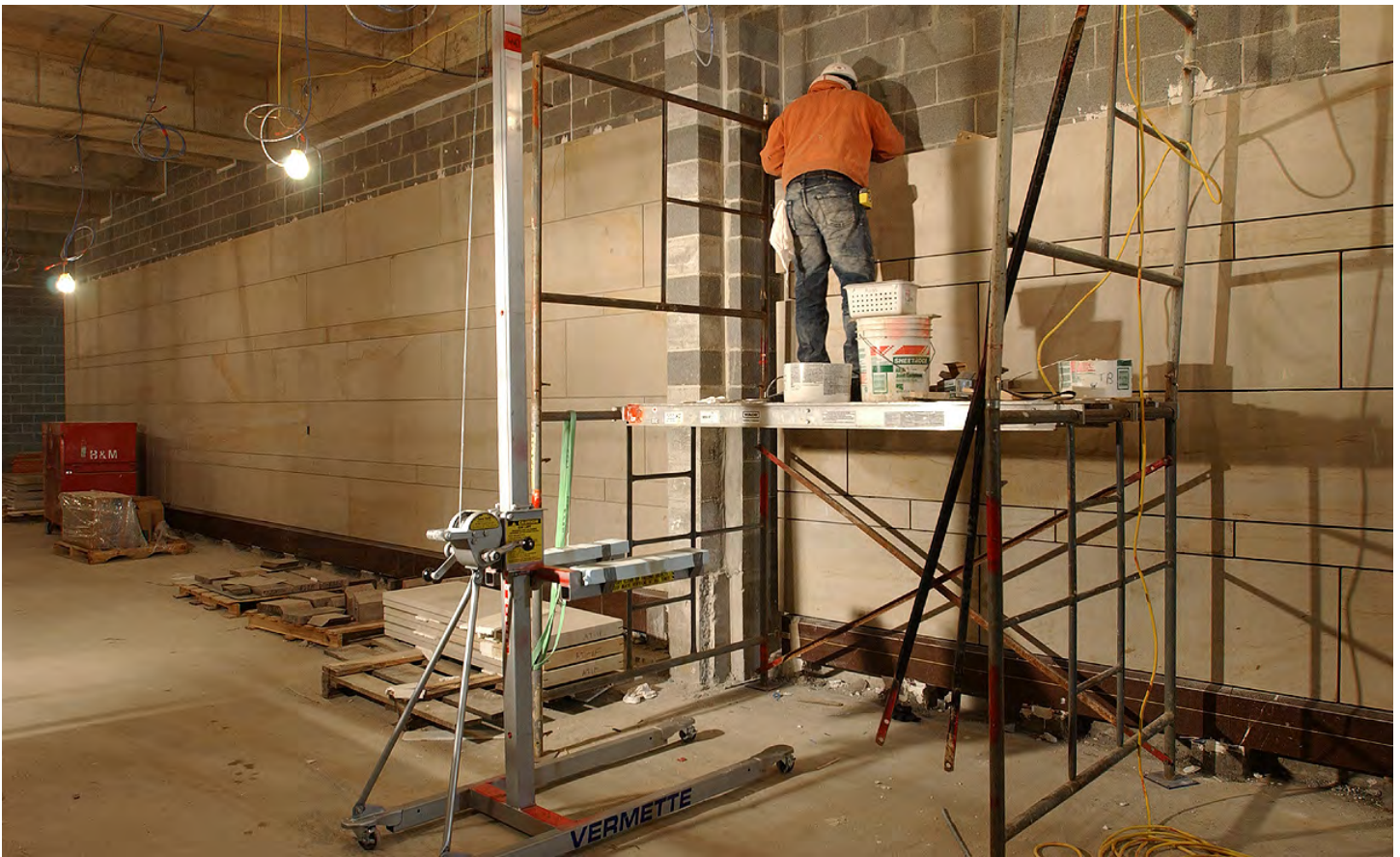
A stone mason installs sandstone blocks along one of the corridor walls near the CVC food service area on the lower level.
