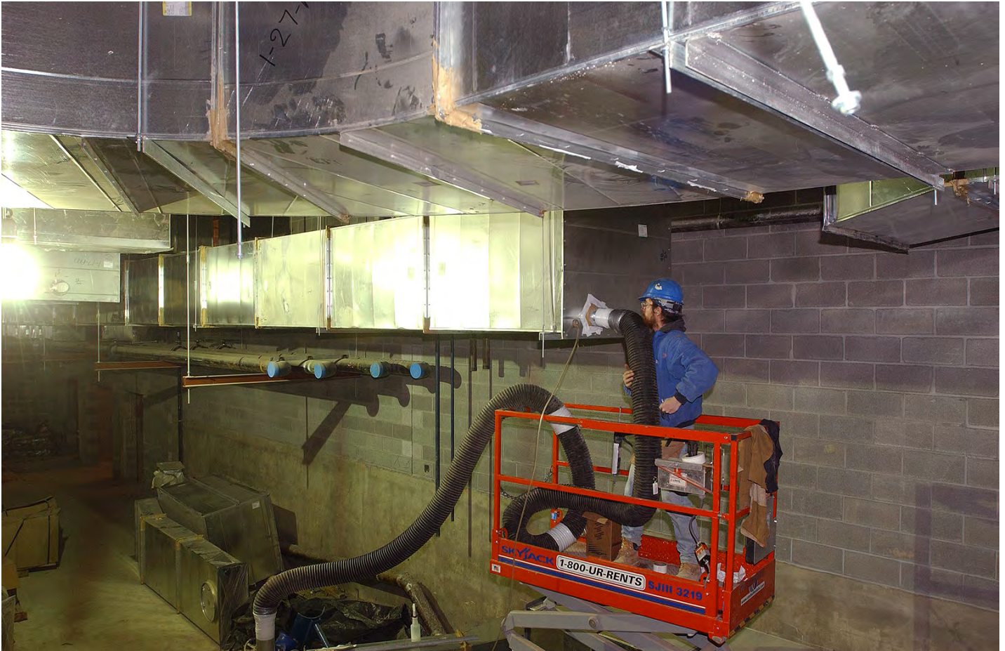
In the lower level of the CVC a worker pumps air at high pressure into a portion of ductwork to test the seals that connect the ductwork sections.
