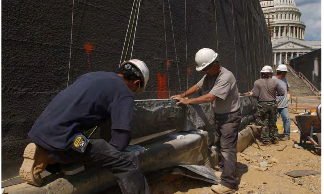
Stone masons set a granite block from a quarry in Culpeper, VA., to the south-side retaining wall within the CVC entrance zone. The “split-face” cut of the granite is intended to mimic the Capitol’s historic perimeter retaining walls designed by Frederick Law Olmsted in 1874.
