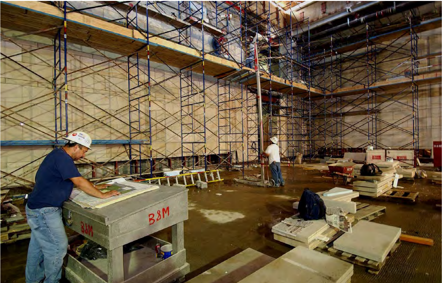
Sandstone rises nearly 30 feet along the south walls of the Great Hall. An information desk will be situated in front of the wall at left.
