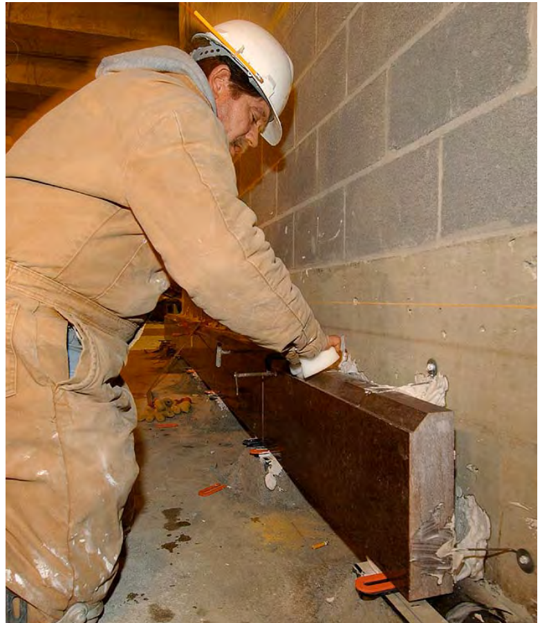
In the lower level of the CVC, a stone mason installs a marble base stone, the first finish stone to appear inside the CVC.
