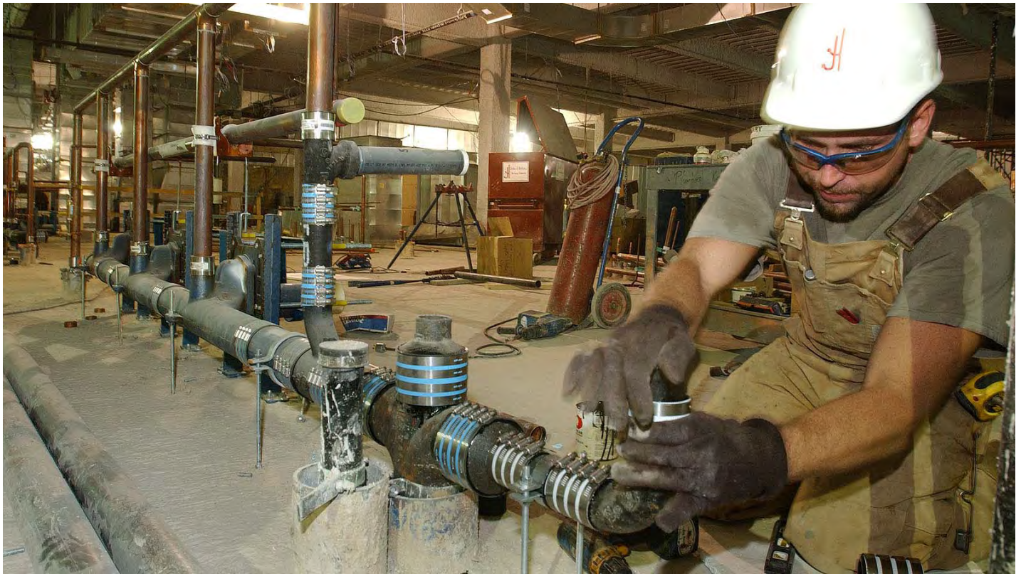
A pipefitter assembles a portion of the plumbing configuration in one of the CVC's 26 restrooms, which include 10 family restrooms.
