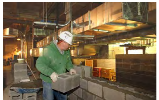
In the lower level of the CVC, a worker sets one of the 750,000 masonry blocks that will help define the interiors spaces within the CVC.
