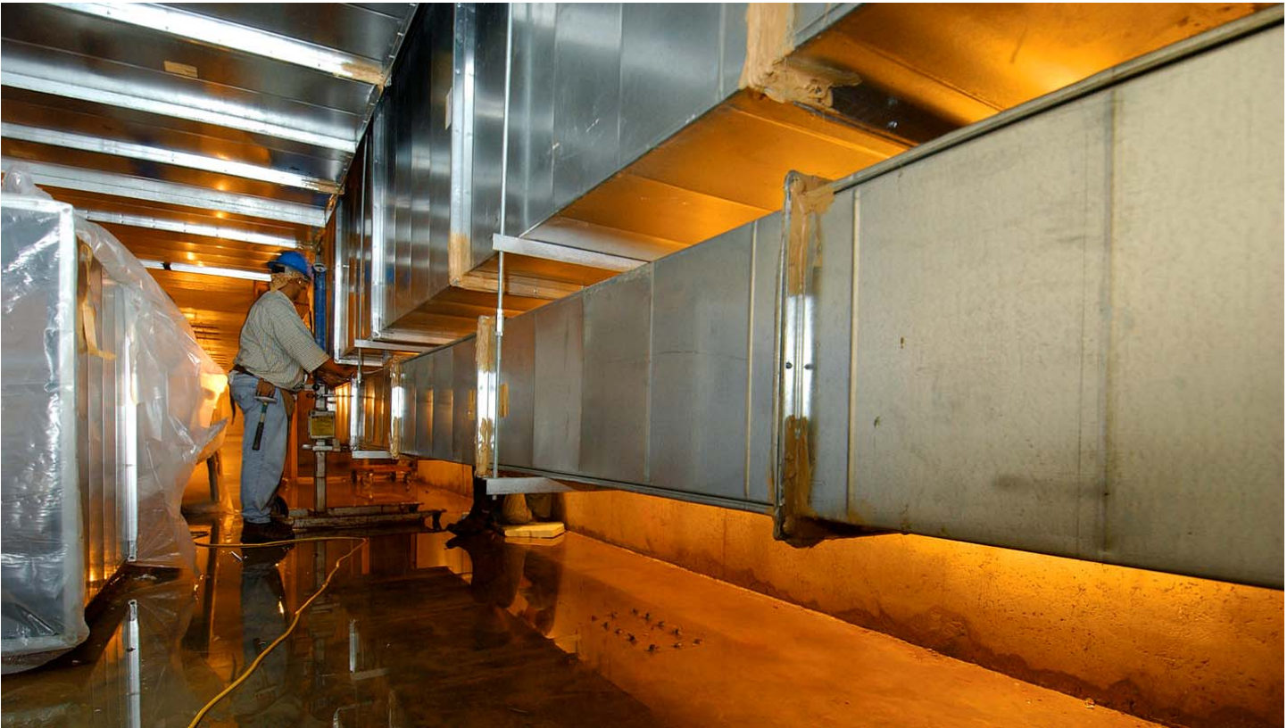
A worker installs air handling ductwork in the CVC service level. Utility installation will continue through the end of 2004.
