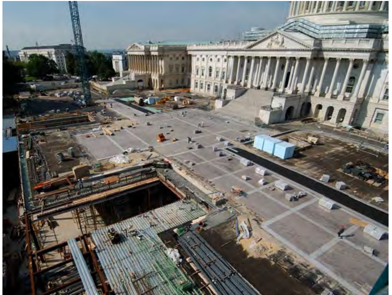
During the recess, stone crews laid approximately 30,000 granite pavers, which are now visible throughout the western half of the CVC roof deck.
