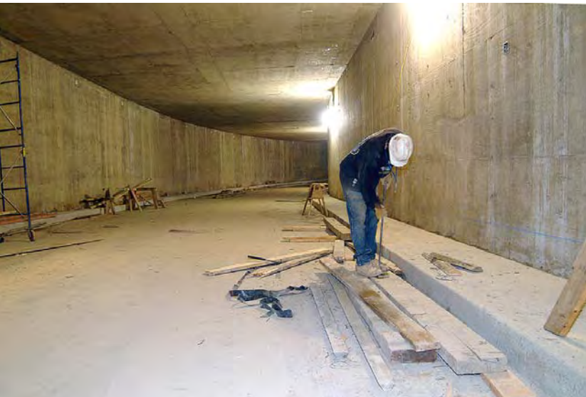
Most of the concrete has been placed for the roof slab and walls of the CVC truck tunnel.
