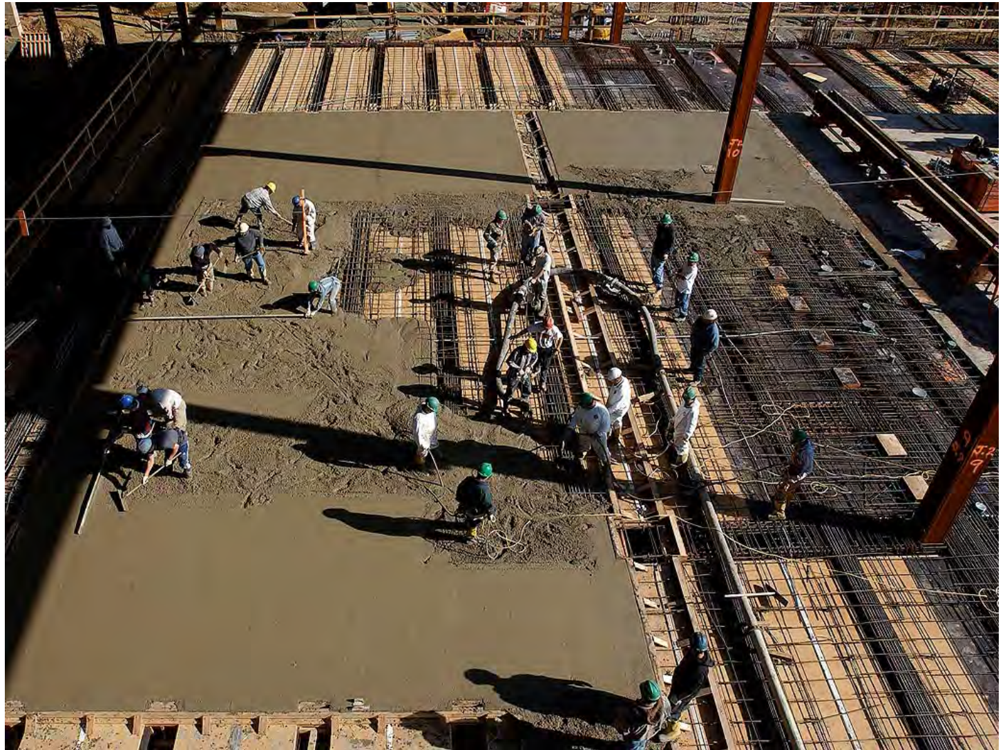
A crew guides the placement of concrete over formwork for the floor slab of the Great Hall.
