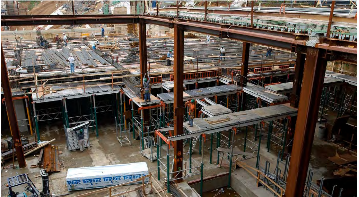
Looking east through the Great Hall's south skylight opening, workers continue to erect formwork for the upper level floor slab.
