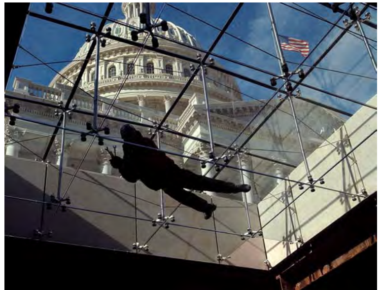
A worker secures one of 32 glass panes to a CVC skylight on the East Plaza.
