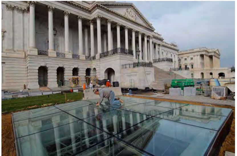
A worker installs a sealant between the glass panes of a CVC skylight located on the House side of the East Front Plaza. Other skylights will be covered for the inauguration.
