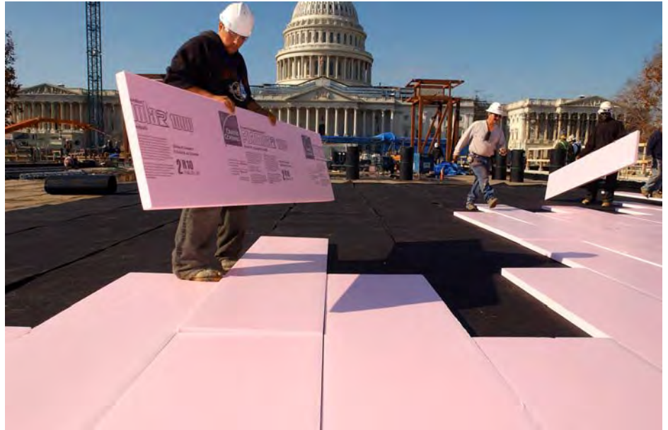
A CVC worker installs insulation board on the roof deck of the Congressional Auditorium.
