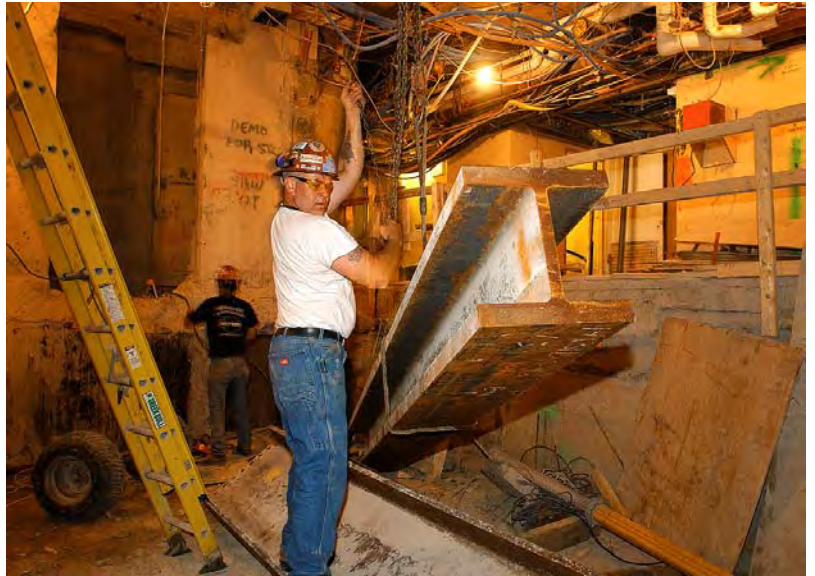
Inside the East Front, a worker uses a chain pulley to lift a steel beam in place.
