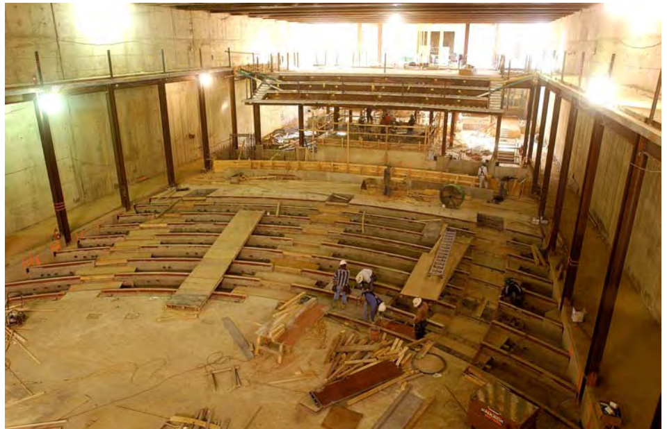
Most of the concrete slabs have been placed for the mezzanine and lower level of the Congressional Auditorium. The tiered seating structure is visible in the center of the photo.
