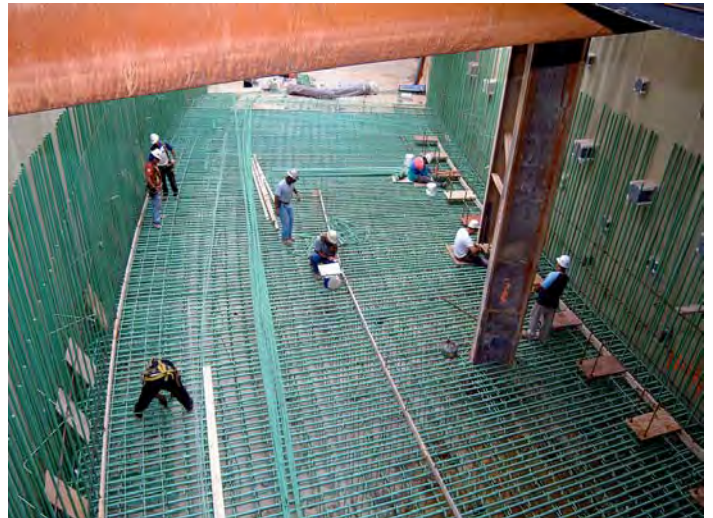
Workers assembly steel rebar for the base slab of the new truck tunnel where it approaches its connection to the CVC.
