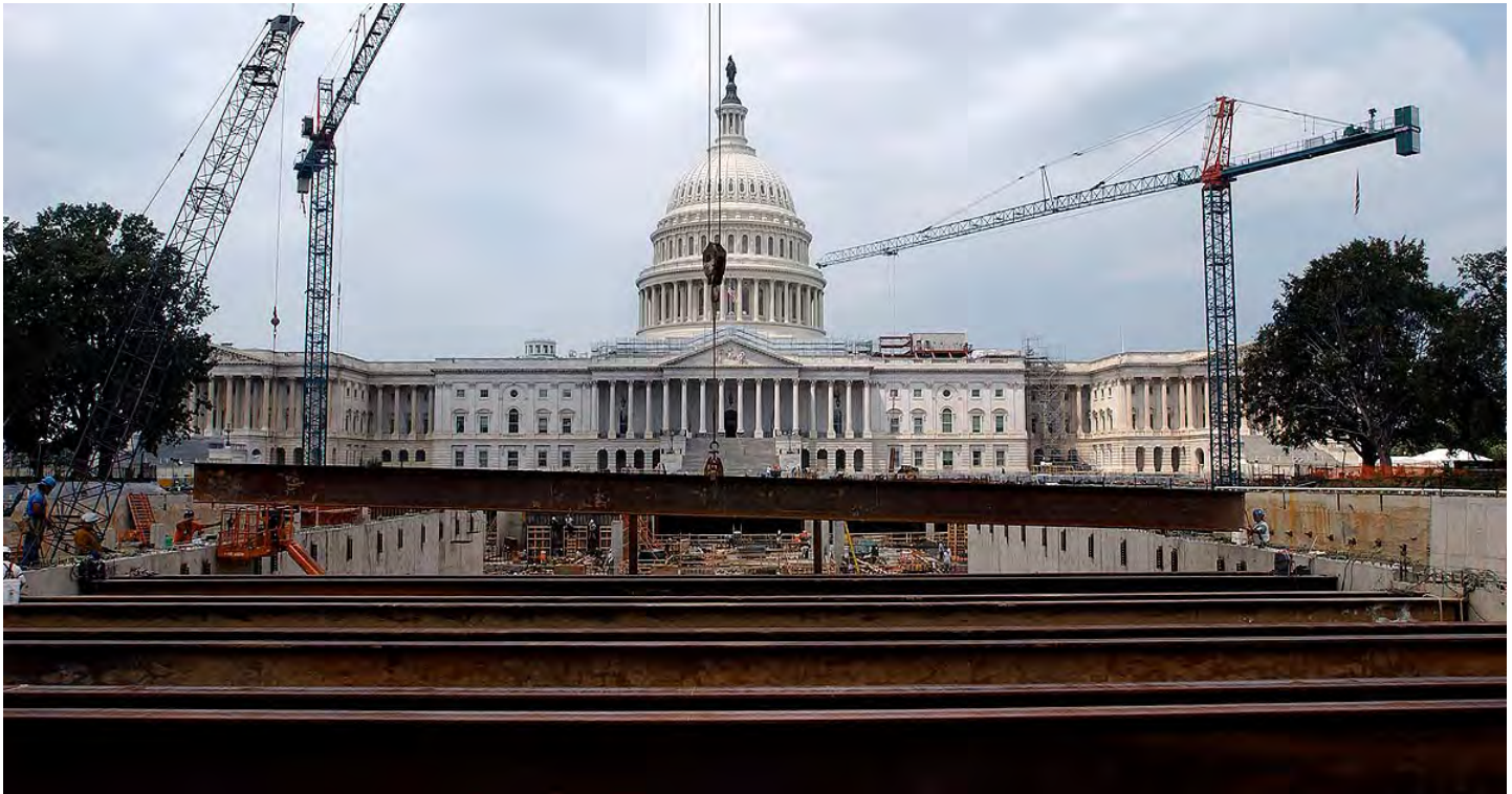
A CVC crew guides a steel crossbeam in place for the roof of the Congressional Auditorium at the eastern end of the site.
