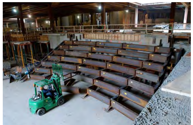
A small forklift is used to move a steel beam into place for the seating structure of one of the two CVC orientation theaters. Each theater will accommodate approximately 250 people.
