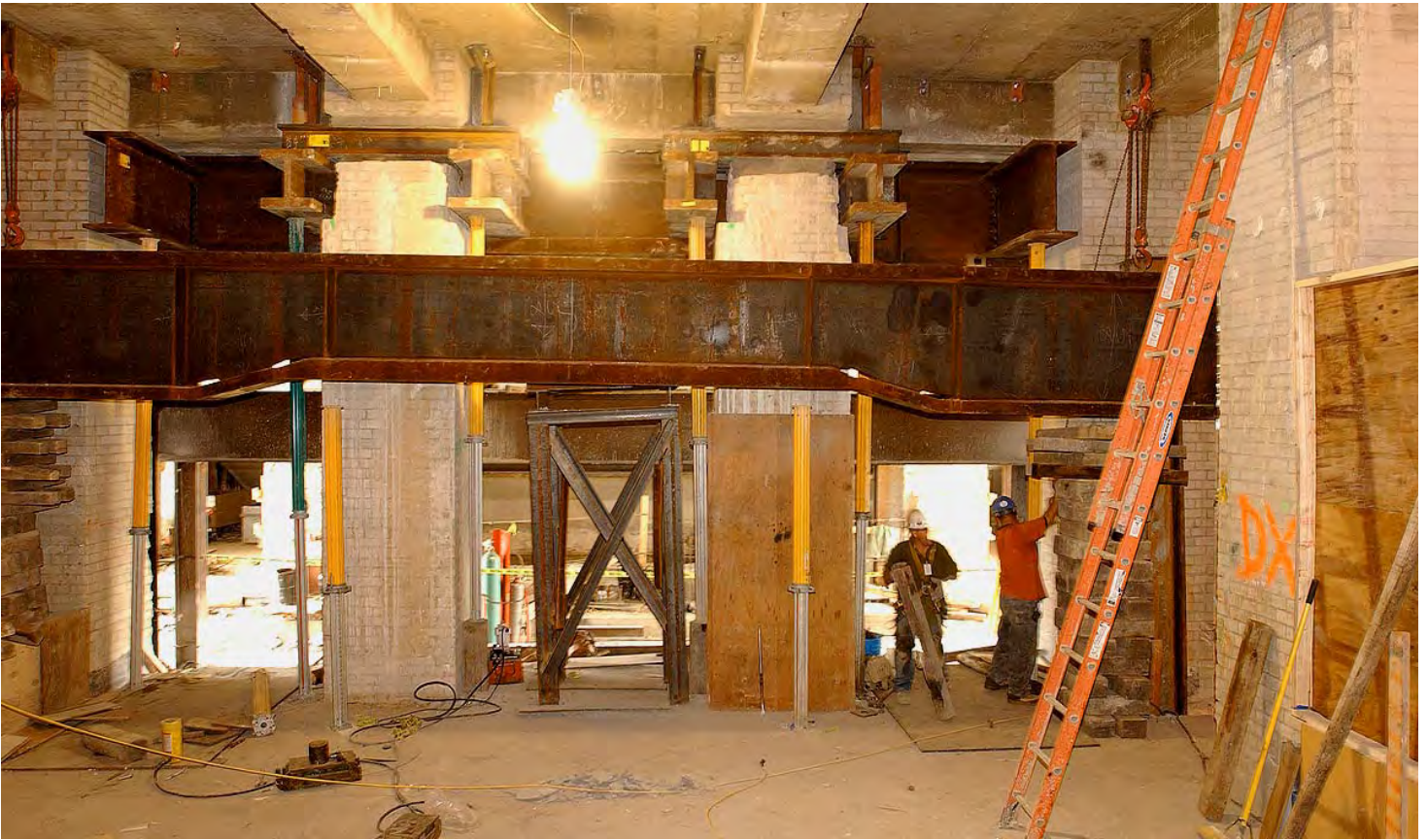
A 26,000-pound steel beam (center) is slowly raised into place to support a portion of the East Front portico above and clear the way for demolition of adjacent columns. The area depicted here, formerly known as Room EF100, a ceremonial room, will serve as the primary transition area between the CVC and the Capitol. A monumental staircase and escalators will lead approximately 12,000 visitors a day into this zone.
