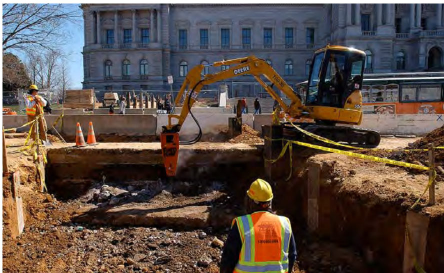
Excavation continues for a new pedestrian tunnel to the Library of Congress (background).
