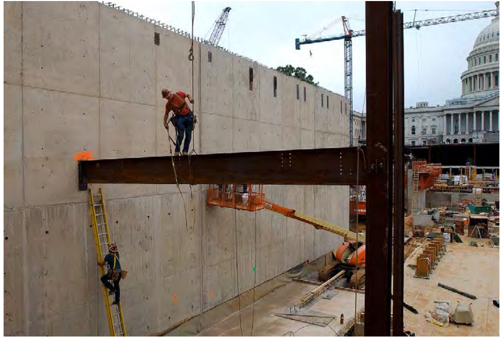
Late last week, steel workers began erecting columns and crossbeams for the Congressional Auditorium.
