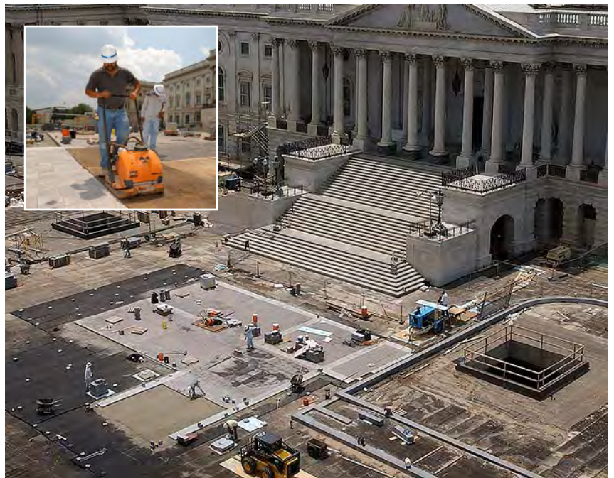
Astone crew continues laying granite pavers near the East Front Center Steps. By changing the paving bed from asphalt to a much more forgiving bed of sand and concrete, workers are able to tamp the stones (see inset) and thereby offset any surface variations in the concrete roof deck below and also compensate for minor fluctuations in the size of each paver.
