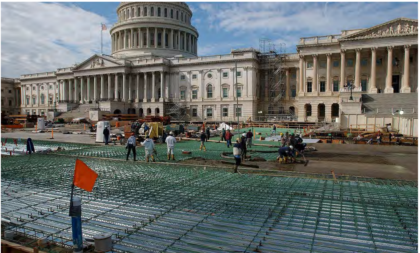
Crews guide the placement of concrete on the northern half of the CVC roof deck. The last major placement of concrete is expected to occur March 9, 2003.
