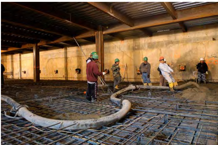
A significant concrete placement occurred last week on the upper level floor slab inside the House Expansion space.
