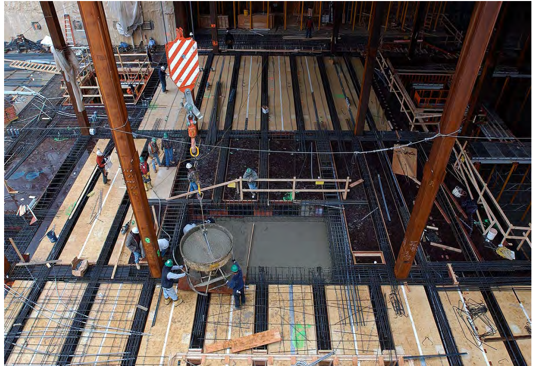
Workers have begun placing concrete for the floor slab of the Great Hall.
