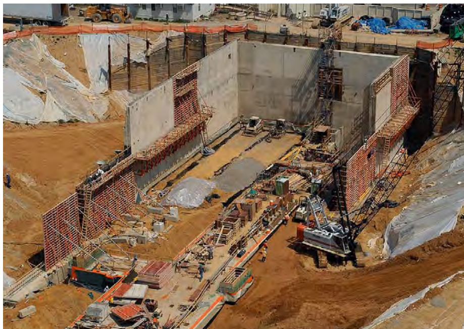
The north and south walls of the Congressional Auditorium continue to rise as construction progresses westward toward the facility’s main connection with the CVC at the center of the site.
