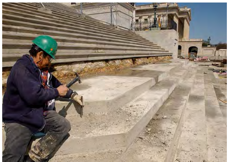
After the concrete base had cured sufficiently, a worker chiseled away any significant imperfections. The original stone step plates, which had been carefully removed, will be reinstalled on the concrete base later this spring.
