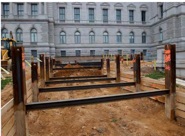
Near the northwest corner of the Library of Congress, crews have excavated the first five feet of a new pedestrian tunnel to the CVC.
