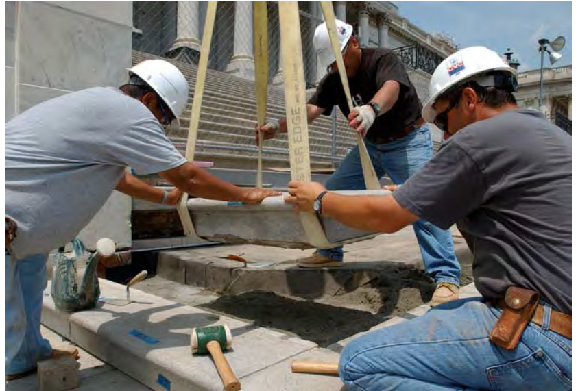
This week, a crew will complete placement of the stone slabs for the East Front Center Steps.
