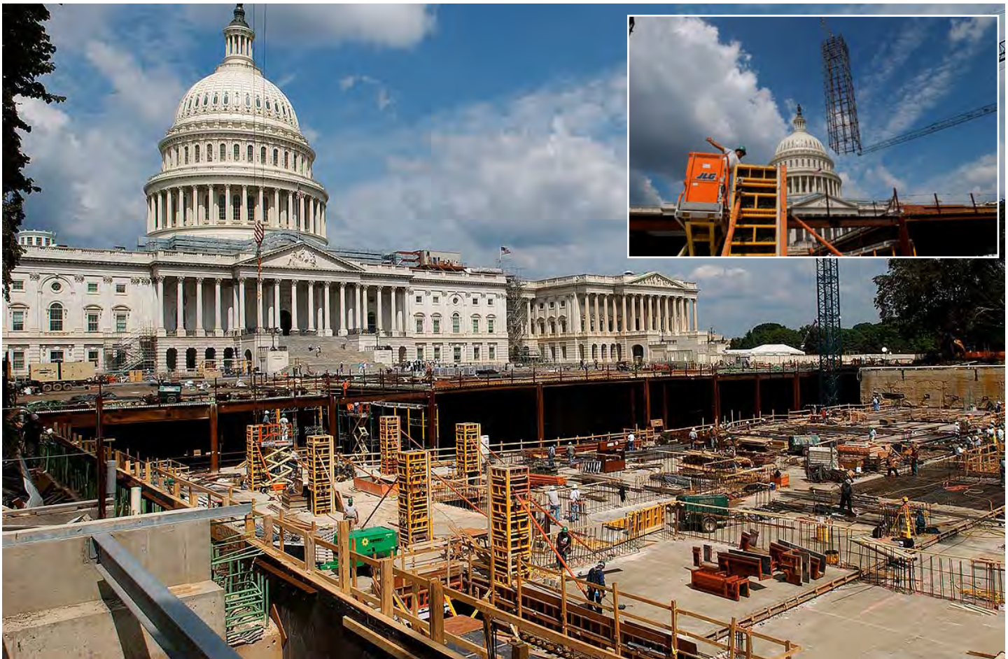
A view of the CVC's upper level floor slab (foreground) also shows the formwork for some of the columns that will support the roof deck over the eastern half of the site. Inset: A worker guides the placement of a rebar cage into a column formwork structure near the balcony of the Great Hall.
