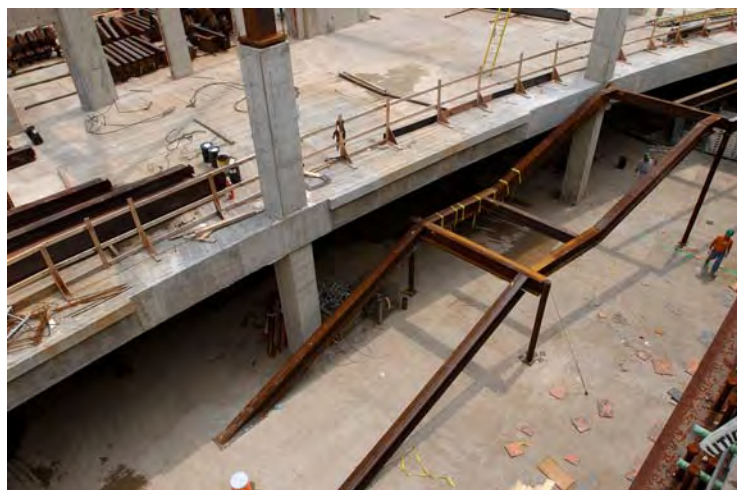
In the center of the CVC site, steel beams define the base for one of two staircases that will connect the upper level main entrance area to the floor of the Great Hall on the lower level.
