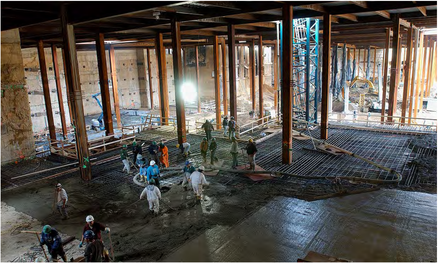
A CVC crew places concrete for the Lower Level floor slab, one level up from the slab-on-grade. After the slab cures for several days, it will support formwork for the Upper Level floor slab (where dowels protrude from the steel columns). The CVC roof deck is visible at the top of the photo.
