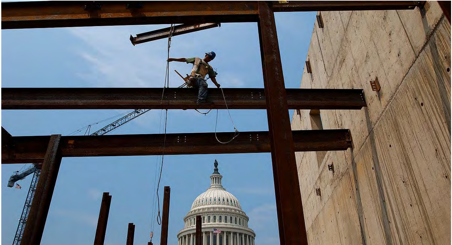
At the eastern end of the CVC site, a steel worker guides a crossbeam in place for the mezzanine structure of the Congressional Auditorium.
