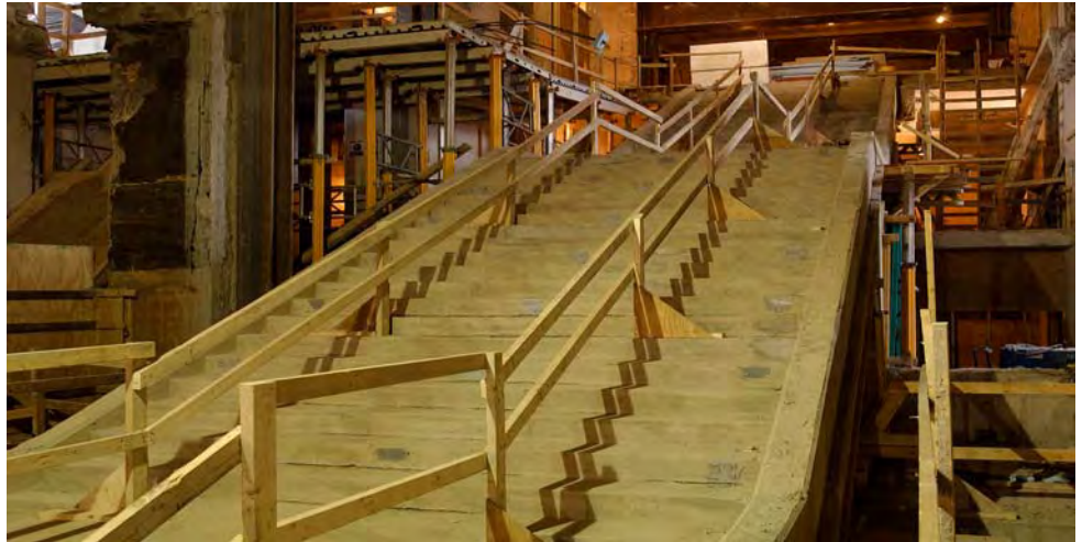
The base concrete structure for the main central staircase that links the CVC to the Capitol has been placed. Escalators will flank both sides of the staircase when this zone is completed.
