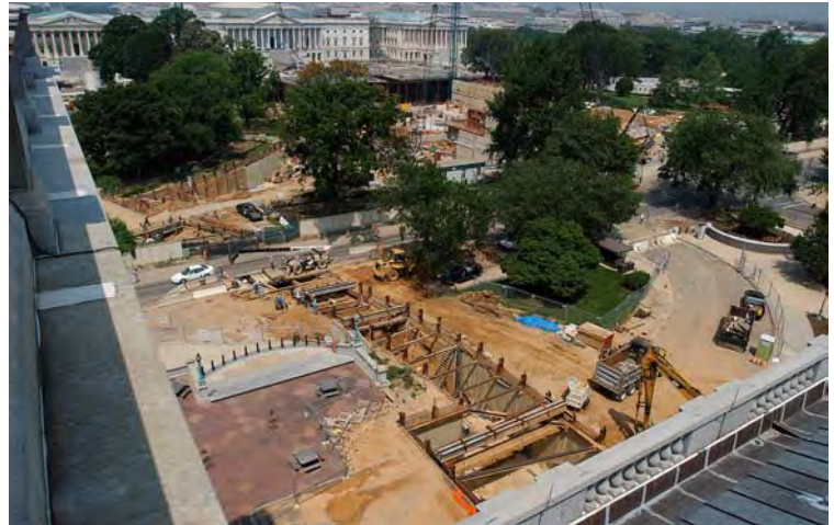
A view of the Library of Congress (LOC) pedestrian tunnel from the roof of the LOC.
