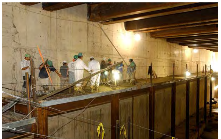
A crew places concrete for the mezzanine level of the Congressional Auditorium.
