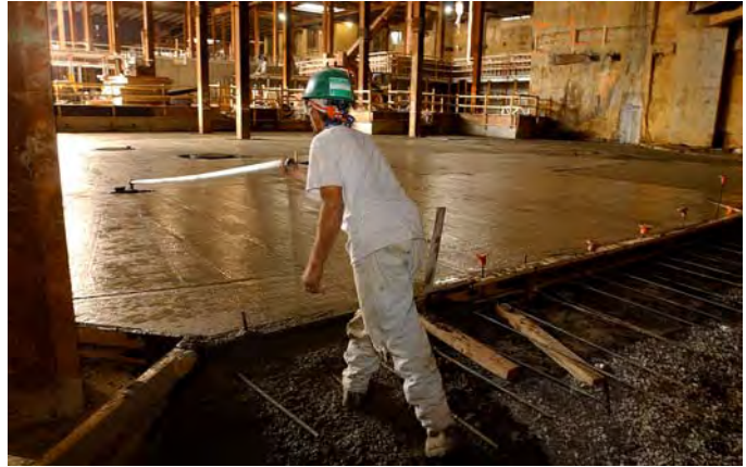
A CVC worker applies the finishing touch to a concrete slab at the north end of the site. The slab will serve as a part of a new 8-truck loading dock below the Senate expansion space.
