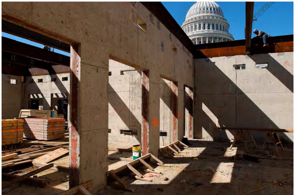
A worker (top right) secures steel for the roof deck in the northeast quadrant of the site. The openings at left are part of the CVC entrance area. Eventually, 12,000 visitors a day, nearly 3.5 million a year, will pass through this zone before entering the CVC's Great Hall.
