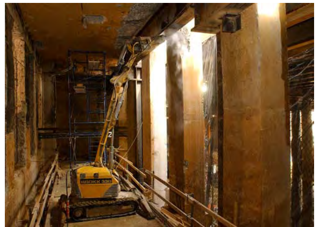
A remote-controlled mini hoe-ram is being used to demolish one of the large concrete columns below the East Front Center Steps. Eventually, this area will be occupied by a grand staircase and escalators that will bring visitors from the CVC into the Capitol.
