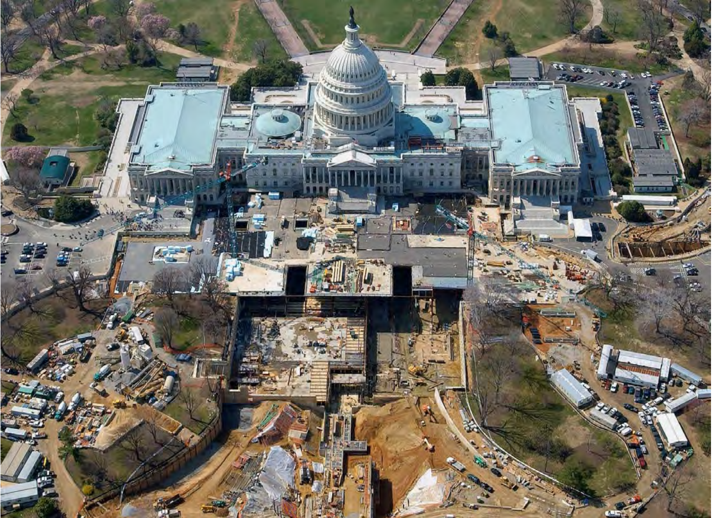
Aerial view of the CVC project site taken Thursday, March 25, 2004. A 13-inch concrete slab now covers the steel roof deck over the entire western half of the project area. Much of the first roof slab has been waterproofed and crews have now begun placing the second concrete slab. Formwork assembly, concrete placements and utility installation continue throughout the site on all three levels below the roof deck.
