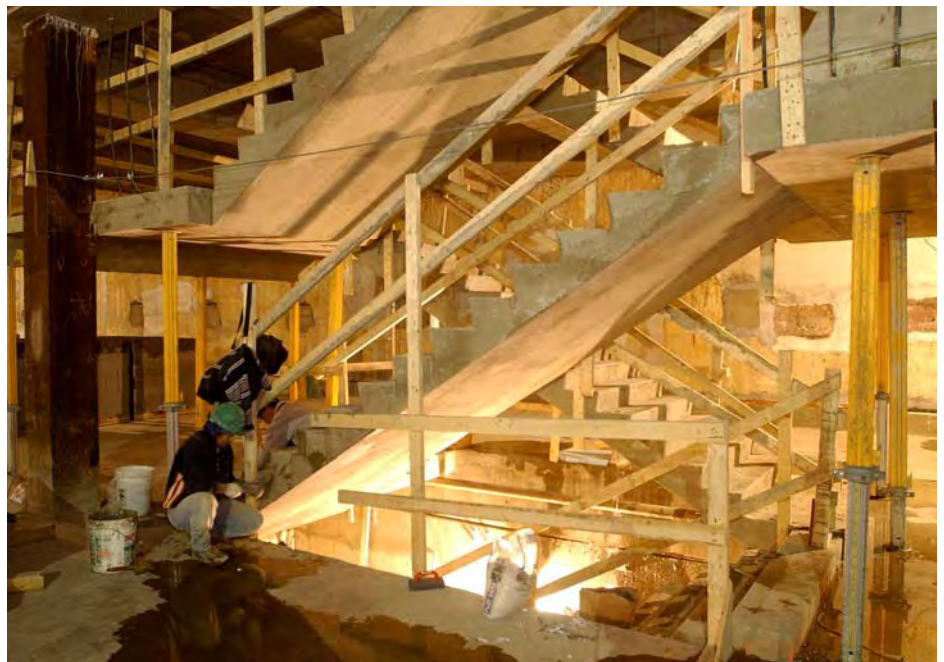
The Sequence 1 contractor, Centex Construction, has now completed all of the major structural elements of the CVC, including interior and exterior stairwells. Most of the remaining minor work in the Sequence 1 contract will be completed in December, while the structure for the tunnel to the Library of Congress will be completed in late January.
