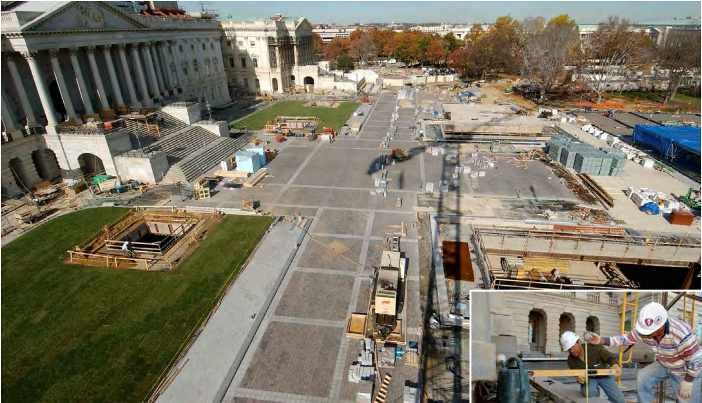
Work on the East Front Plaza deck continues on pace to support inaugural activities in January 2005. At right, workers reinstall the granite slabs on the north side of the East Front center steps.
