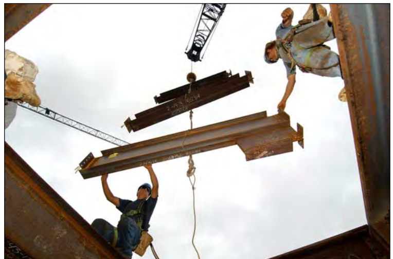
Workers set steel in place for the roof deck above the CVC entrance area.
