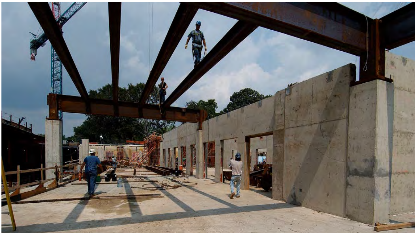
Steel workers install crossbeams for the CVC roof deck. The concrete walls at right define a portion of the visitor screening zone.
