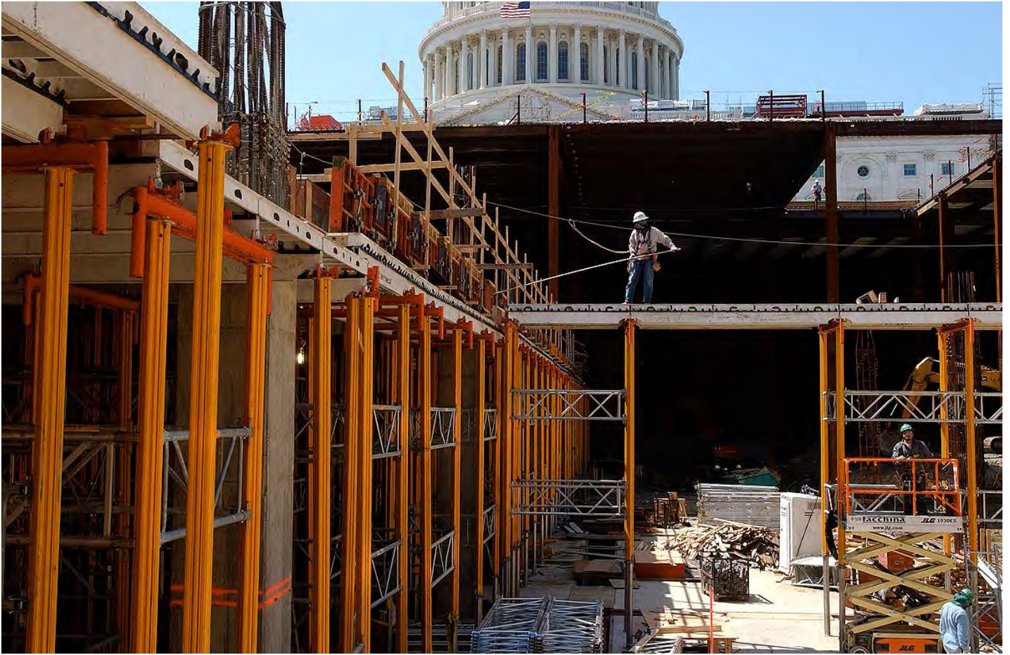
Above: A worker positions formwork for the floor slab of what will eventually become part of the CVC's 600-seat cafeteria.
