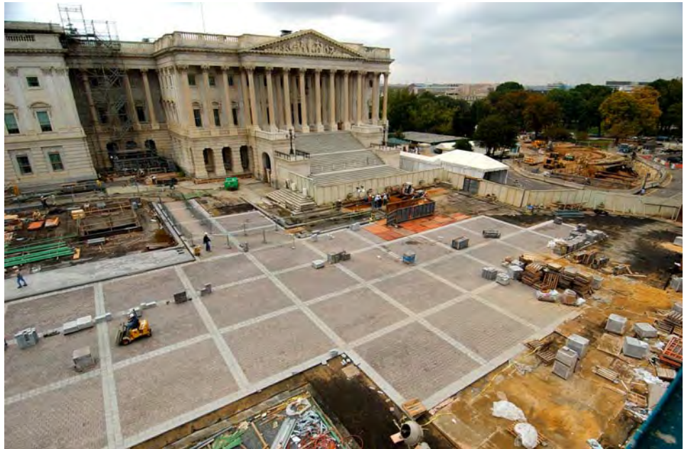
Granite paving stones have now been installed over most of the northwest quadrant of the site.
