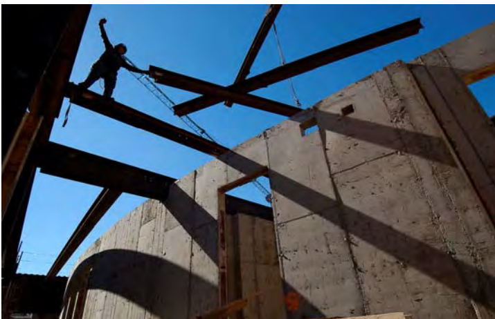
A worker guides roof steel in place above the CVC entrance structure.
