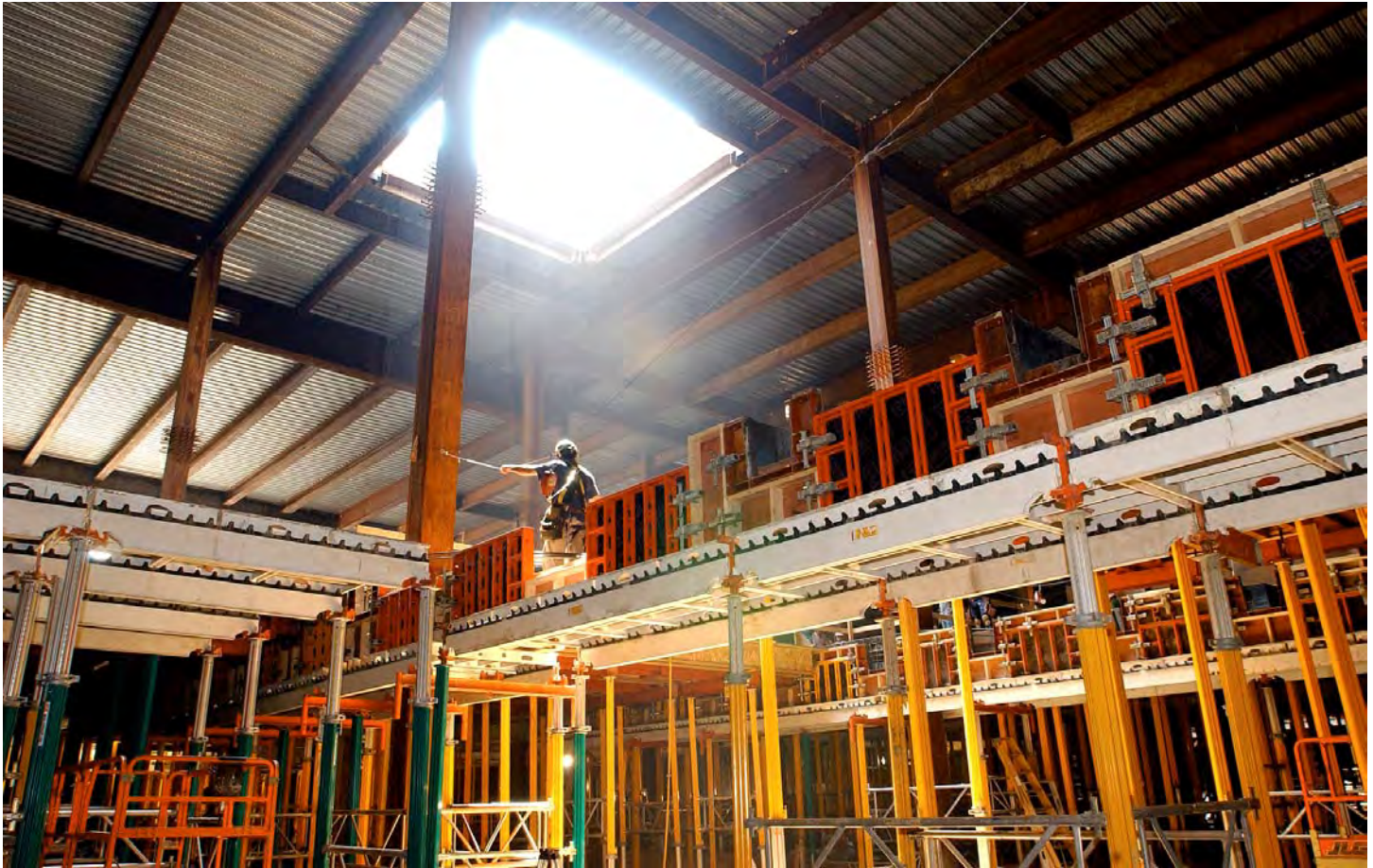
Sunlight streams through a CVC skylight opening and illuminates a portion of lower-level formwork in the southwest quadrant of the site.
