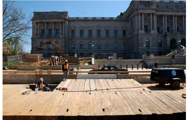
A temporary wood and steel bridge along First Street SE will minimize impacts to traffic flow while excavation for the LOC tunnel occurs below.
