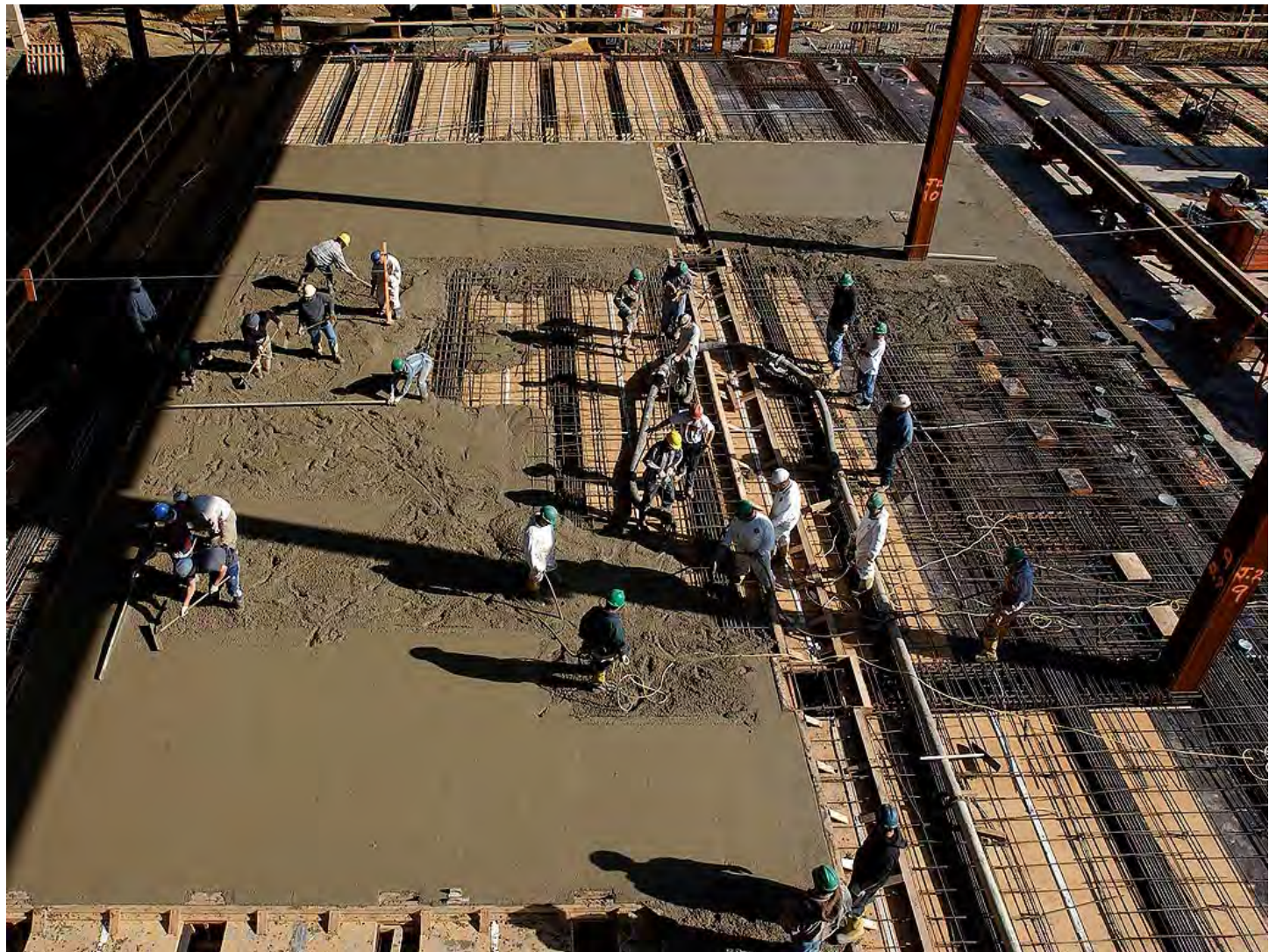
A crew guides the placement of concrete over formwork for the floor slab of the Great Hall.
