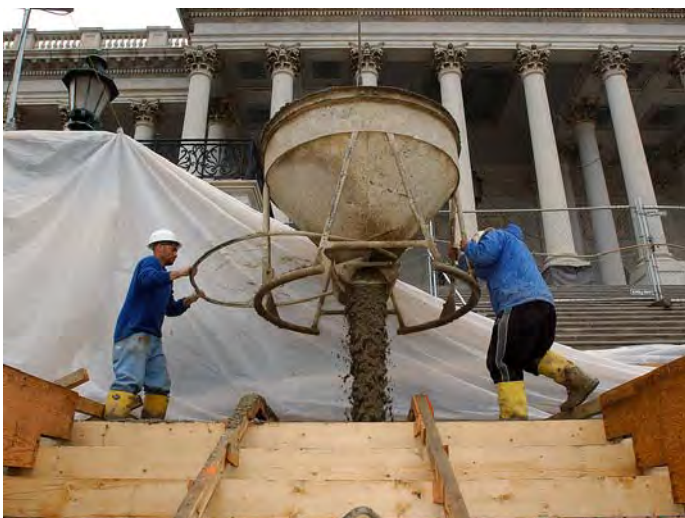
During a break in the persistent rainfall last week, workers placed concrete into the formwork for the lower base of the East Front Center Steps.
