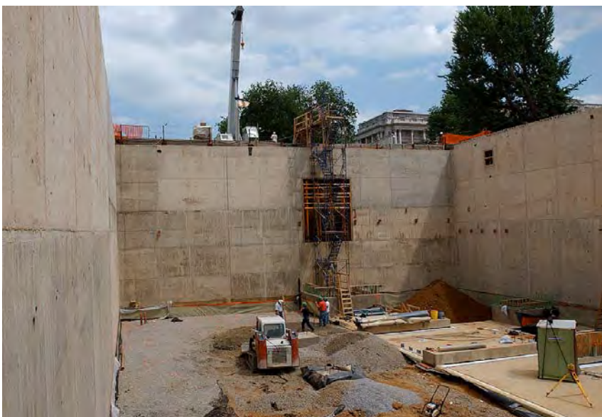
The Congressional Auditorium continues to take shape at the eastern end of the CVC site.
