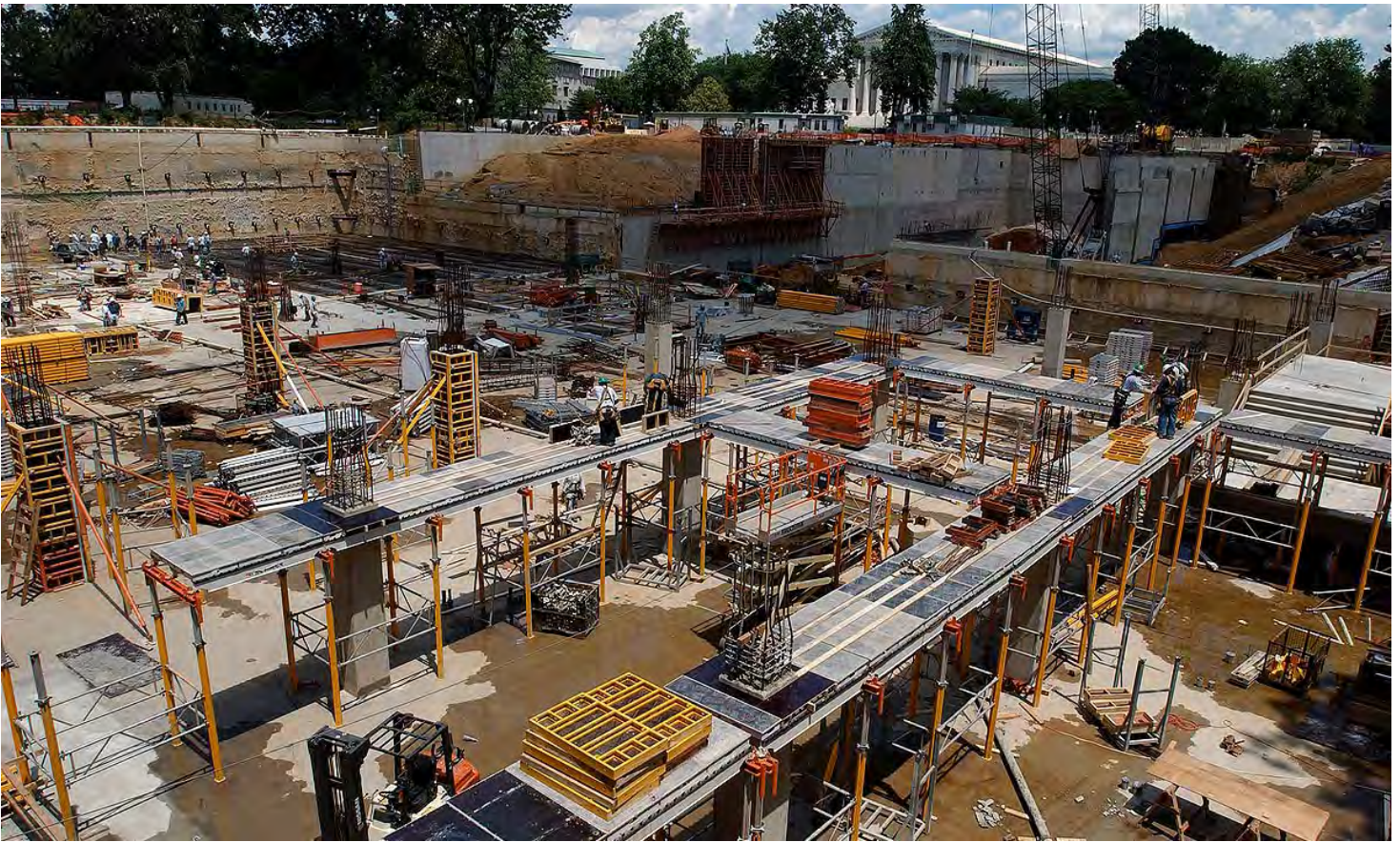
After the holiday weekend, crews returned June 1 to continue placing concrete (top left of photo) and assembling formwork for the upper level floor slab (center).
