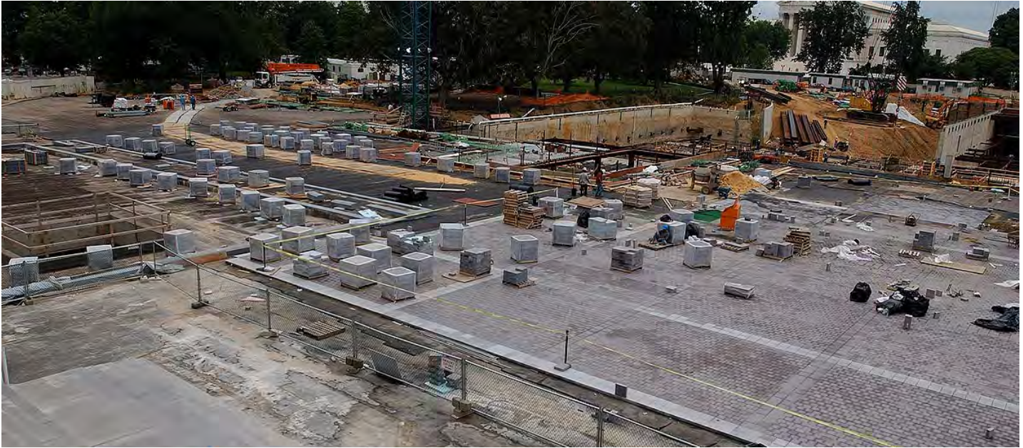
Dozens of crates of granite paving stones are lined up on the CVC roof deck. Approximately 75,000 8-inch-square pavers will be laid by the time Congress returns from recess in September as crews begin a strong push toward paving the entire western half of the plaza by the Inauguration in January 2005.
