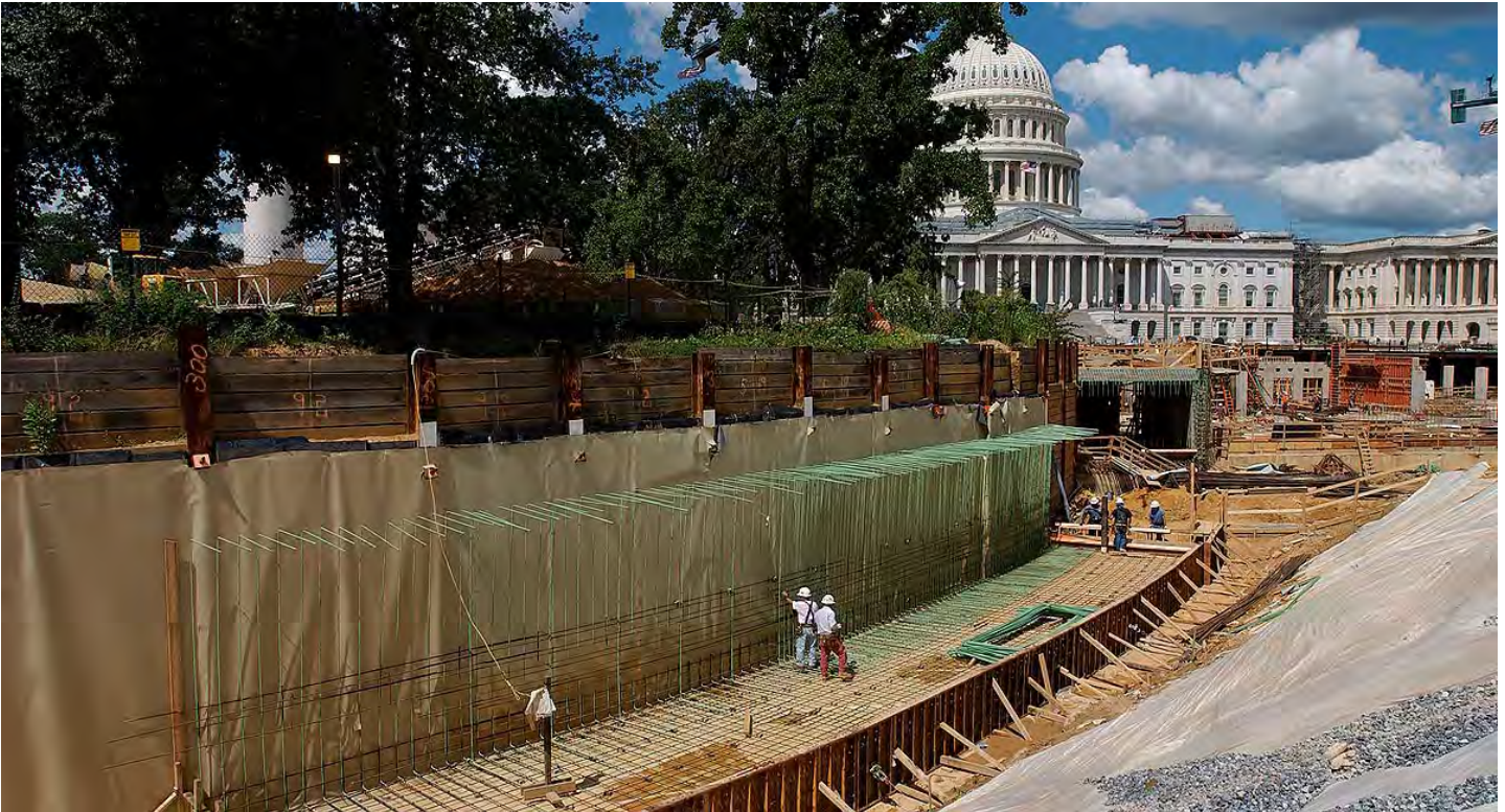
A CVC crew assembles rebar for the interior wall of the pedestrian tunnel to the Library of Congress in the southern half of the site.
