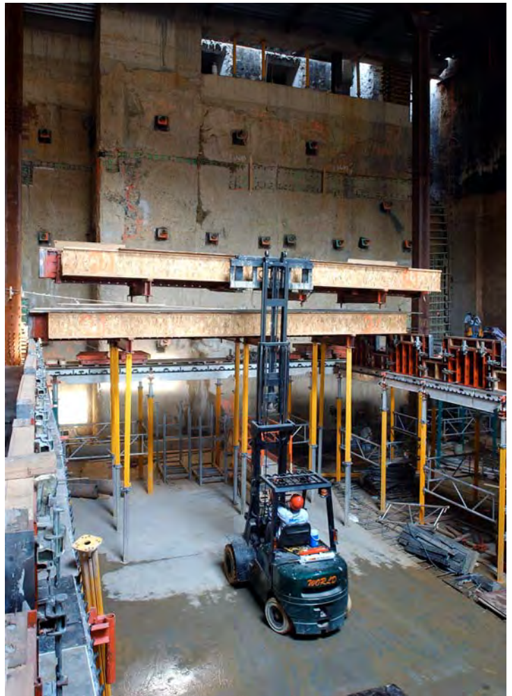
A forklift raises formwork beams in place for the floor slab of the CVC Exhibition Gallery. The 16,500 square-foot Gallery will span nearly 300 feet across and will have more than twice the floor space of the Capitol's Rotunda.
