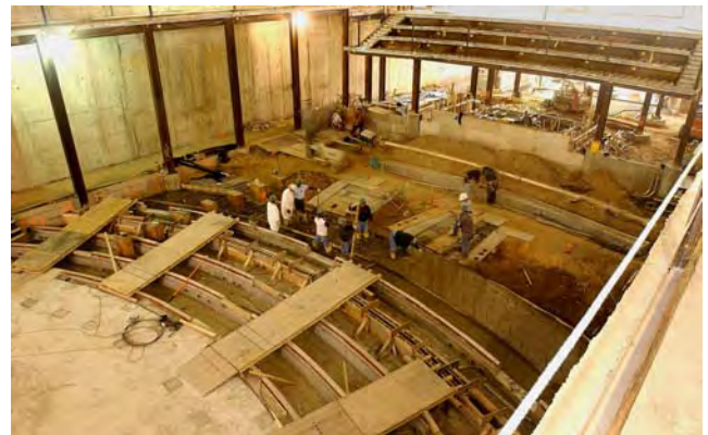
A CVC crew places concrete in formwork for the tiered seating structure on the lower level of the Congressional Auditorium.
