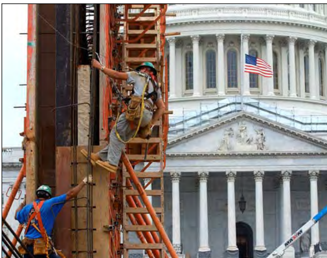
In the eastern half of the CVC site, workers assemble the formwork for the upper half of the Congressional Auditorium's south wall.
