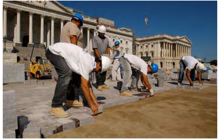
Installation of granite pavers on the western half of the East Front Plaza is a top priority in order to accommodate inaugural activities in Jan. 2005.
