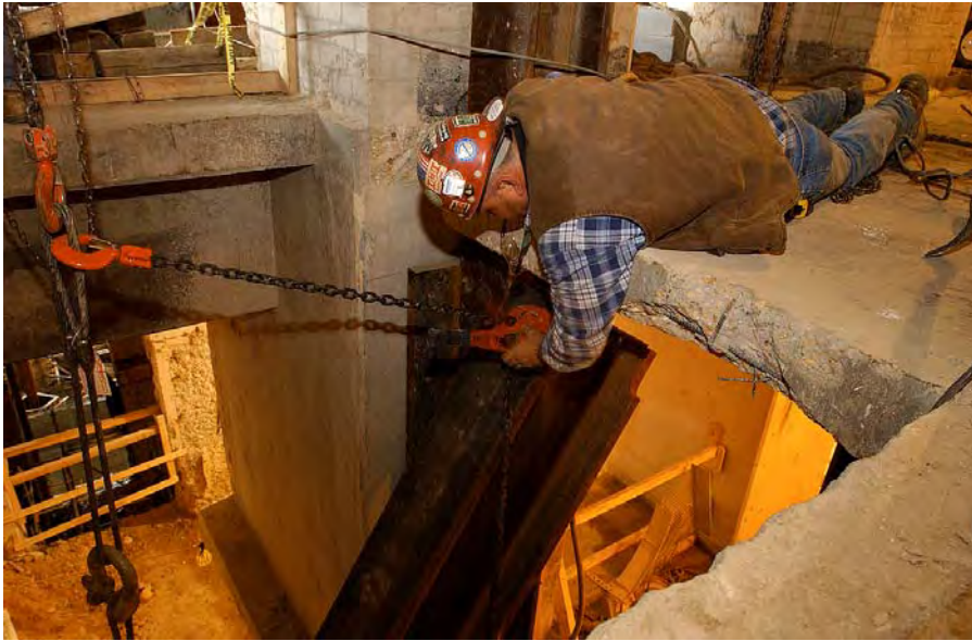
A worker guides a steel beam in place inside the East Front Extension.
