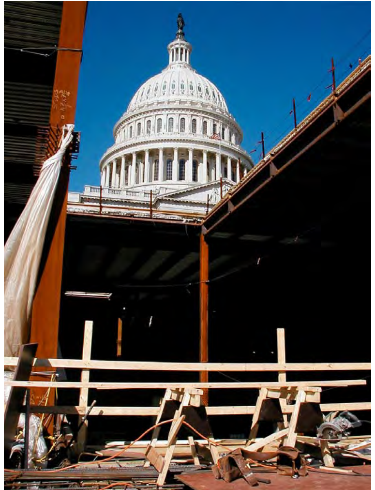
Above: With the formwork in place for a portion of the floor slab of the Great Hall, one can see the actual view that visitors will have of the Capitol Dome through the Great Hall's south skylight.
