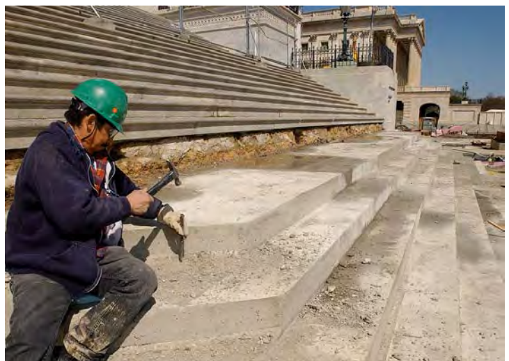
After the concrete base had cured sufficiently, a worker chiseled away any significant imperfections. The original stone step plates, which had been carefully removed, will be reinstalled on the concrete base later this spring.
