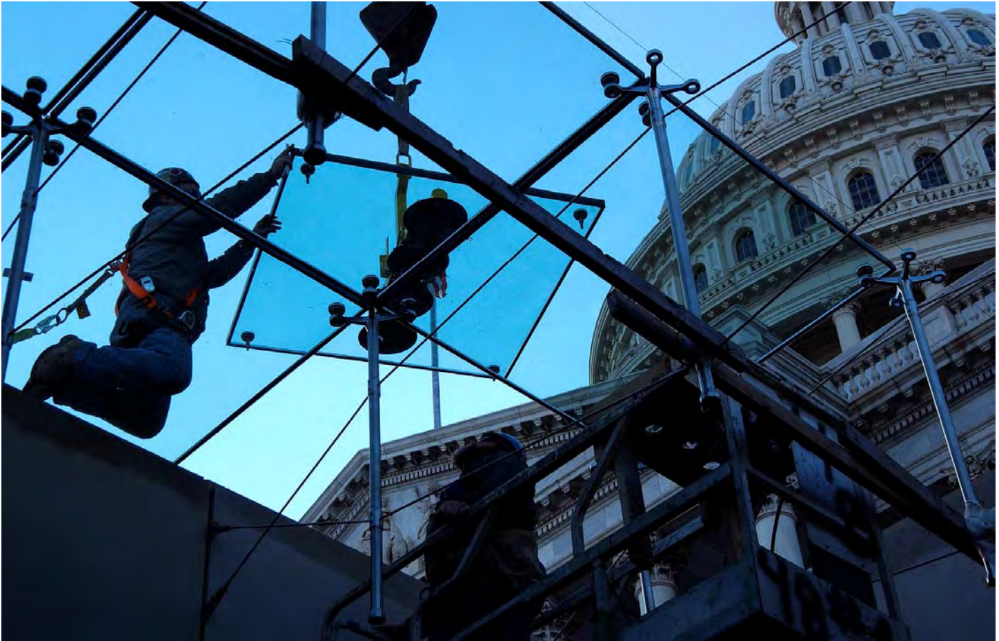
A worker installs a glass pane for one of four skylights near the face of the Capitol on the north side of the Plaza.
