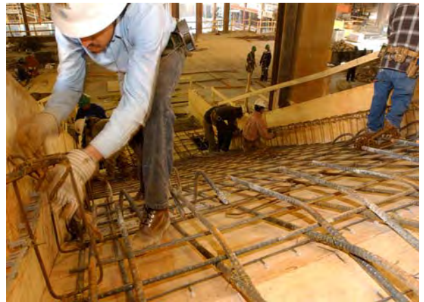
Workers assemble steel rebar for the main central staircase that will connect the CVC to the Capitol at the Crypt level.
