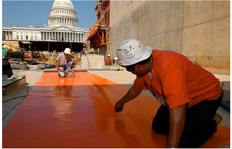
Workers measure a section of a waterproofing membrane that will be used to line a portion of the concrete structure of the Congressional Auditorium.
