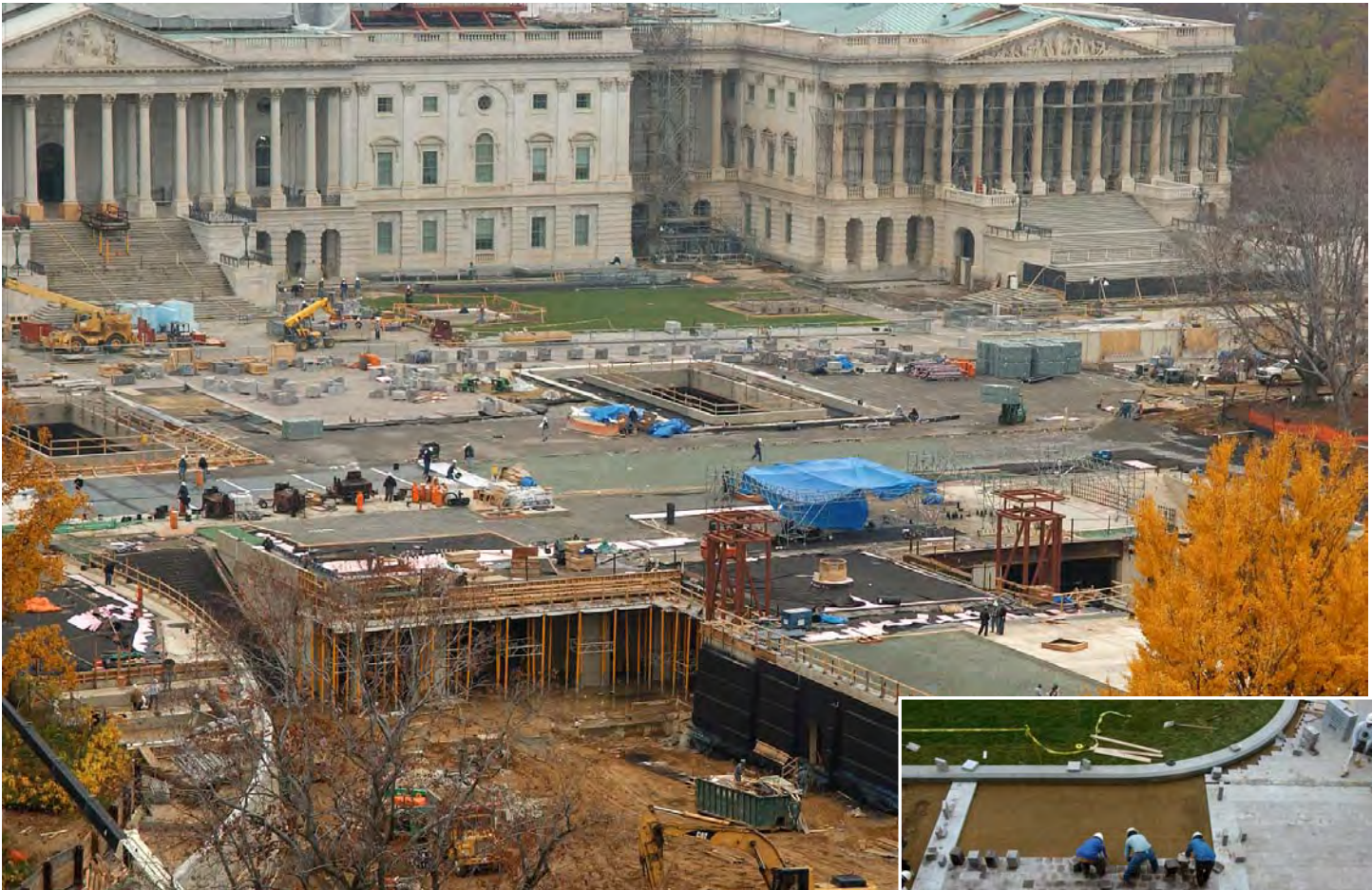
A view of the CVC from the Library of Congress shows work on the East Front Plaza deck progressing on pace to support inaugural activities in January 2005. Inset: Stone crews place granite paving stones near the grassy bed in front of the original Senate Wing.
