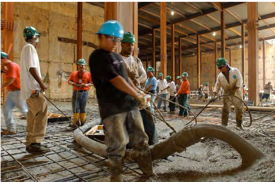
Workers place concrete in the northwest quadrant of the CVC service level.
