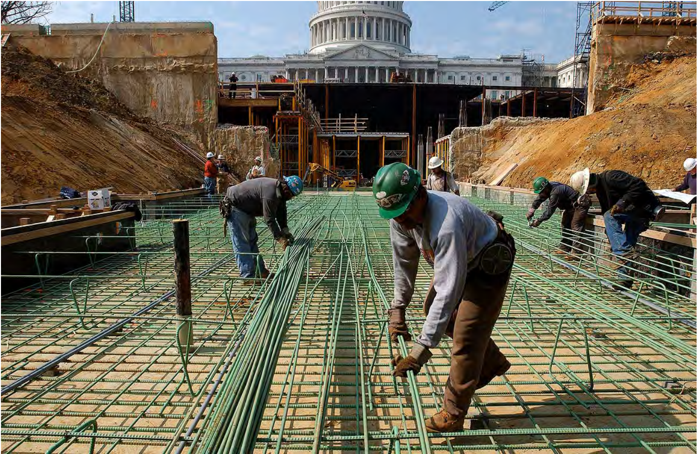
Crews assemble steel rebar for the floor slab of the Congressional Auditorium in the easternmost portion of the CVC site.
