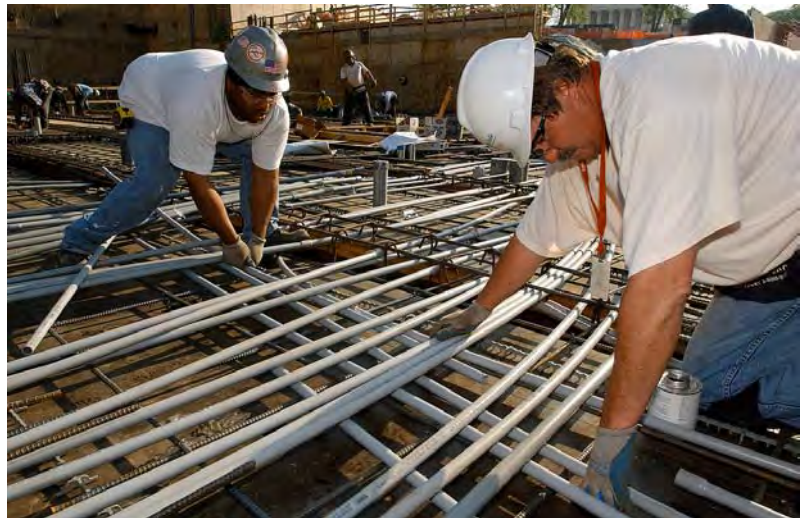
Sequence 2 contractors are busy laying miles of electrical conduit piping within the reinforcing steel for the concrete floor slabs. The conduit must be spaced properly to ensure that there are no significant structural gaps within the concrete slabs.
