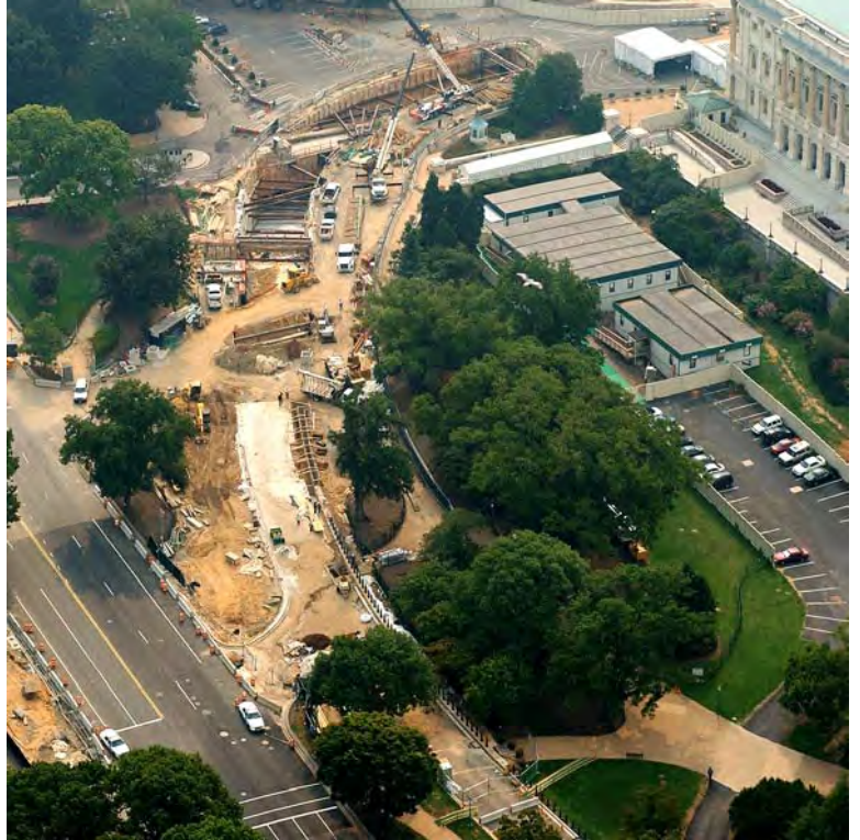
Taken in late August 2004, this aerial view of the new service tunnel along Northwest Drive near the Senate wing (top far right) shows only the southeastern-most portion of the tunnel (top center) remaining to be back-filled. Pedestrian access, staff parking along the drive, and landscaping elements will be restored later this fall.
