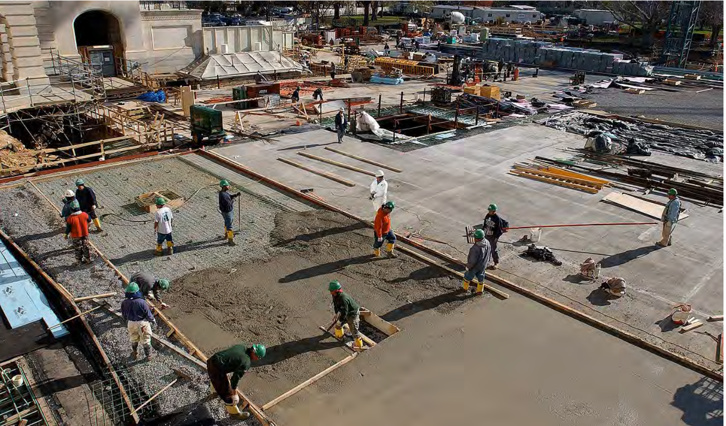
During the week of April 5-9, 2004, workers began placing the second concrete slab on the CVC roof deck in front of the original Senate wing.
