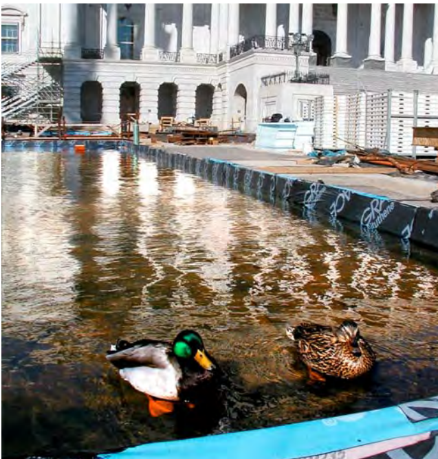
Left: Waterproofing inspectors? Not exactly, but one waterproofing zone on the CVC roof deck has lured at least two ducks to test the waters on the East Front Plaza.
