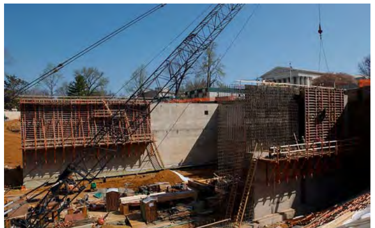
Below right: Construction of the north and south walls of the Congressional Auditorium continues westward. The roof of the auditorium will serve as the East Capitol Street Extension.
