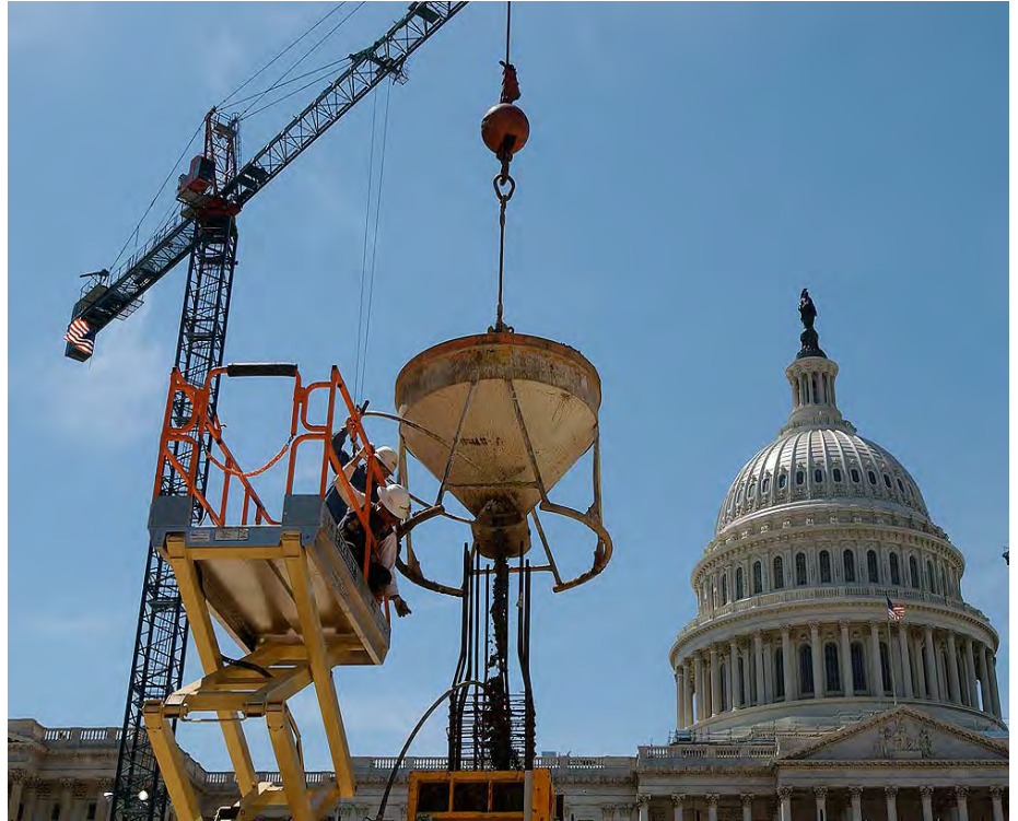
In the southeastern quadrant of the CVC site, workers guide a large bucket containing concrete to its release point at the top of a column formwork structure.
