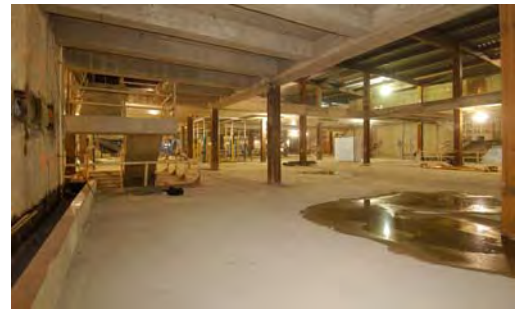
Clearing out: The Sequence 1 contractor, Centex Construction, has now completed all of the major structural elements of the CVC and has now begun clearing personnel, materials and equipment from the site.
