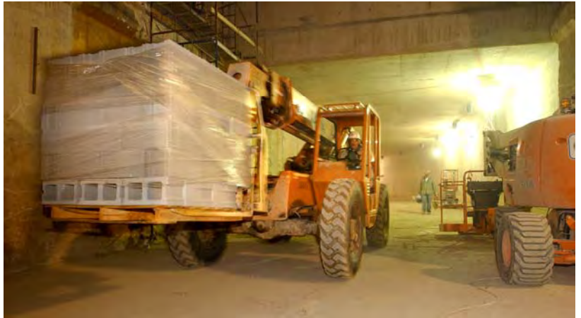
CVC Milestone: The first trucks to use the new CVC truck tunnel on the north side of the Capitol began rolling in at 8:00 AM on Monday, November 15, 2004.
