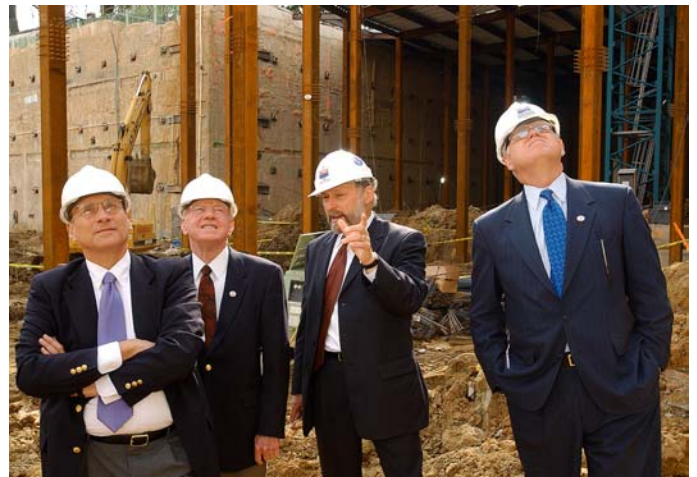
Standing 55 feet below grade in the center of the CVC site, (from left) Rep. John Mica (R-FL), Rep. Vernon Ehlers (R-MI), Architect of the Capitol Alan Hantman, and Rep. John Larson (D-CT) observe demolition activities below the East Front Center Steps during a site visit October 21, 2003.
