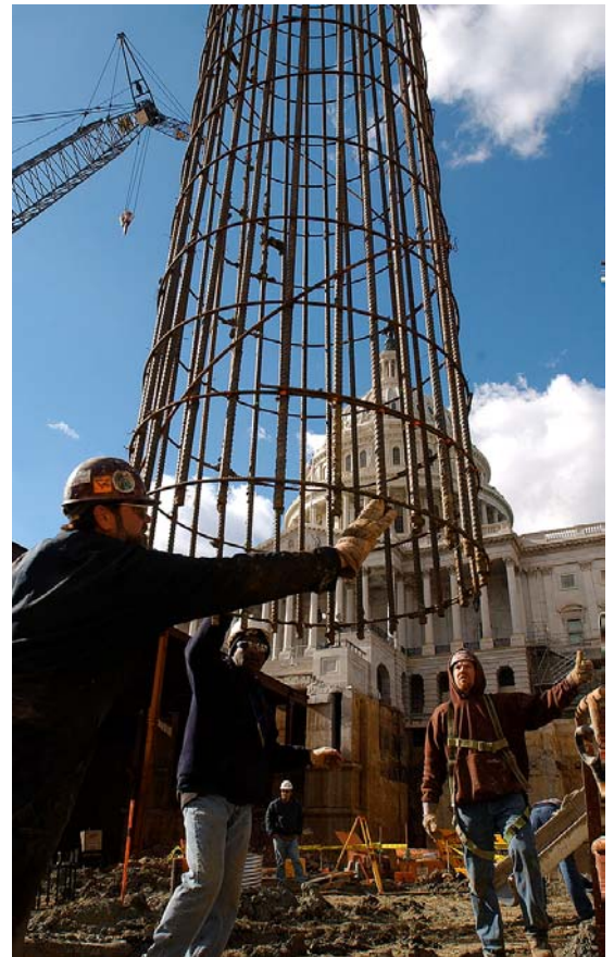
Workers guide a cylindrical steel rebar cage into a caisson trench. A caisson is a concrete footer that serves as the foundation for each steel or concrete column that is erected on site. The last of 186 caissons may be completed by the end of this week.
