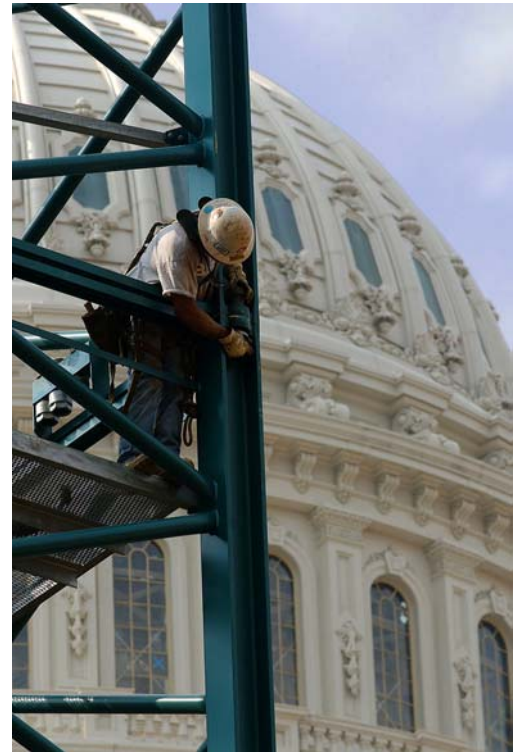
Nearly 200 feet above ground, a worker connects two sections of a new tower crane erected on the CVC site on Saturday, September 27, 2003.
