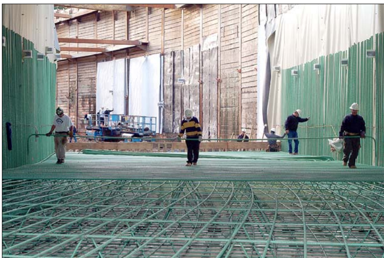
Last month, on the north side of the Capitol, workers inside the new truck tunnel laid steel rebar along the base of the tunnel to prepare it for placement of a concrete road bed.
