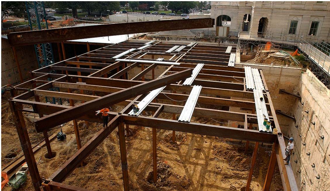
Steel workers guide a crossbeam into place near the face of the Capitol between the House Steps and Rotunda Steps. Steel roof decking will be installed over the next several weeks and then covered with a 13-inch concrete slab. When completed, the roof deck will have a thickness of 27 inches.
