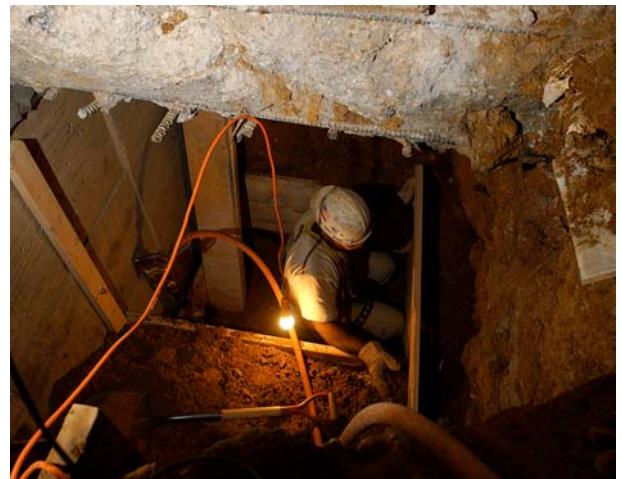
In the basement level of the East Front Extension, CVC construction crews often work within extremely tight conditions that require workers to excavate the old-fashioned way—with shovels and buckets.
