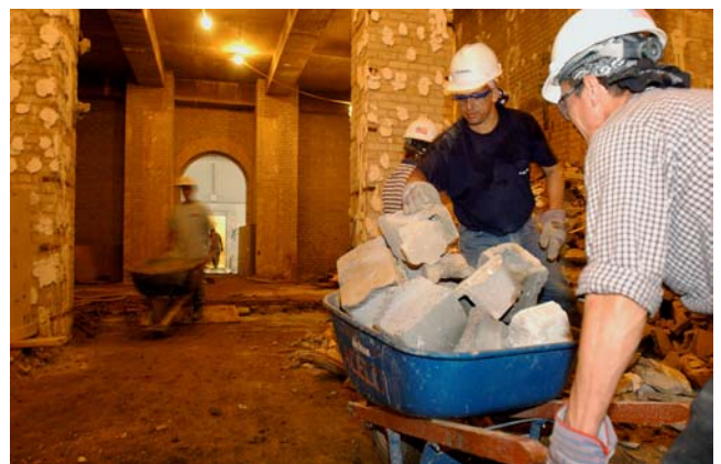
Demolition crews continue to remove tons of debris from the East Front. Here, workers pile concrete rubble in an area that formerly housed the Capitol Historical Society gift shop.
