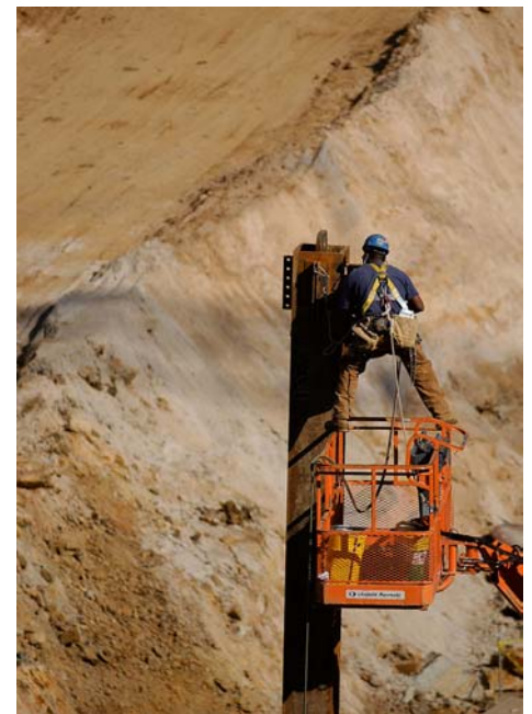
In the center of the CVC site, a worker welds a steel clip at the top of a 50-foot-high steel column. A dirt access ramp, visible in the background, provides vehicle access to the site.
