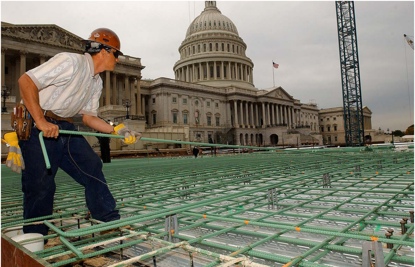
A worker positions steel rebar on the roof deck of the CVC in the southwest quadrant of the project area. The rebar will serve as structural reinforcement for the first of two concrete slabs that will be placed on the roof deck. The green epoxy coating on the rebar prevents rusting.
