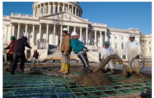
A crew guides the placement of concrete on a portion of the CVC roof deck in the center of the site.
