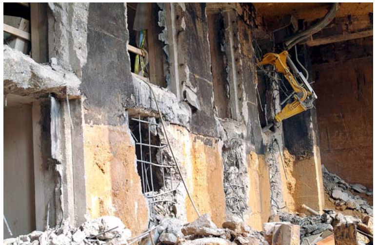
A remote-controlled mini hoe-ram (top right of photo) continues demolition of structural elements below the East Front Steps. This zone will house the grand stairwell and escalators that will connect the CVC to the Capitol.
