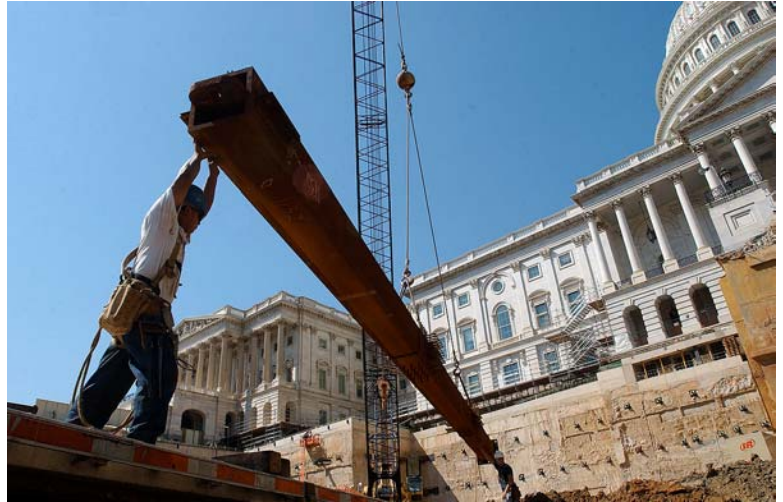
Man of steel: A worker guides a steel crossbeam into position in the southwest quadrant of the CVC site.
