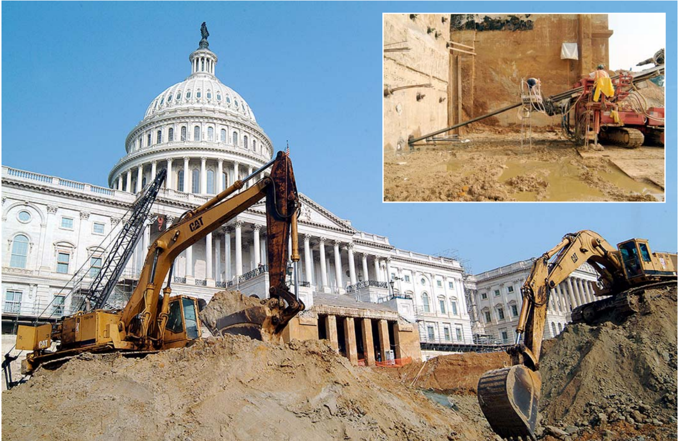
Excavation (above) and installation of tiebacks (inset) continue to be the dominant activities on the CVC project site. (Photos from 8/8/03)
