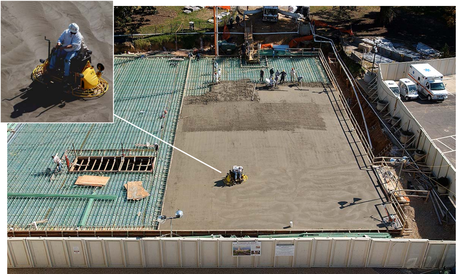
Looking east from atop the House Steps last Friday, October 24, 2003, a crew is seen leveling the first concrete slab placed on the CVC roof deck. Inset: Once concrete sets a while, a sit-on trowel machine that rides on two rotating blades is used to make the concrete surface smooth and level.
