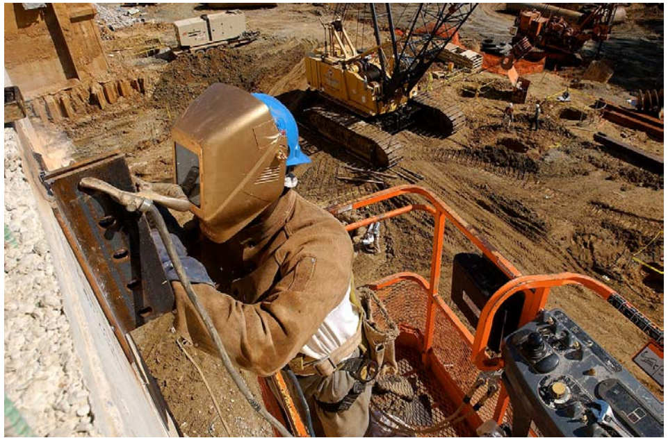
Elevated 50 feet aboveground, a welder secures a steel crossbeam support clip to the perimeter wall in the southwest quadrant of the site.
