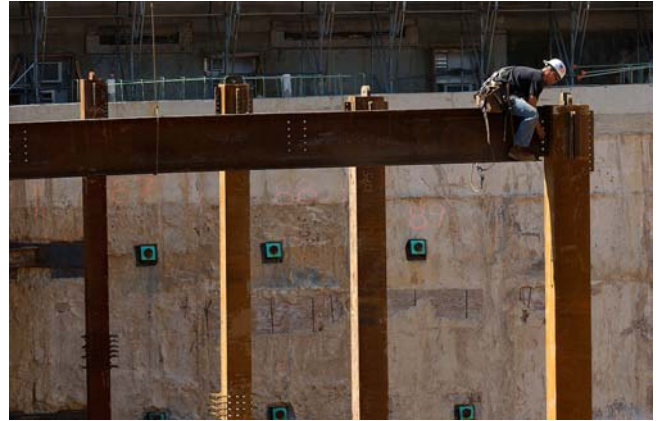
A worker secures a steel crossbeam to a column in the southwest quadrant of the CVC site.
