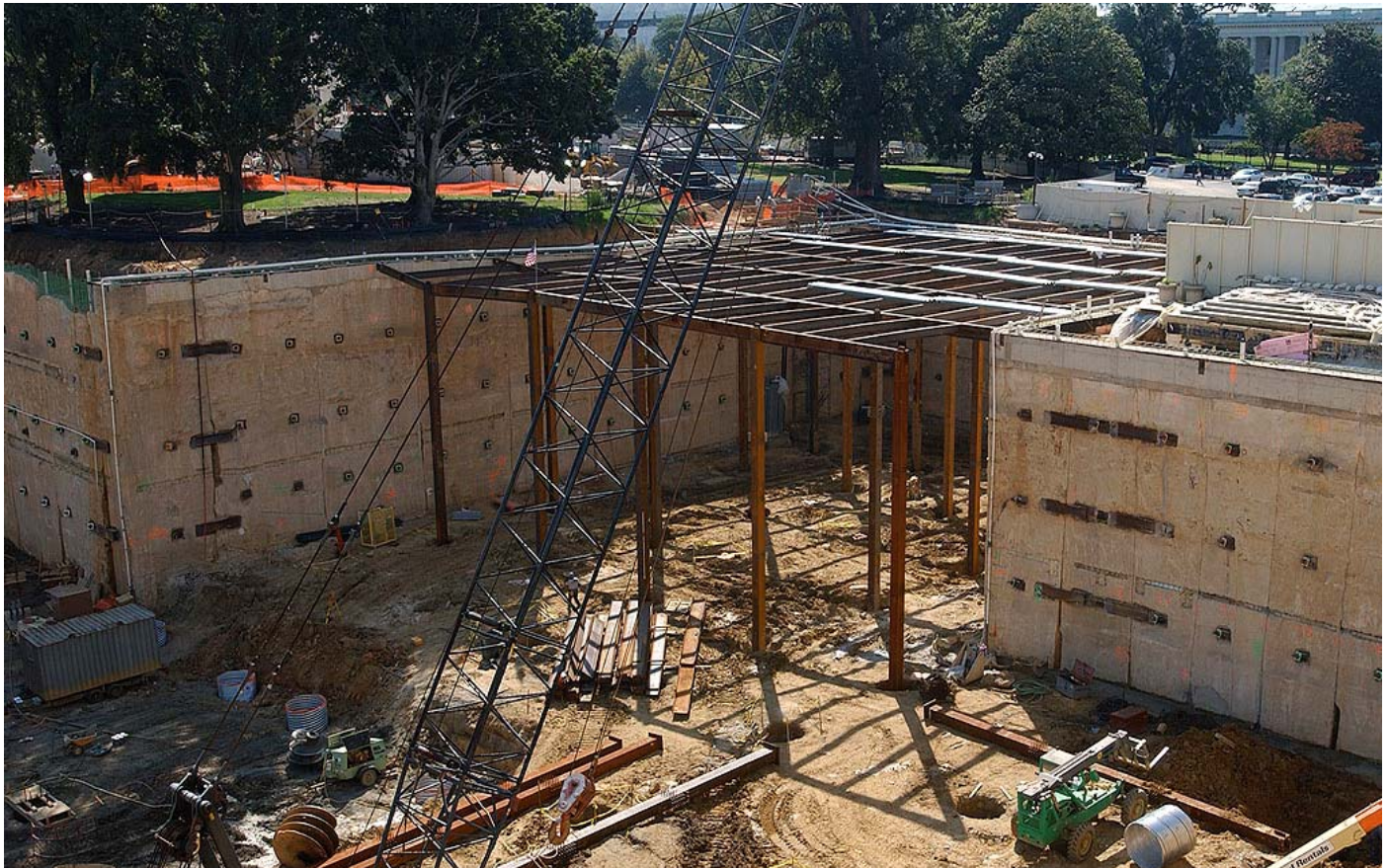
The steel structure of the CVC begins to take shape in the southwest quadrant of the site in the area to be occupied by House expansion space.
