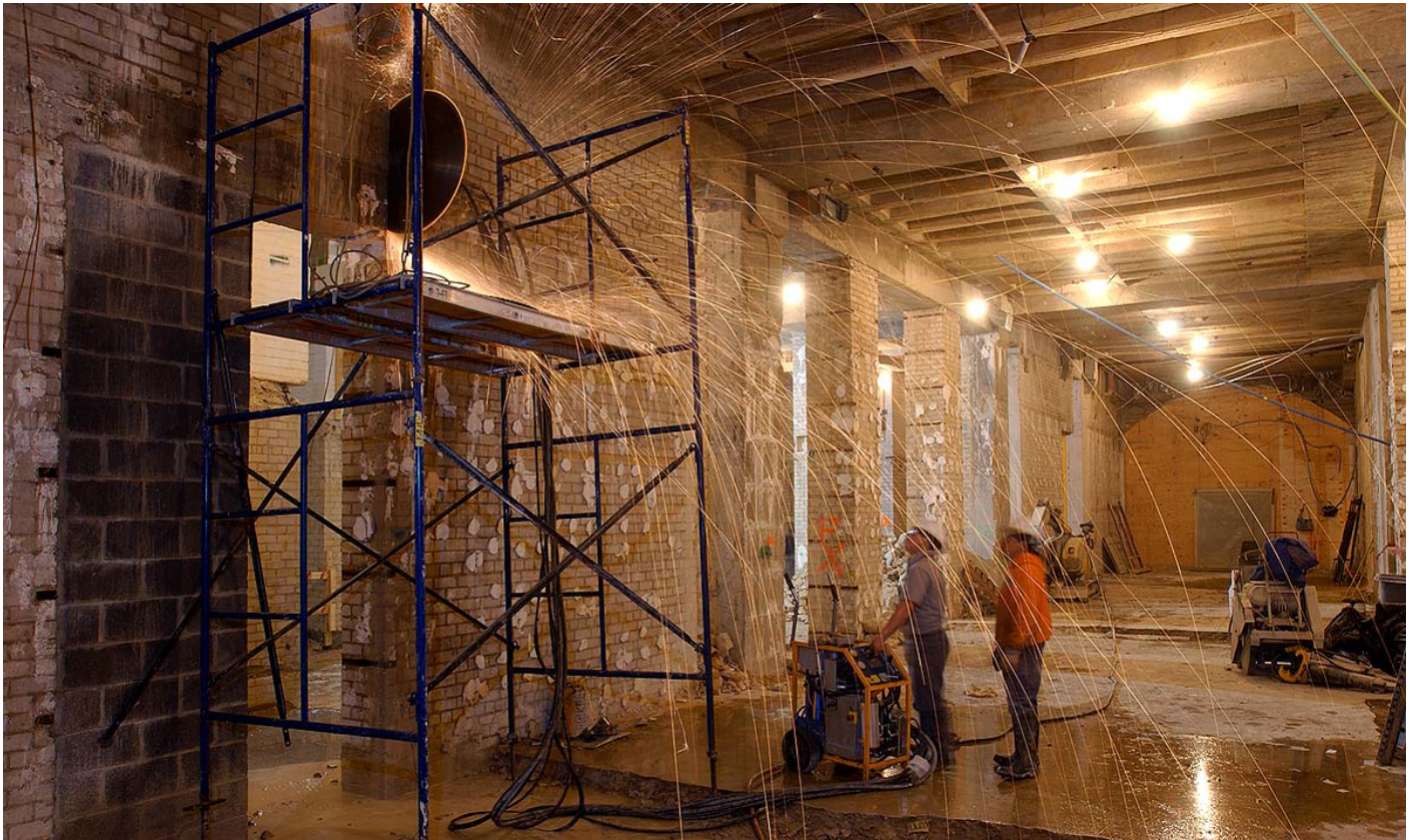
Demolition crews continue saw-cutting through walls to clear the way for new elevators, escalators and mechanical rooms in the East Front.
