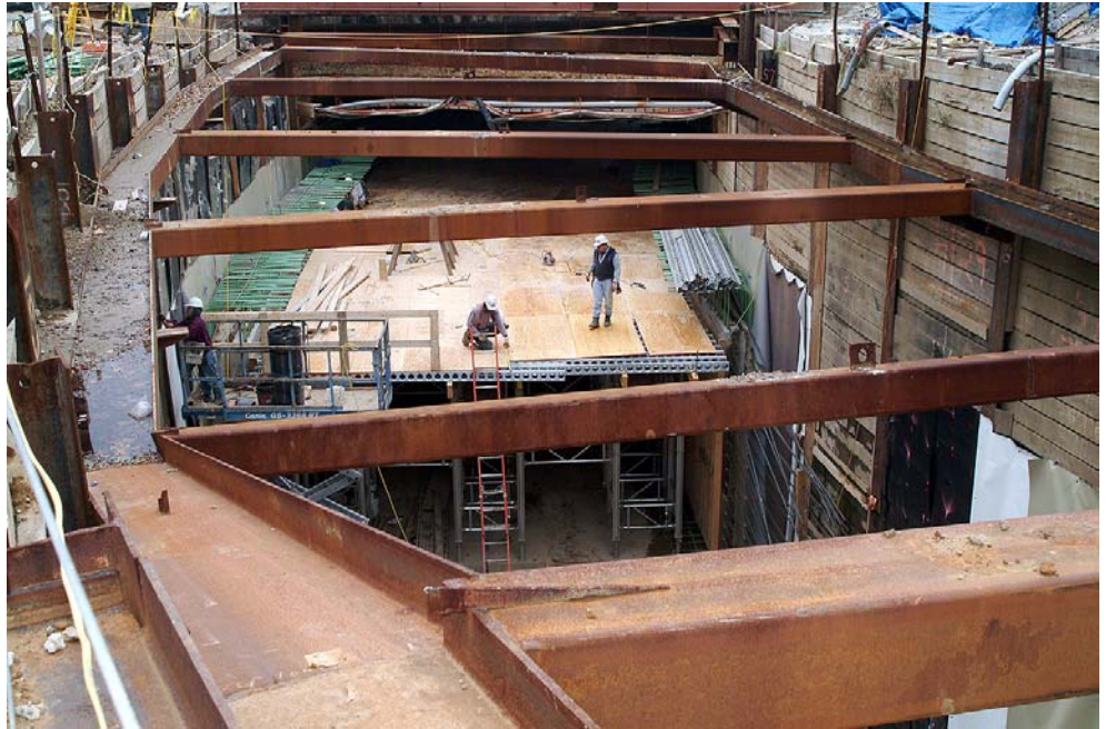
A crew working on the new truck tunnel builds the formwork for the roof of the tunnel in preparation of a concrete pour. Eventually, the area above the tunnel roof will be backfilled.
