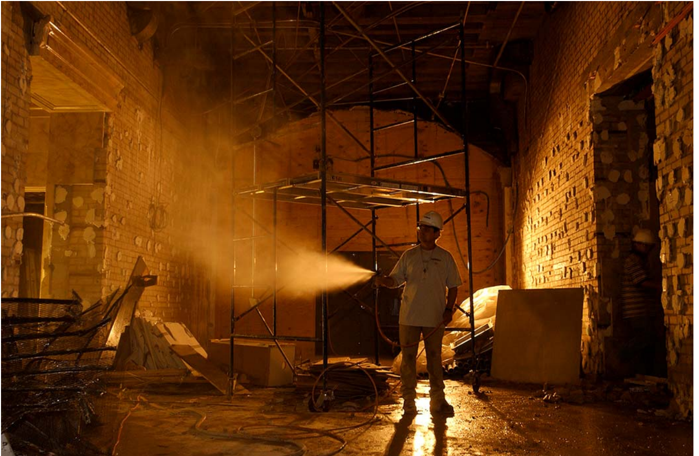
Within the East Front Extension, in an area just east of the Crypt that formerly housed the Capitol Historical Society gift shop, a worker uses a water hose to control dust in preparation for additional demolition that will occur in this zone.
