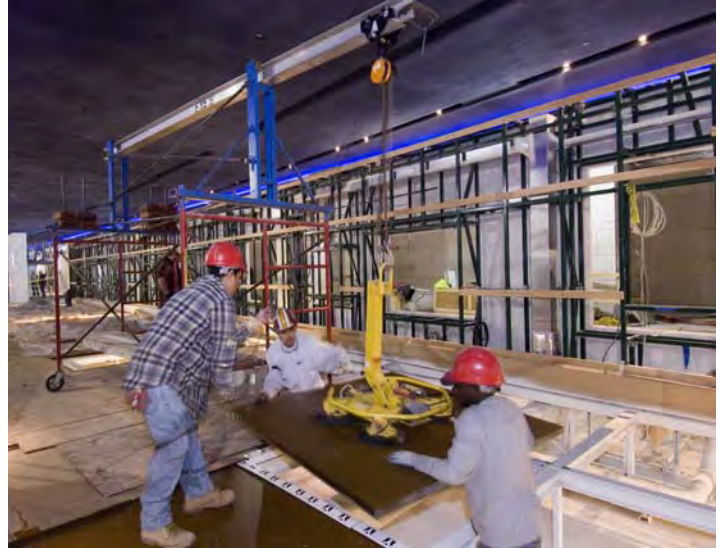
Workers set a glass floor panel on a steel grid inside the CVC Exhibition Hall. The panels will be illuminated from below, providing a soft glow around the central Wall of Aspirations.
