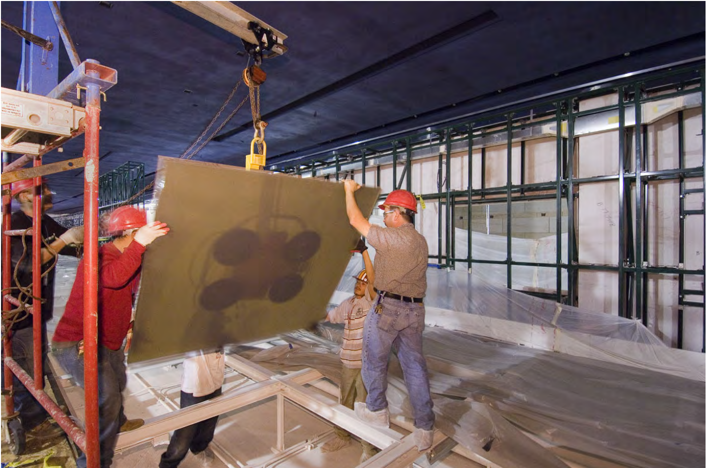
With the aid of an electronic suction machine, workers set a 500-pound glass floor panel to a steel support grid in the CVC's Exhibition Hall.
