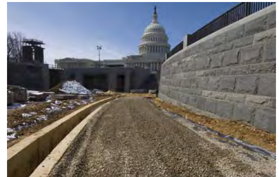
A gravel bed has been placed along the north entrance ramp in preparation for the placement of an aggregate concrete sidewalk that will look and feel like the sidewalks throughout the Capitol campus.
