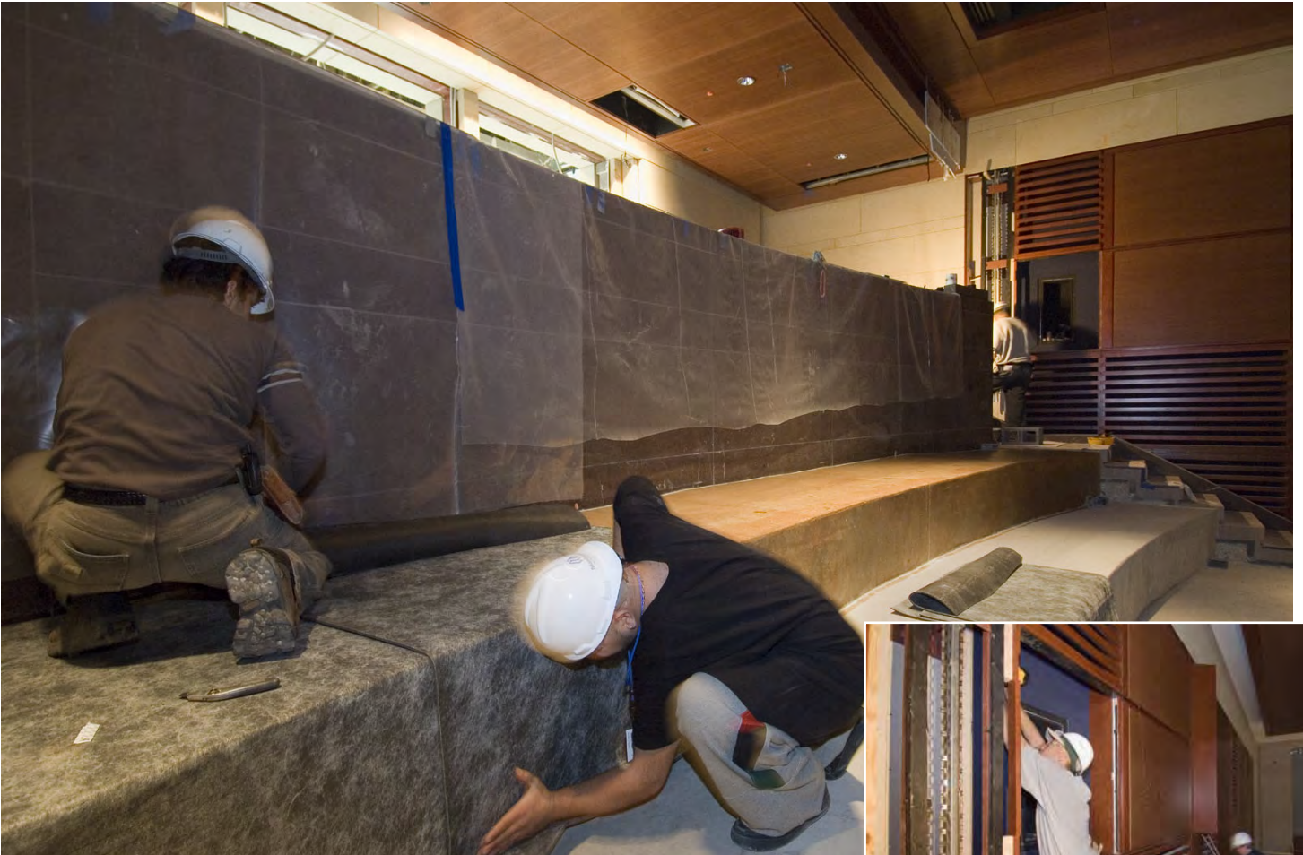
Inside the North Orientation Theater, carpet installers lay padding for carpeting on the uppermost seat tier marking the first carpet installation to occur anywhere in the CVC. Carpet installation is expected to be completed in both the North and South Theaters early in February. Inset: Workers continue to install wood and fabric wall panels in both theaters.
