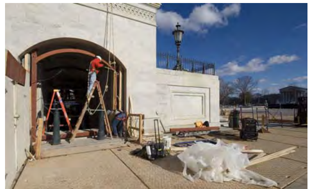
Workers assemble some of the steel support structure for one of two glass walls that will enclose the central carriageway below the East Front Center Steps. The walls will help secure the transition zone that connects the CVC and the Capitol while allowing natural light to illuminate the central stair and escalators.
