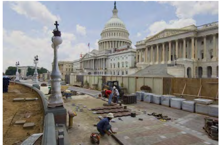
Just east of the Senate wing, masons set pavers in a decorative pattern inspired by a Frederick Law Olmsted-designed pattern that was identified by the project design team in photographs taken in the 1890s.
