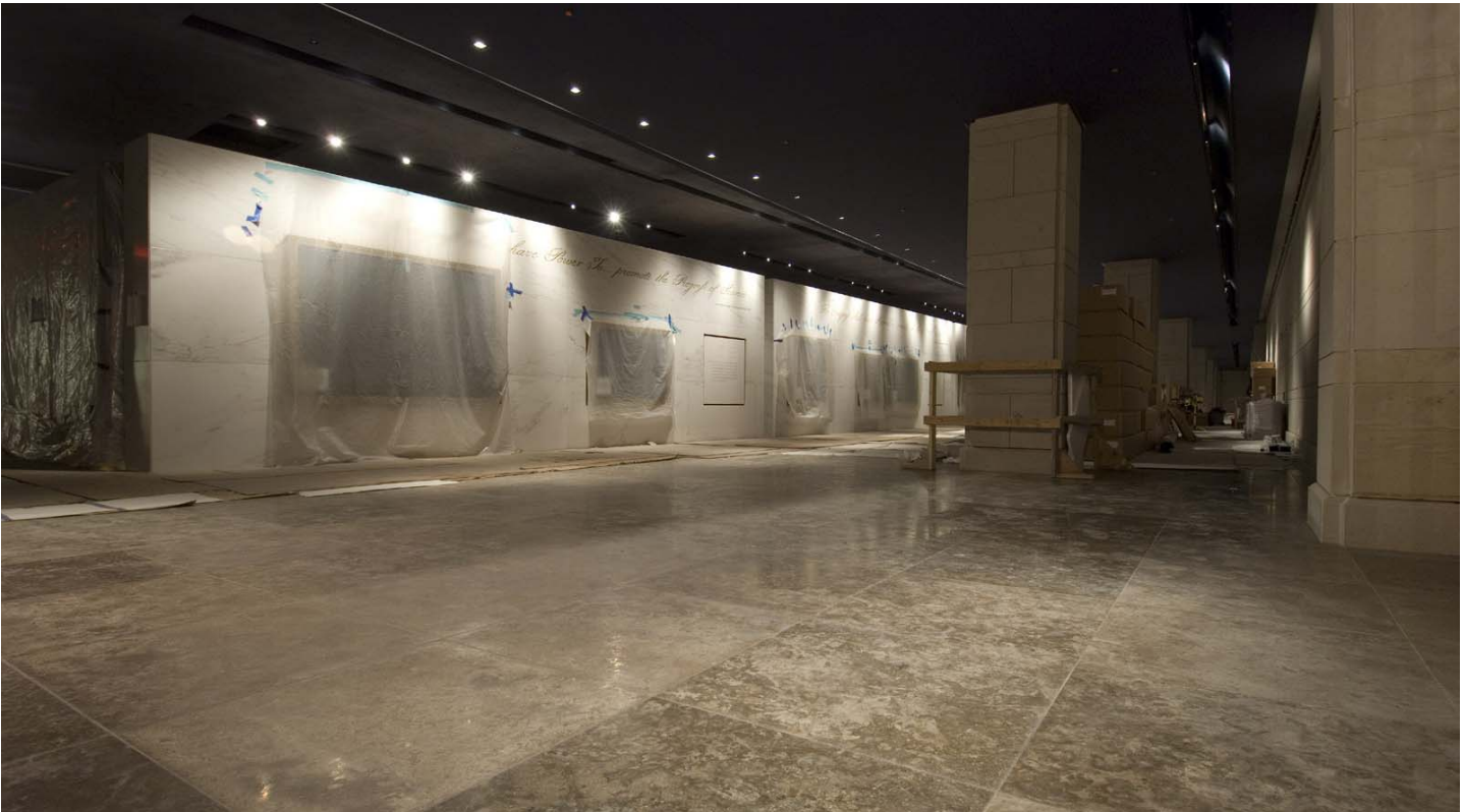
Inside the CVC's Exhibition Hall, workers have removed much of the protective covering from the floor stone as the area nears completion.
