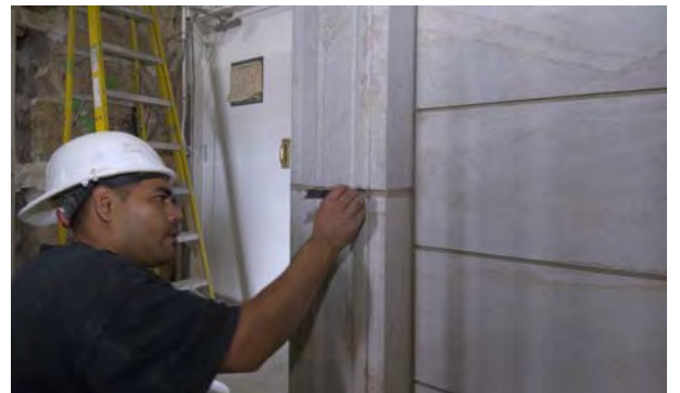
In the East Front of the Capitol, a mason applies grout between two stones that line the threshold of the Rotunda Door.
