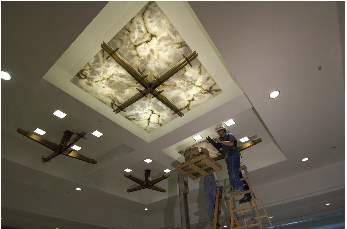
A worker installs translucent alabaster stone panels that will diffuse the ceiling lights in a lobby area near the CVC's Orientation Theaters.
