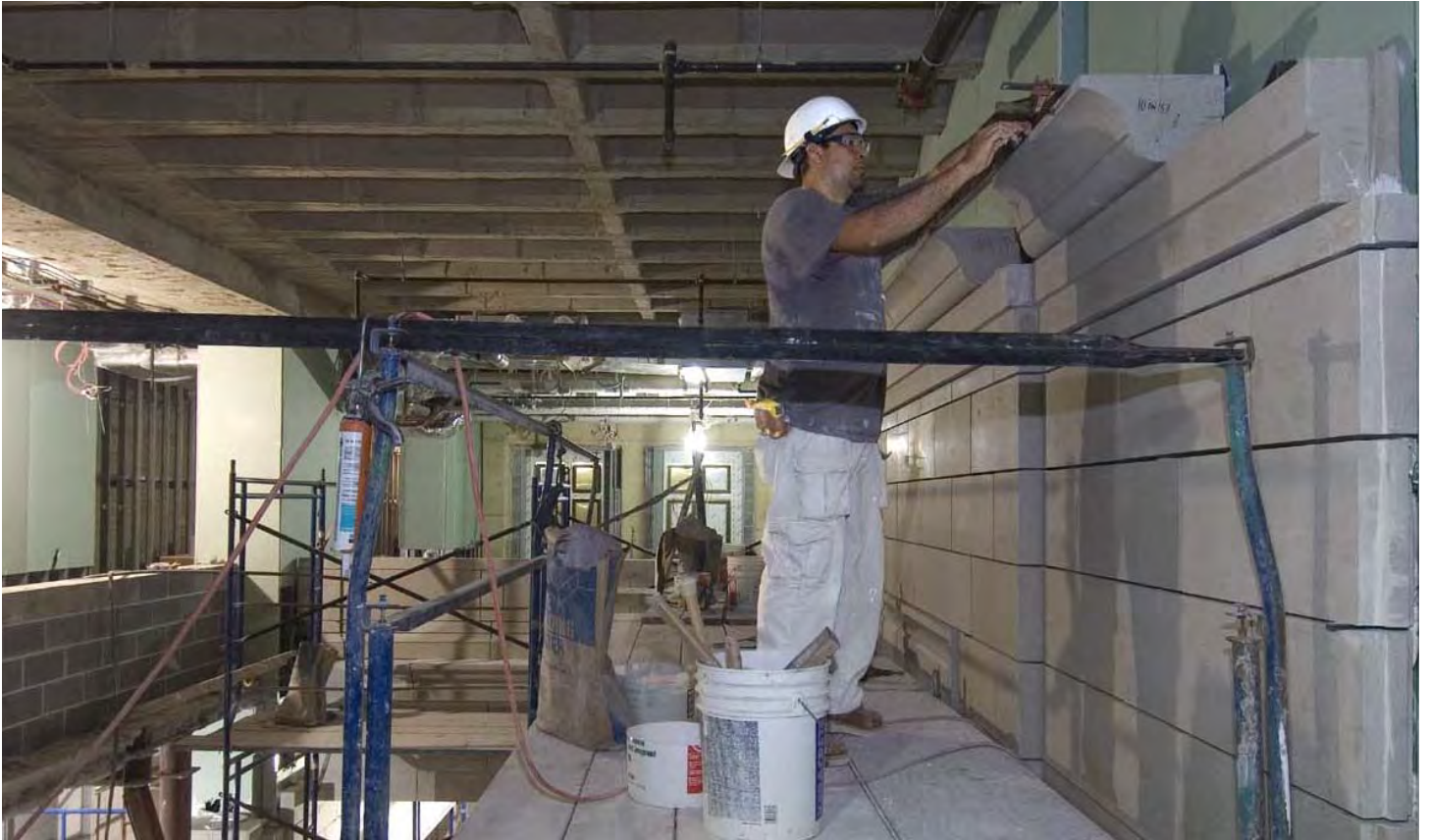
A mason installs a decorative piece of sandstone near the ceiling of the third floor (Gallery level) within the East Front of the Capitol. Nearly 4,700 pieces of stone will line the interior walls of the East Front. The doors for two 25-passenger elevators can be seen at the far end of the scaffold.
