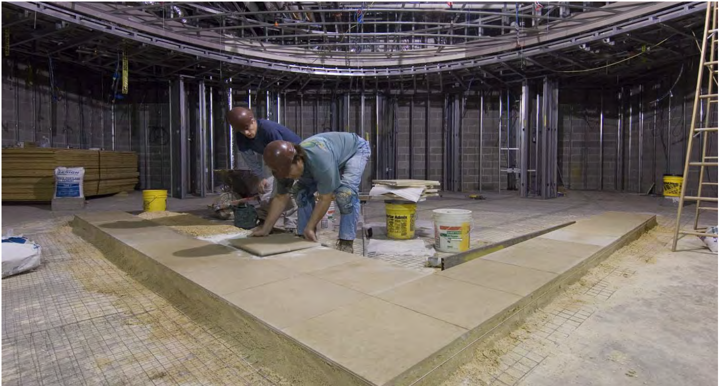
Masons set floor stone in one of the CVC's two gift shops, which are located on the visitor out-flow corridors on the upper level.
