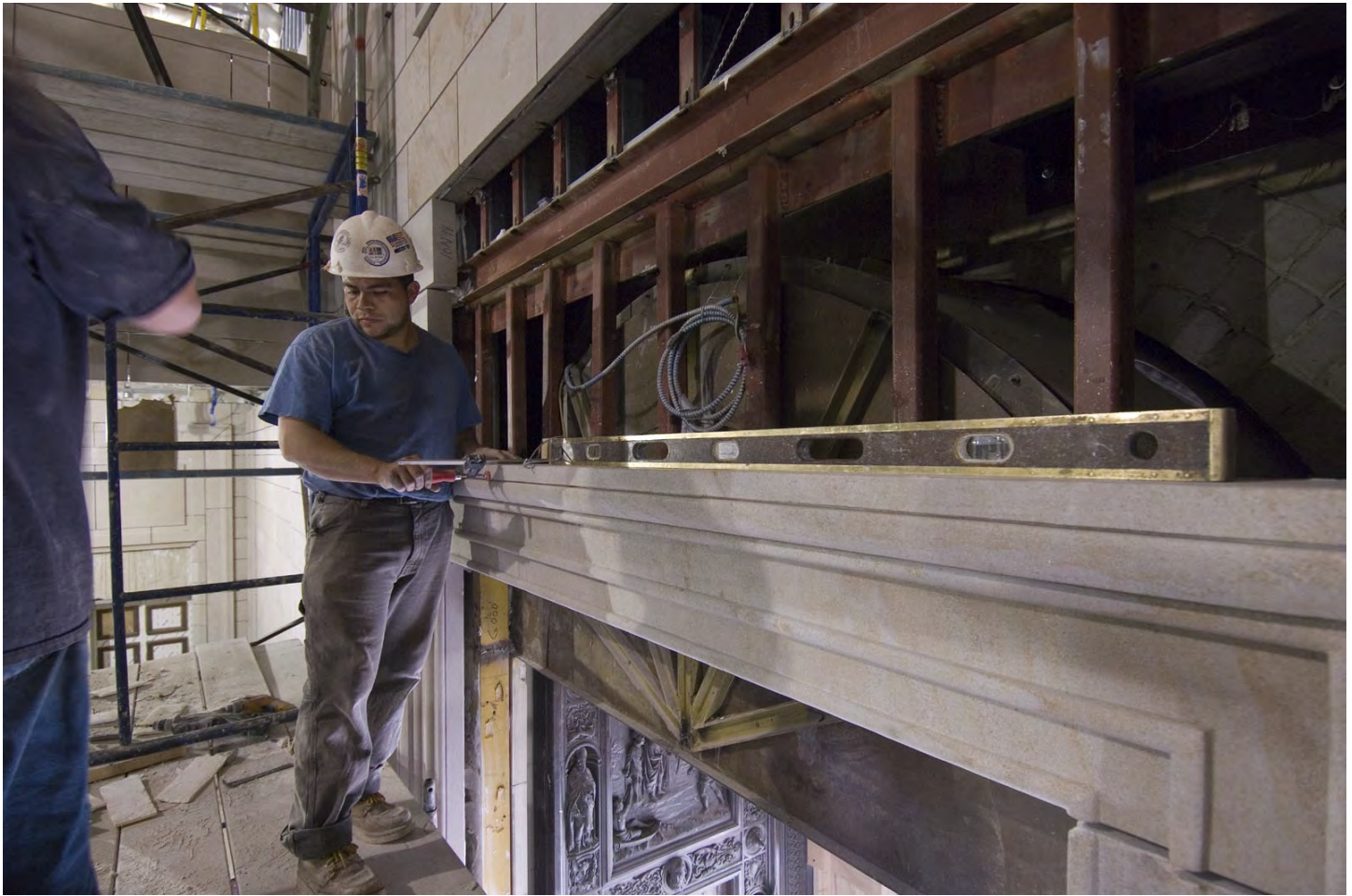
A mason checks the level of a stone threshold piece above the exterior bronze Rotunda Doors. Wall stone installation in the East Front is progressing well and is nearing completion at both the Rotunda and Gallery levels.
