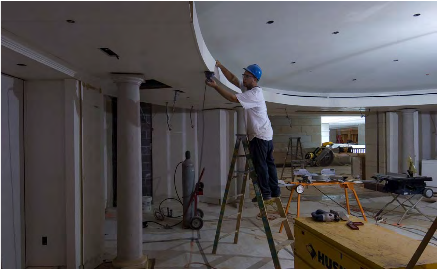
A carpenter uses a sander to finish the ceiling trim in the south side CVC Gift Shop. A similar shop is located on the north side of the facility.
