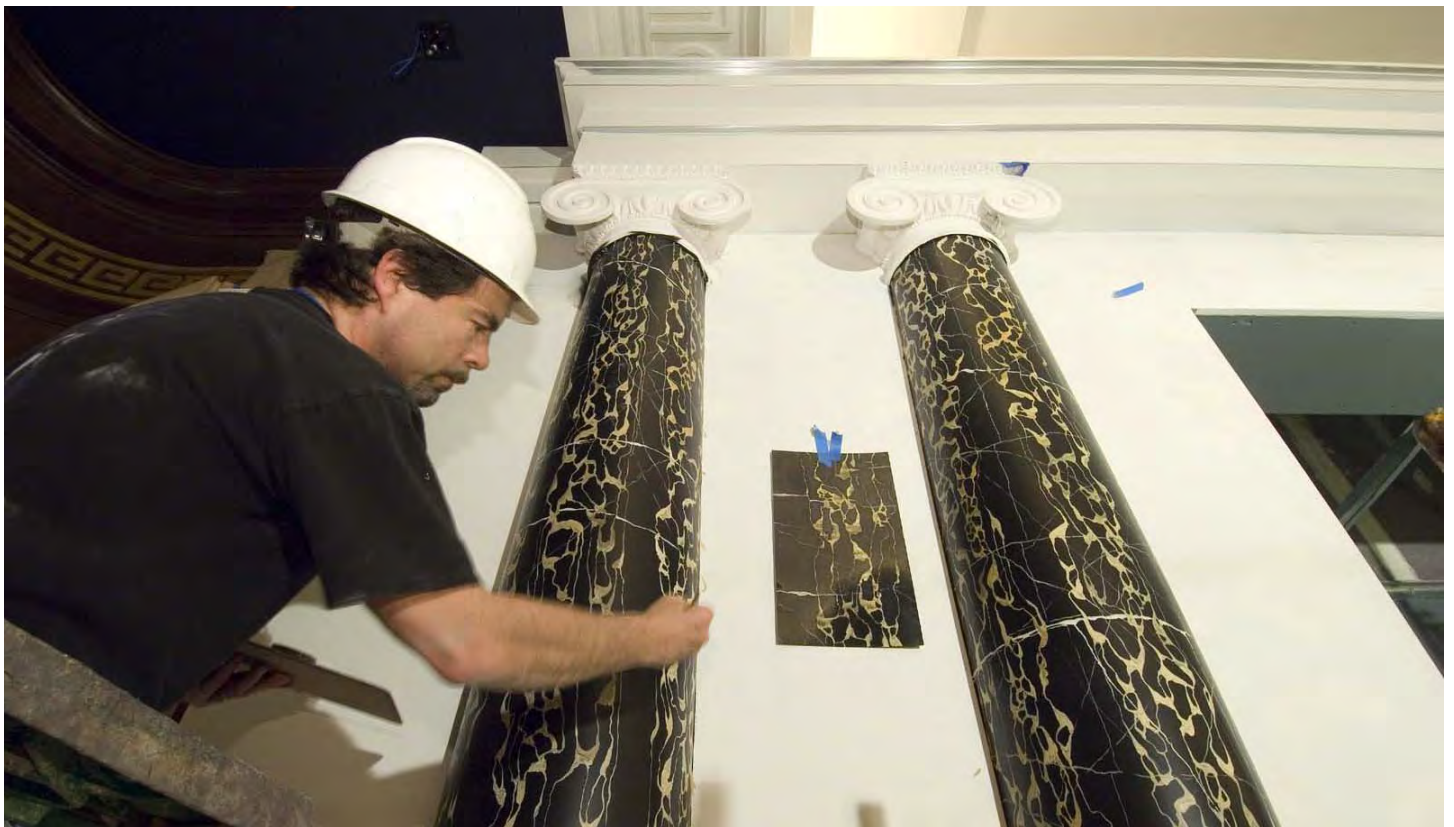
Inside the CVC Exhibition Hall, a painter applies a faux marble finish to columns inside the Virtual House Theater.
