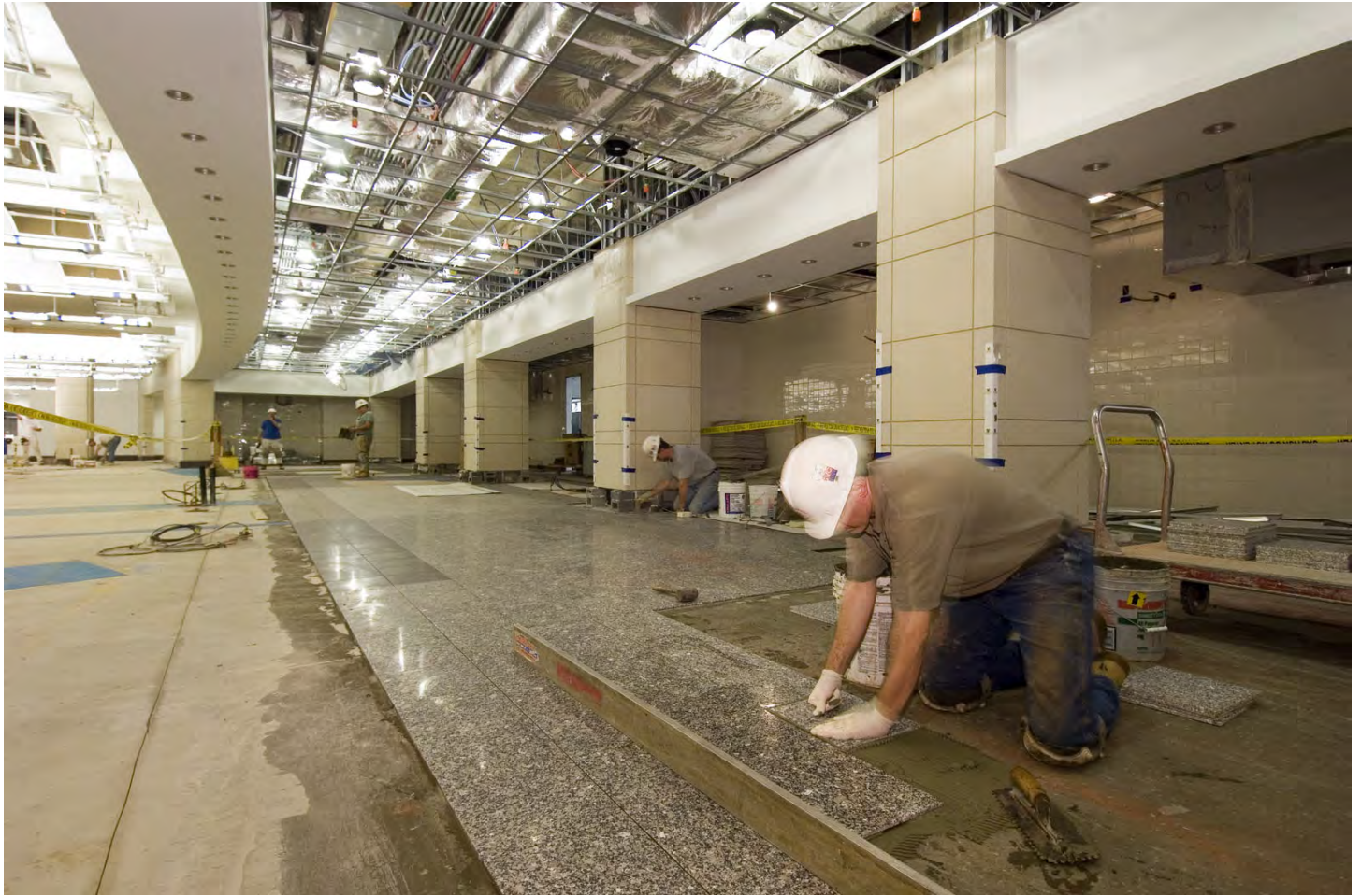
A stone mason lays tile in the Food Service servery area. More than 500 people can be seated in the Food Service Area at one time.
