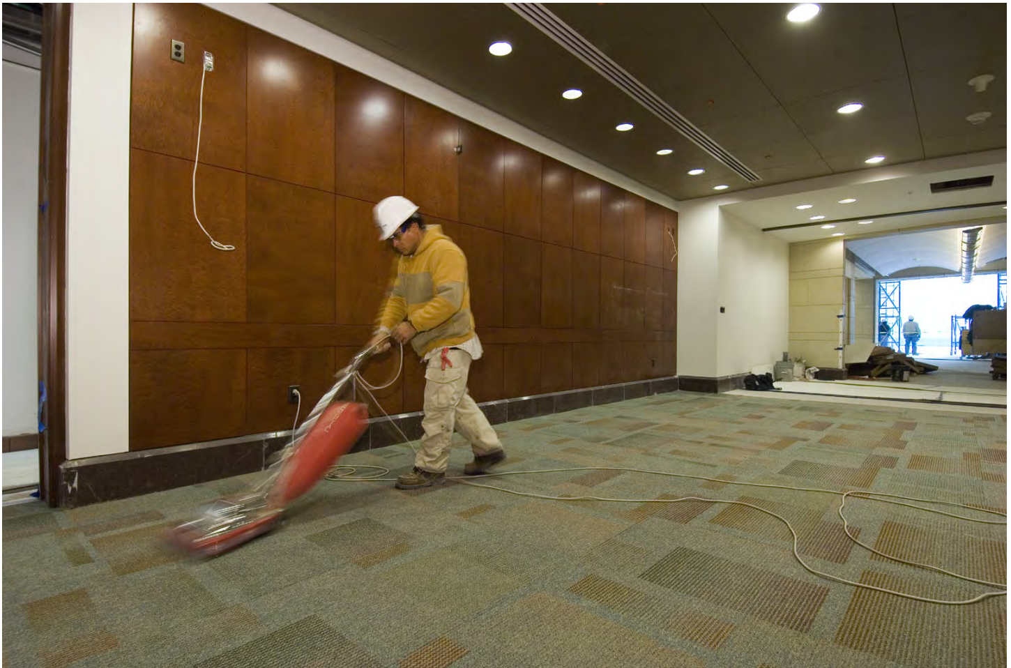
A worker vacuums newly laid carpeting in one of the Food Service seating areas. Tile work surrounding these areas will be completed in February.
