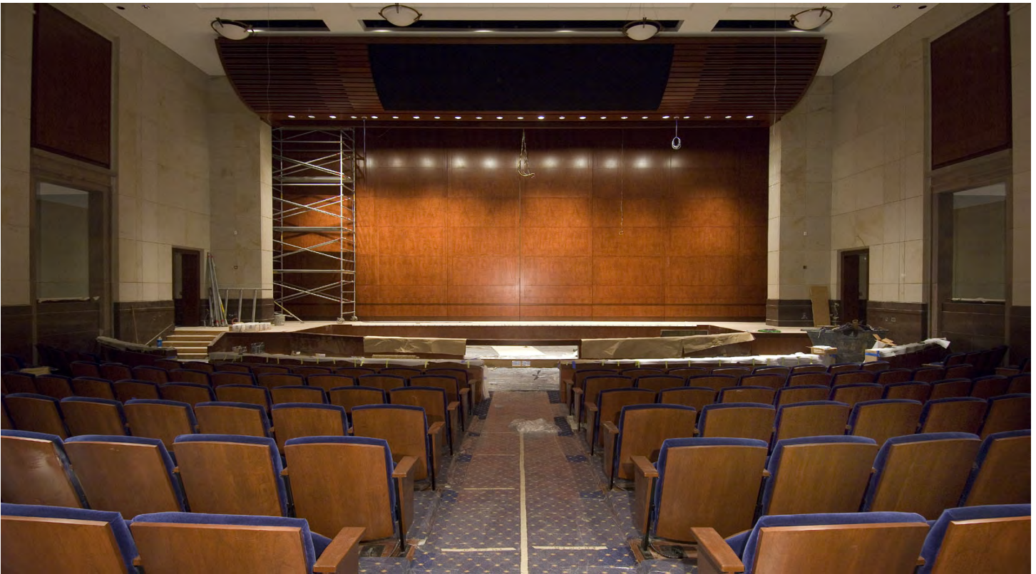
Installation of wall stone, seating, carpet, millwork and light fixture installation are nearly complete in the Congressional Auditorium.
