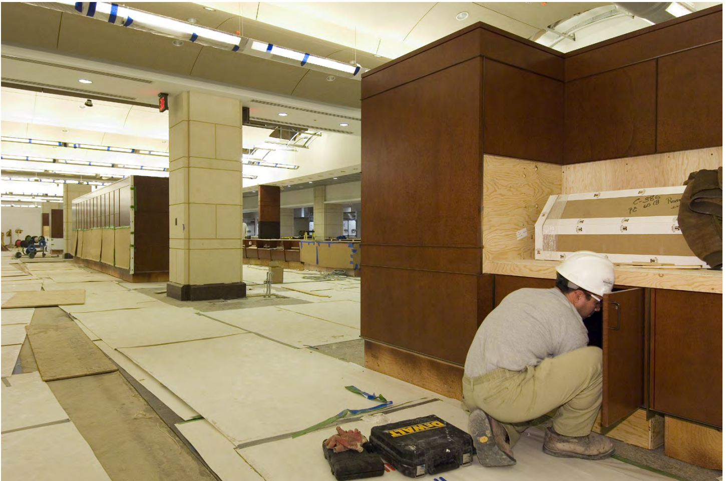
In the CVC's Food Service Area, a carpenter installs cabinetry components in the food servery area. The primary seating area is at left.
