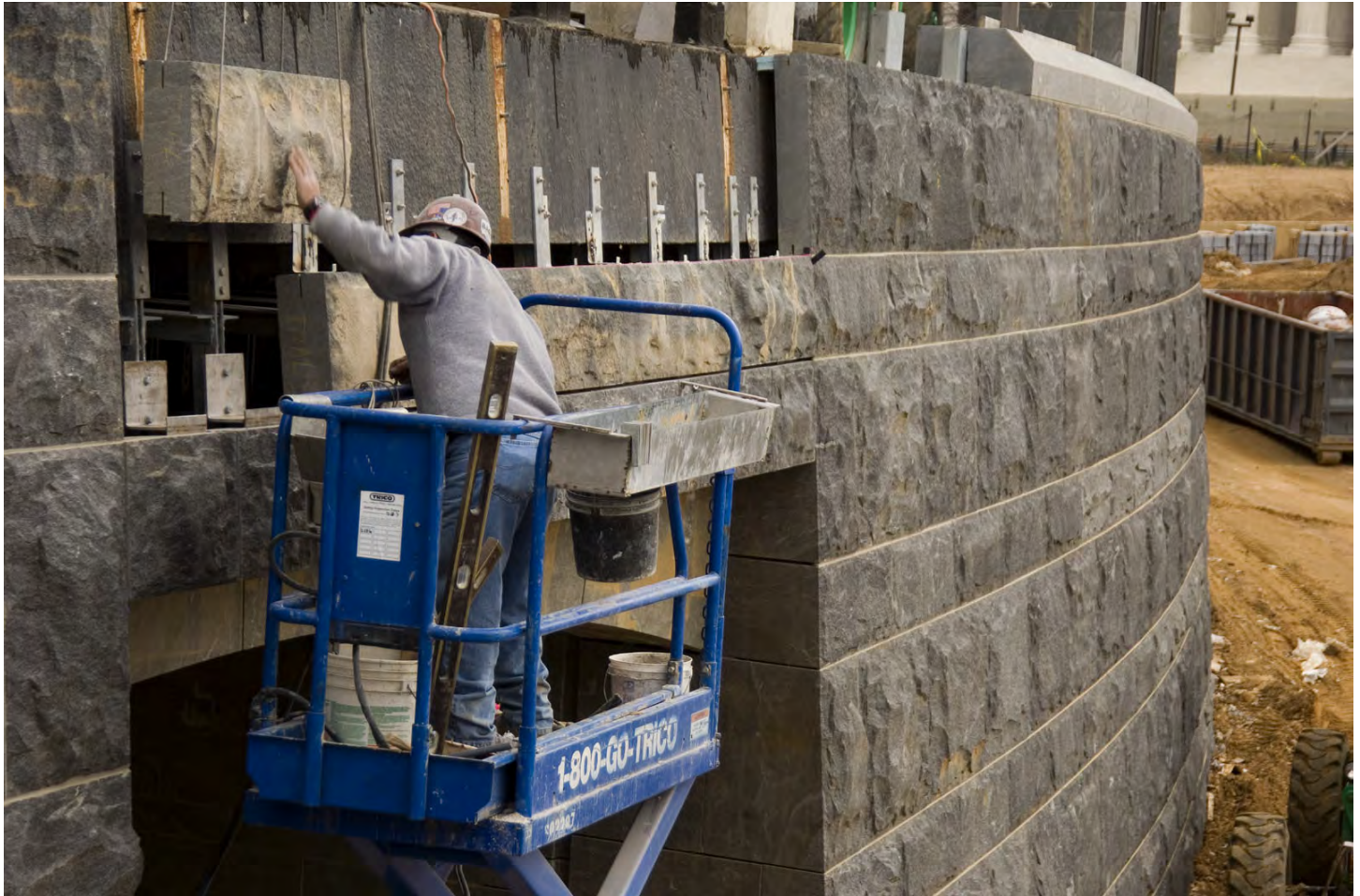
A stone mason sets a block of gray granite from a quarry in Culpeper, VA, to the retaining wall along the CVC's north entrance ramp.
