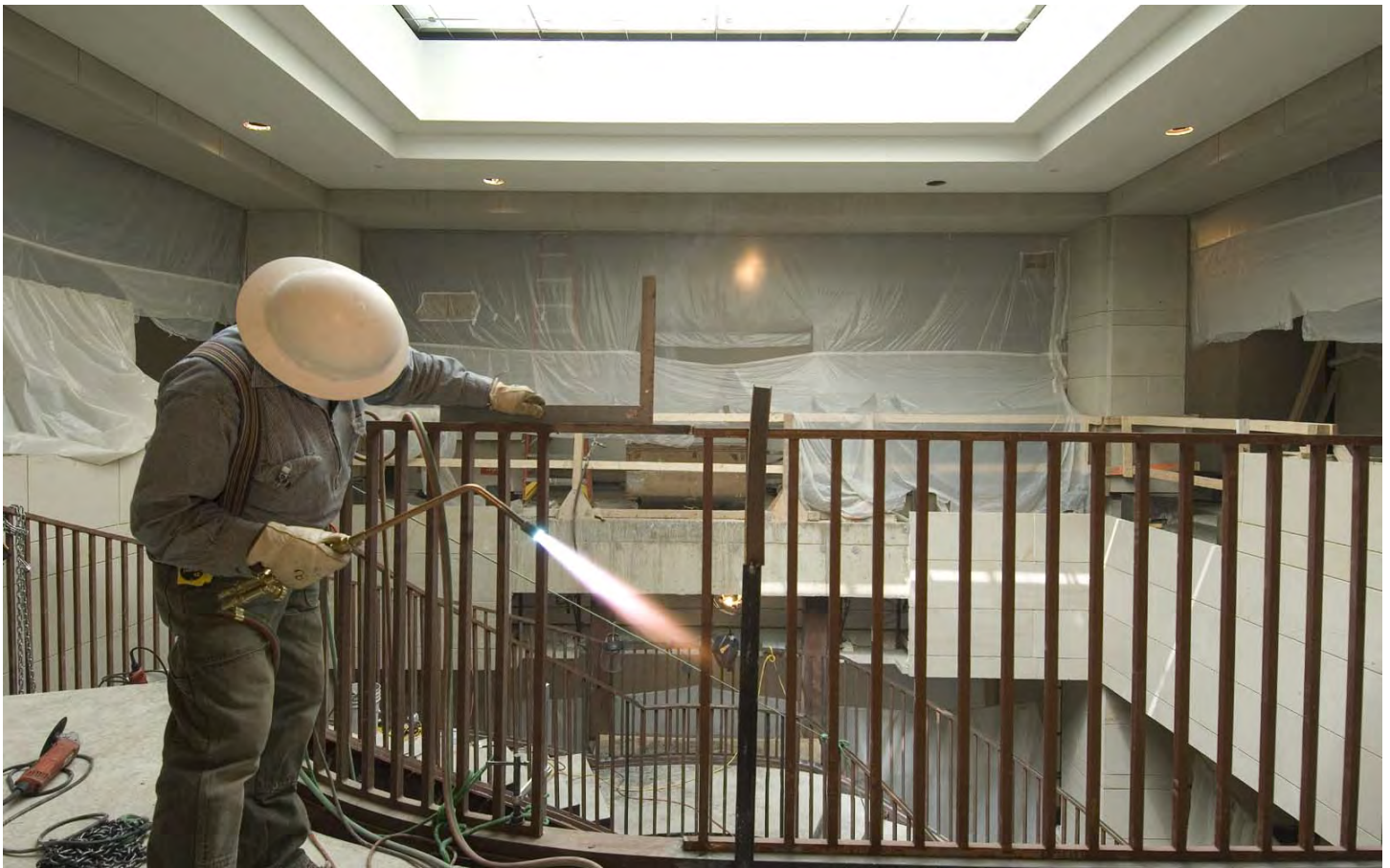
A welder secures two pieces of metal railing for a spiral staircase in the Senate Expansion Space. A skylight illuminates the atrium.
