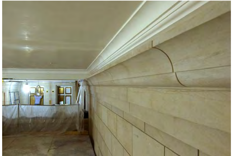
At the Gallery Level (third floor) of the East Front of the Capitol, ceiling work is nearly complete. Stone work in this area was completed this fall.
