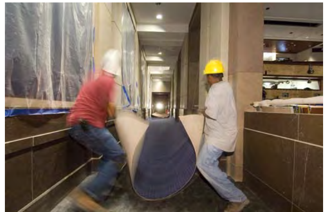
Workers lay decorative blue carpet in the north corridor inside the Congressional Auditorium.
