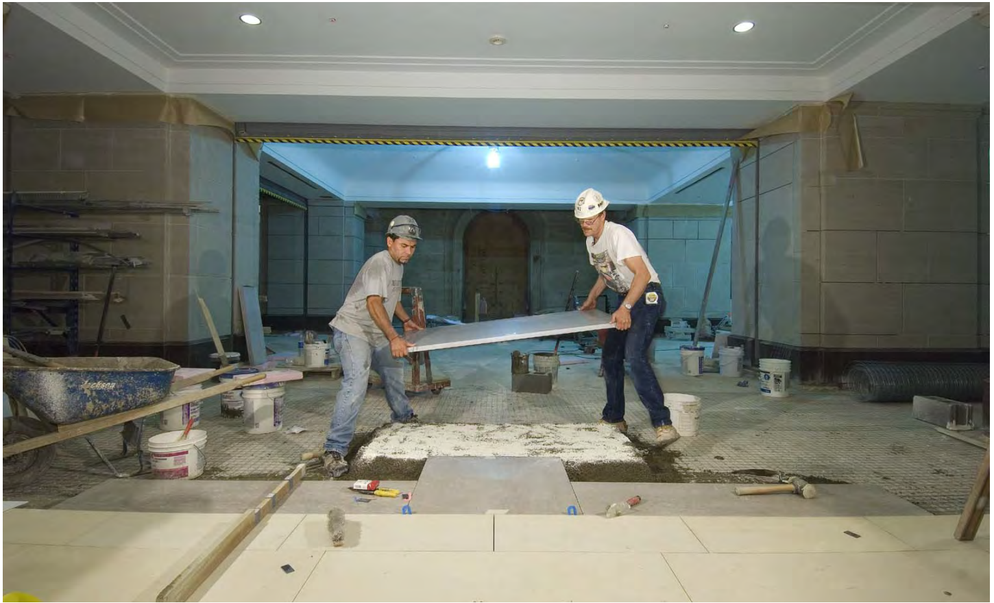
Masons set a piece of marble floor stone at the Crypt Level inside the East Front of the Capitol in an area just west of the main staircase and two escalators that connect the CVC to the Capitol. Up to 15,000 visitors a day will walk through this area to enter and leave the Capitol.
