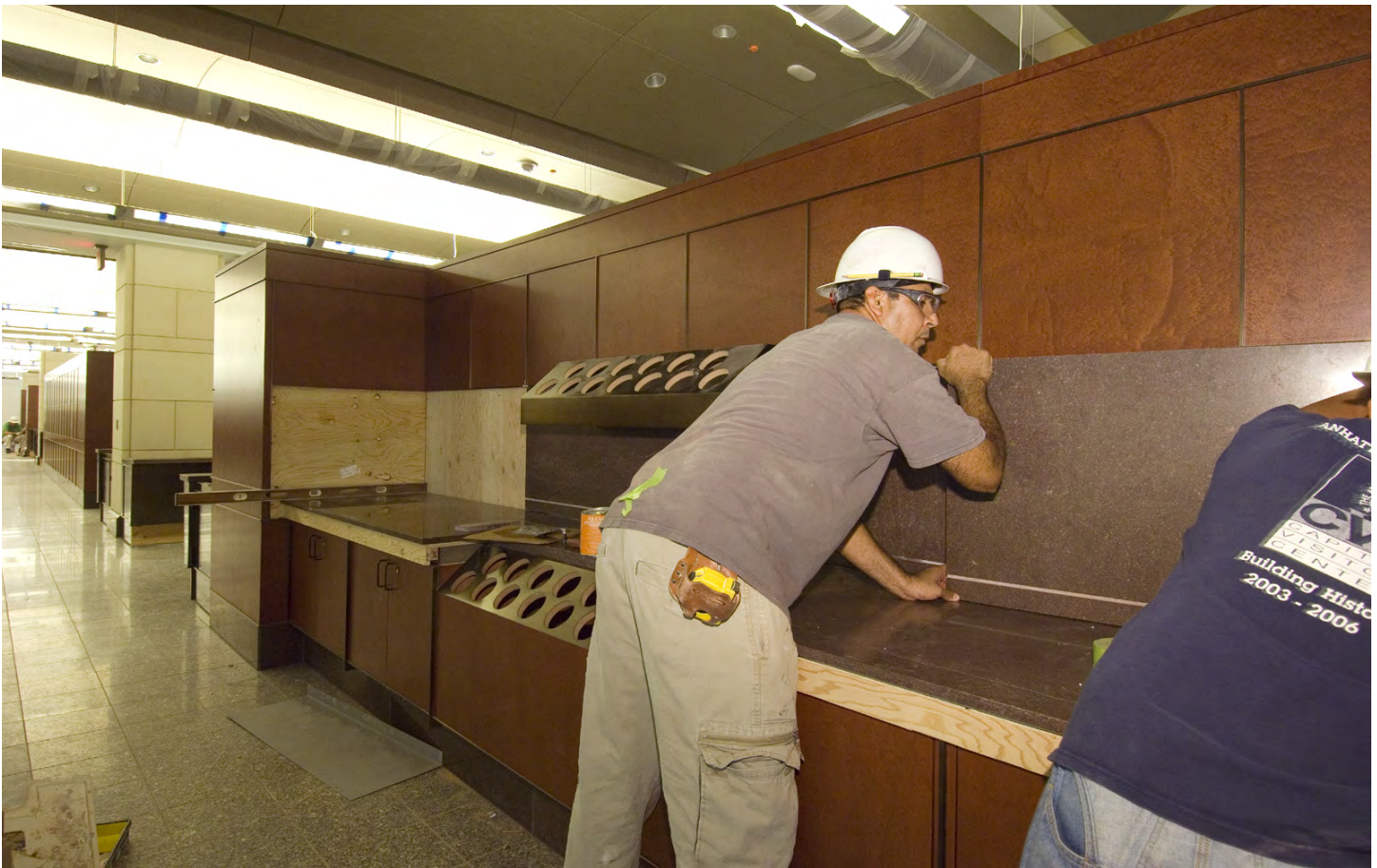
Masons install marble countertops to some of the cabinetry components inside the CVC restaurant.
