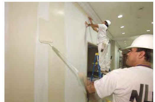
Paint crews are busy applying the final coats of paint to interior spaces throughout the CVC.
