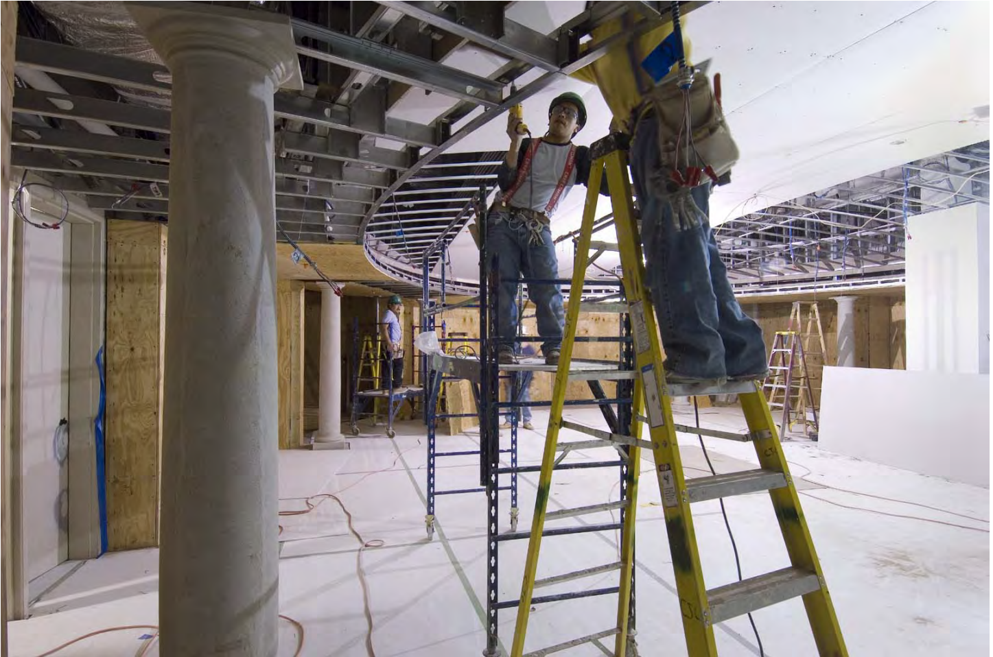
Workers secure drywall to the ceiling grid inside one of the CVC's two gift shops. Sandstone columns line the perimeter of the space.
