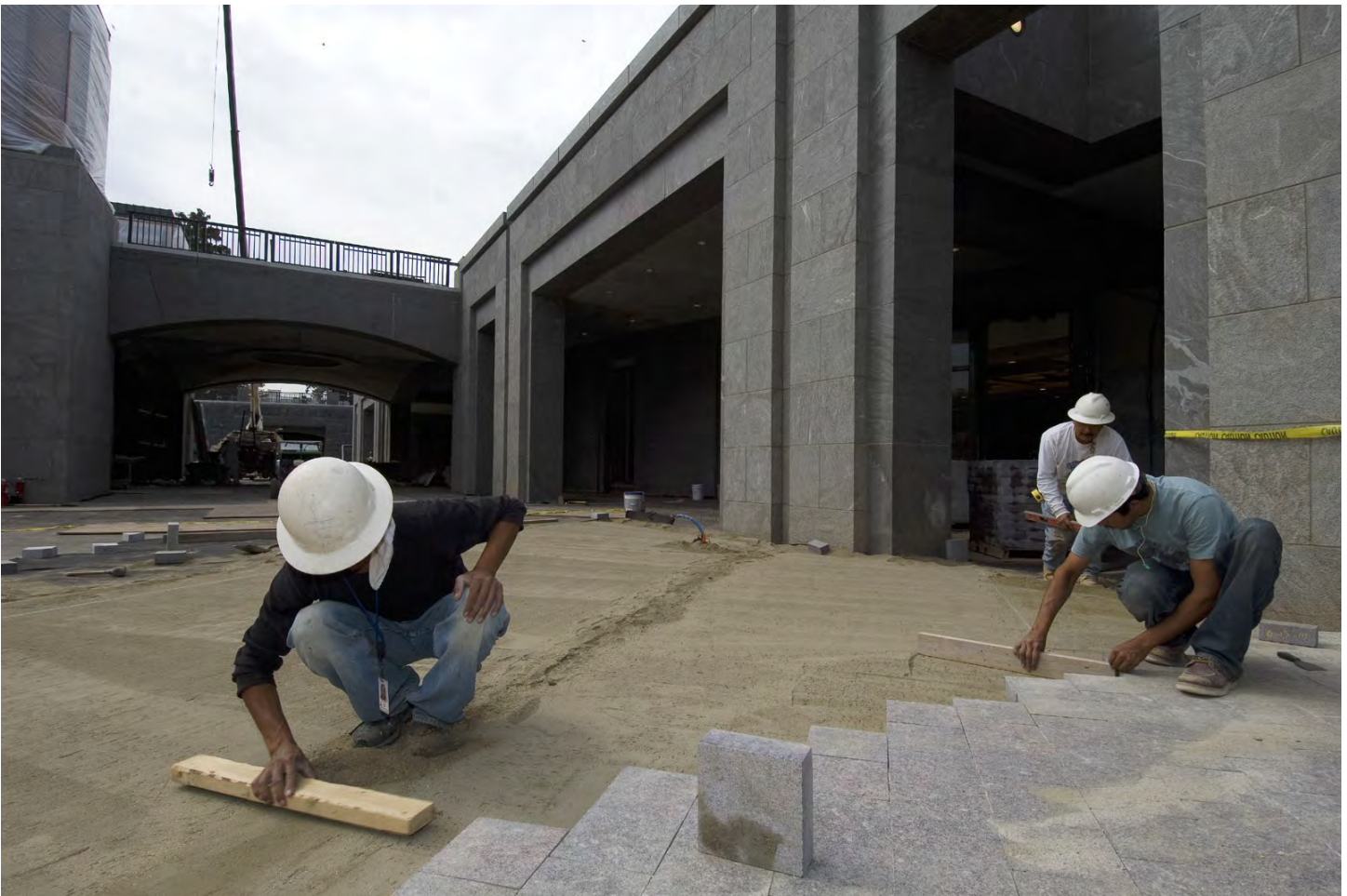
Masons lay granite paving stones on the lower plaza near the CVC's north entrance zone. The work will progress southward through October.
