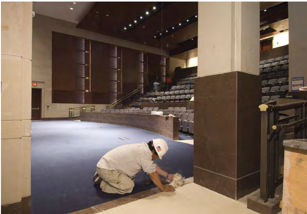
A worker removes some protective material from floor stone near the entrance to the CVC's South Orientation Theater in an effort to prepare the space for the subsequent inspections. Professional cleaning crews are at work in both theaters and in most interior spaces dusting millwork, buffing floor stone, vacuuming carpets, and polishing bronze and stainless steel elements to clear the way for the final testing of the CVC's fire and life-safety systems. That process will begin on November 16 th marking a significant milestone for the project as all major construction work is now complete.
