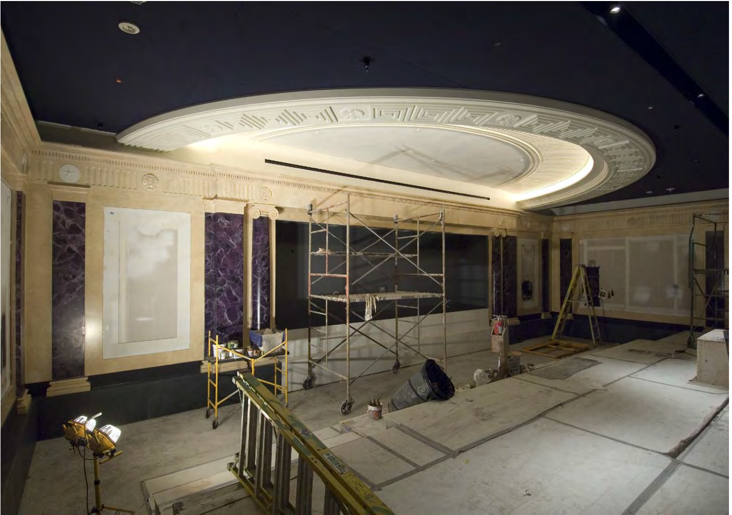
The faux marble painting is complete on the decorative columns and plaster elements in the Virtual Senate Theater in the CVC Exhibition Hall.
