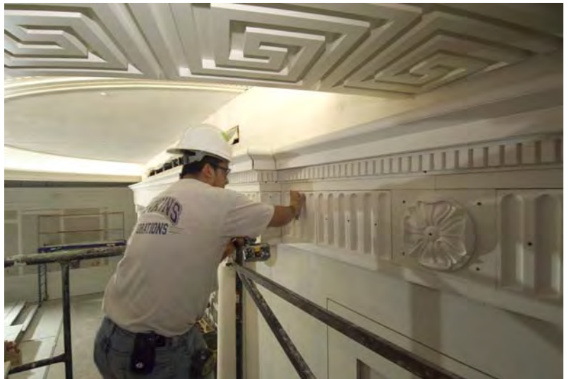
In the CVC Exhibition Hall, a worker installs a pre-fabricated plaster panel to a wall inside the Virtual Senate Theater. The decorative ceiling and wall panels are intended to mimic the architectural elements in the Senate Chamber.
