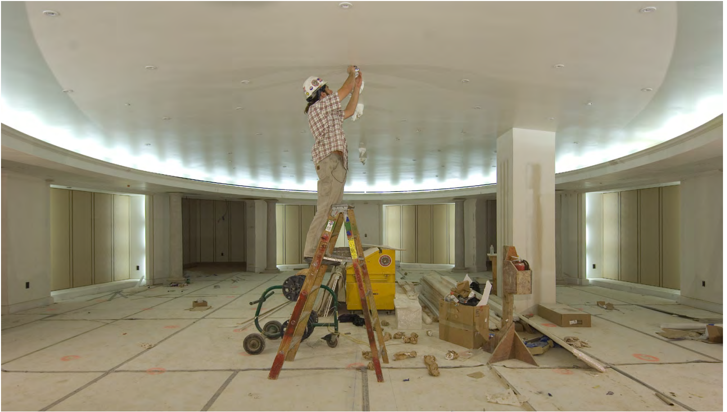
An electrician installs a fire alarm device in the ceiling of one of two CVC gift shops, which are located to the north and south of the Great Hall.
