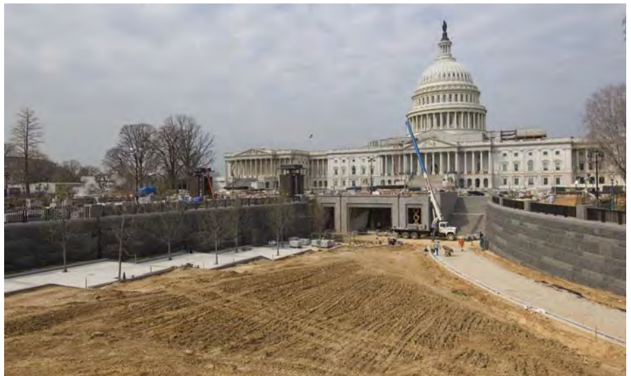
The CVC entrance zones are now being cleared and graded to make way for final sidewalk work, landscaping, installation of lampposts and other restoration activities, which will occur into the summer. As can be seen in this photo, the gently sloping approaches to the CVC entrances preserve the sense of procession to the Capitol.
