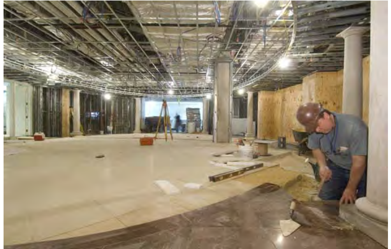
A mason continues setting stone in one of two CVC gift shops.
