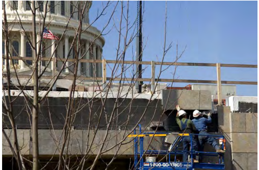
Masons are nearly complete with stonework at the face of the CVC entrance zone.
