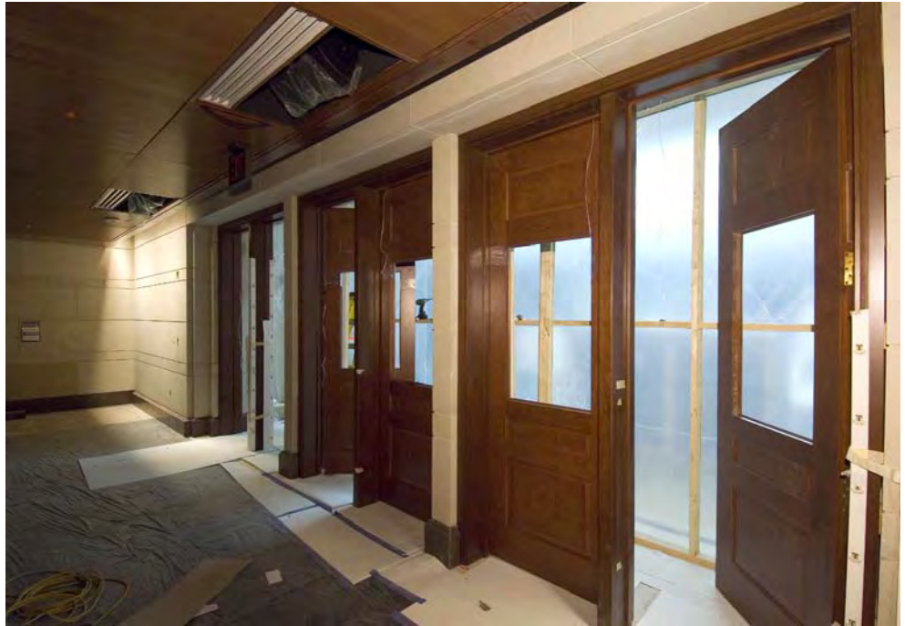
Wood doors have been installed at the top of the North and South Orientation Theaters.
