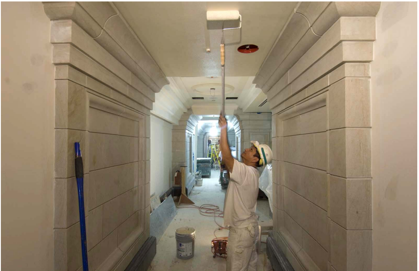
A painter applies a base coat of paint to the recently-completed plaster ceiling of the third floor (Gallery level) in the East Front of the Capitol.
