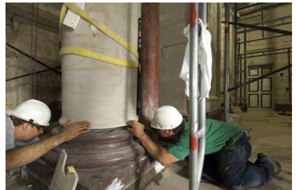
Masons set a sandstone column on the Rotunda level of the East Front of the Capitol.
