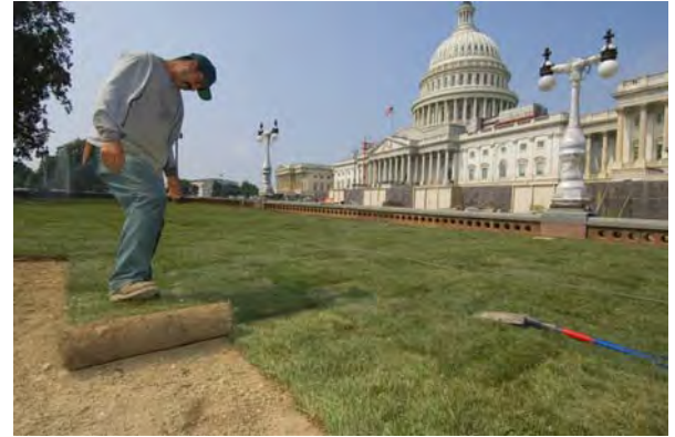
Landscape crews have been placing sod within the Senate Egg to restore the large grassy oval located east of the Senate wing to its pre-construction state.
