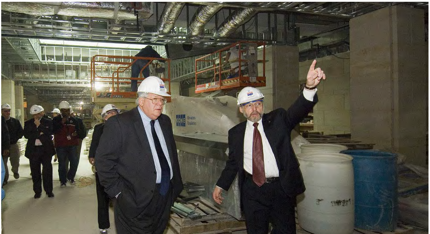
Architect of the Capitol, Alan Hantman (right) points out some CVC ceiling details to Speaker of the House, Dennis Hastert , during a recent site walk.
