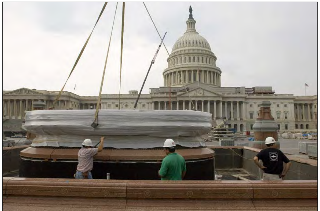
Last week, the historic Olmsted bronze fountain basins were installed on the East Front Plaza.
