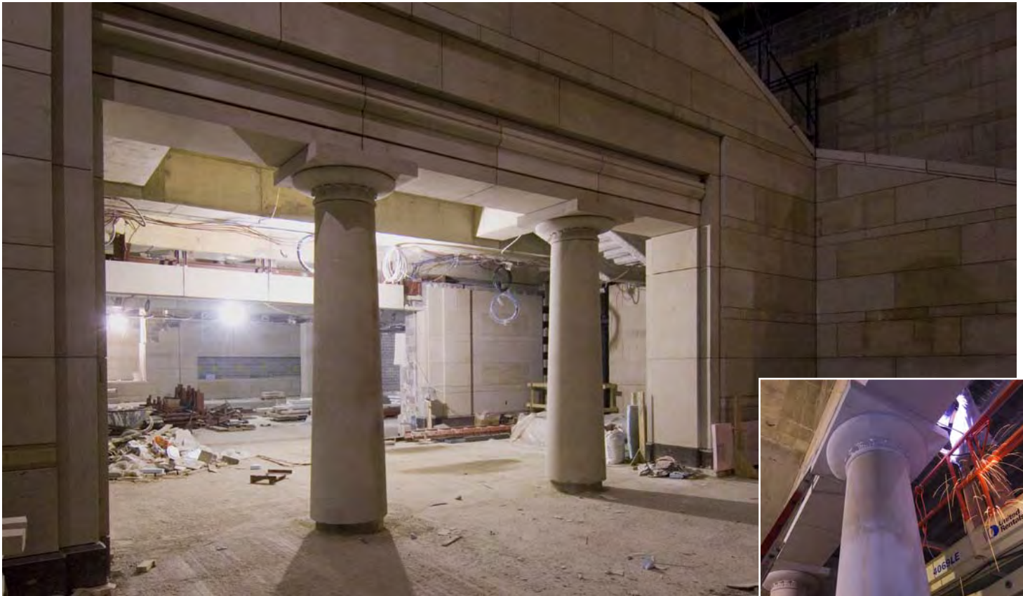
Above: Two sandstone columns, similar to the columns in the Crypt of the Capitol, now mark the entrance to the CVC Exhibition Hall. Inset: A worker welds steel support beams that will support sandstone slabs above the entrance threshold.
