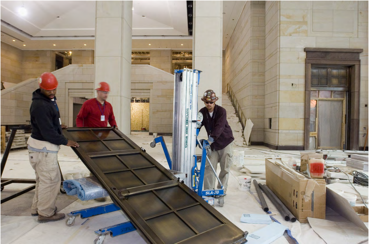
A crew raises one of the two bronze doors for the North Orientation Theater visitor entrance. The entrance threshold is framed with burgundy sandstone (right of photo) to match similar stone work around both of the north and south entrances of the Capitol Rotunda.
