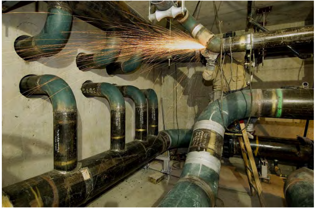
Utility connections are nearing completion in the East Capitol Street Utility Tunnel.
