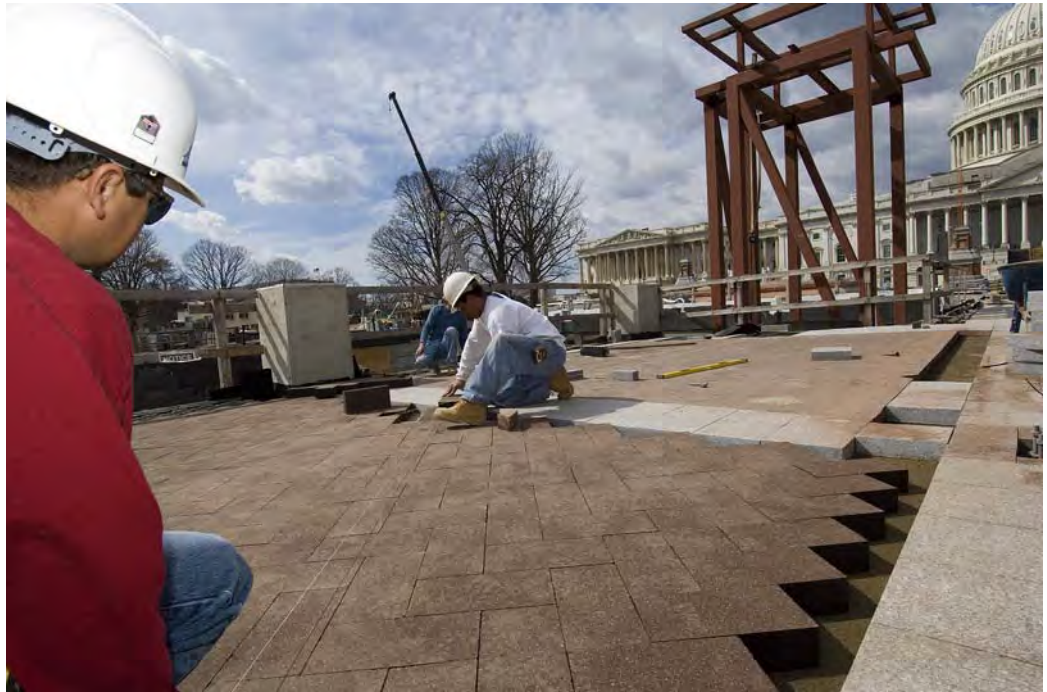
On the East Front Plaza, masons have begun setting granite pavers in a herringbone pattern along the curving walkway that lines the Senate egg. The steel framework for one of two new elevators can be seen in the background. Eventually, red and gray granite stone will ornament the elevator tower.
