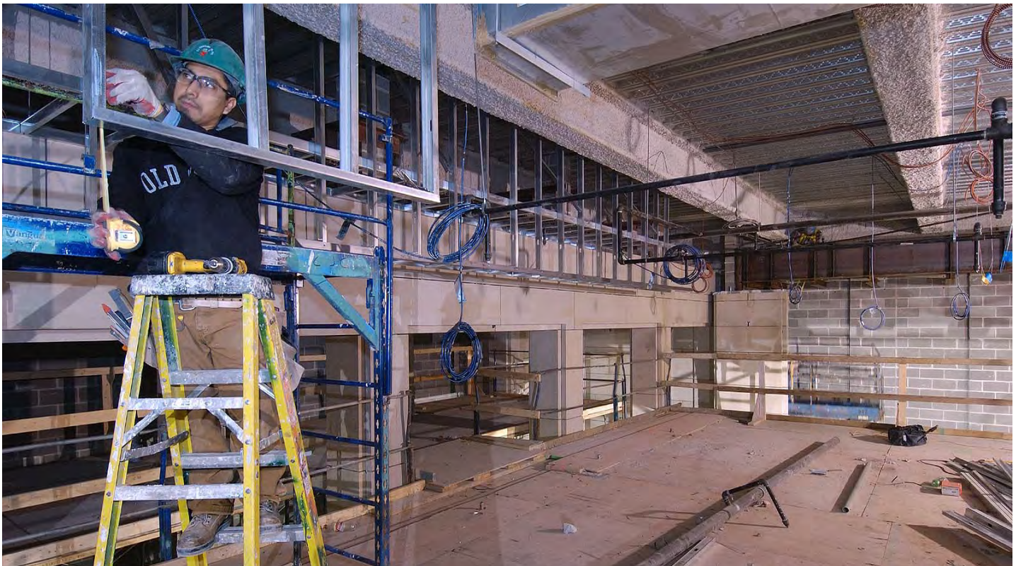
A worker assembles a metal stud support for the ceiling in the South Orientation Theater. The stone work is now complete in both theaters.
