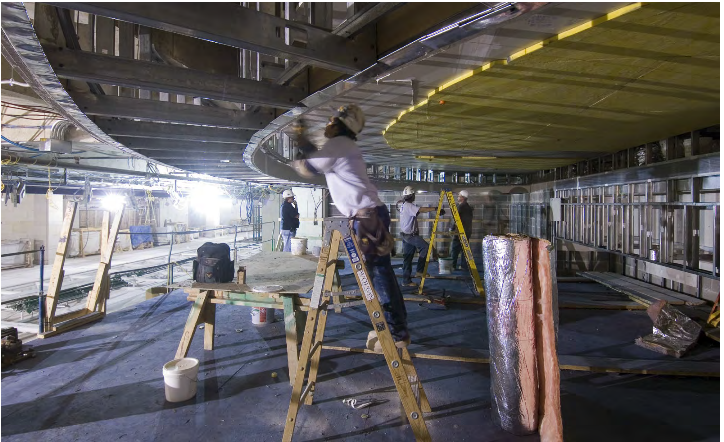
In the CVC's 16,500-square-foot Exhibition Hall, a worker continues ceiling panel installation in the Virtual Senate Theater.
