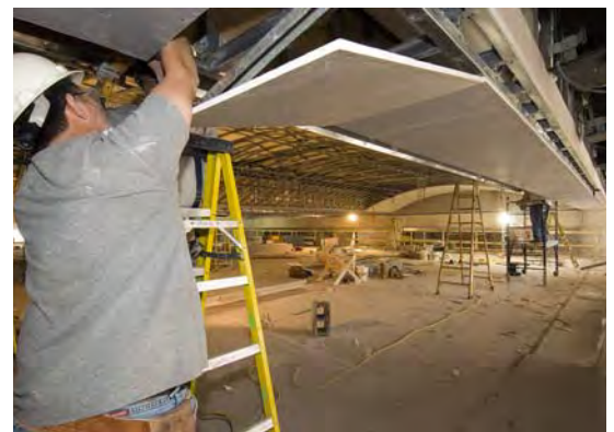
Drywall installation has begun on the ceiling in the Great Hall. A plaster finish will be applied later.
