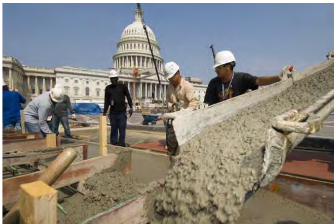
A CVC crew prepares a concrete foundation for the historic seat wall around the large grassy oval on the south side of the Plaza.
