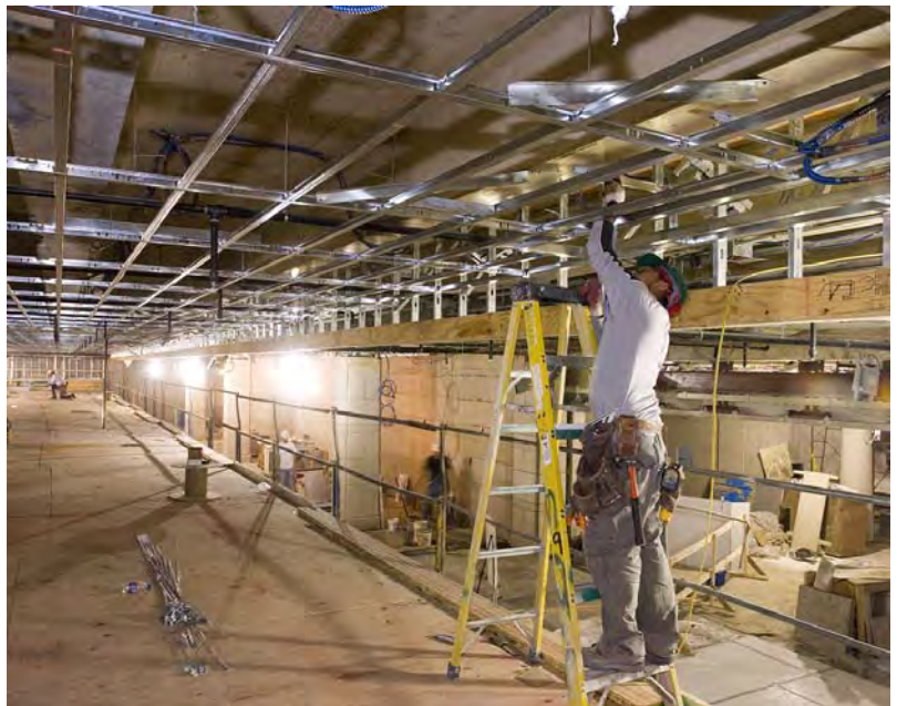
A worker assembles a portion of the ceiling framework above the Exhibition Hall.
