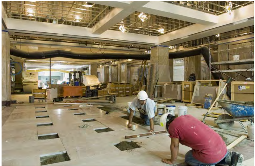
Masons set floor stone in the lobby area just outside of the CVC's two Orientation Theaters.
