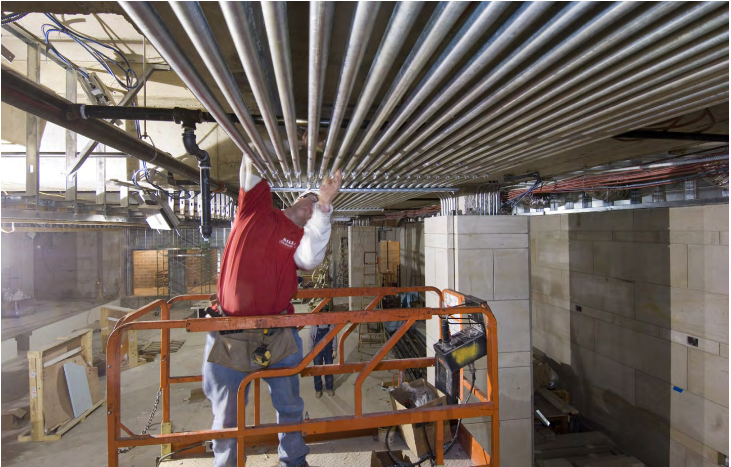
A worker installs telecommunications conduit in the ceiling of the CVC Exhibition Hall. The lines will connect House and Senate Expansion space.
