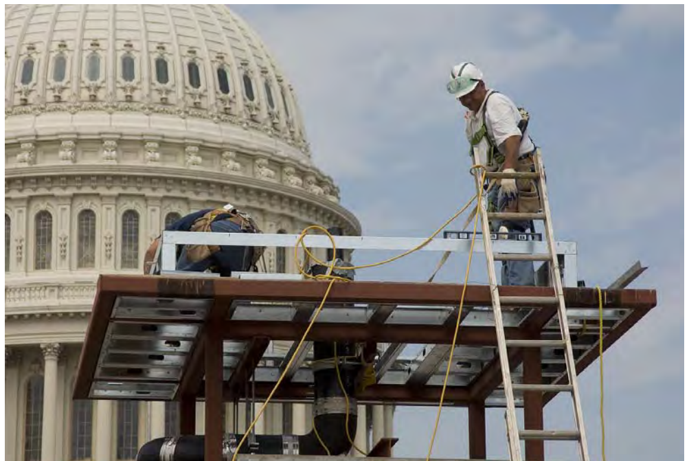
Workers assemble the framework at the top of a new elevator on the CVC roof deck.
