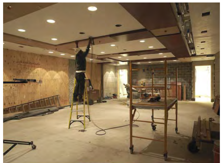
A CVC worker installs cherry wood panels to ceiling soffits in a meeting room adjacent to the Congressional Auditorium. Crews are now installing millwork and fabric ceiling and wall panels in several areas throughout the CVC.
