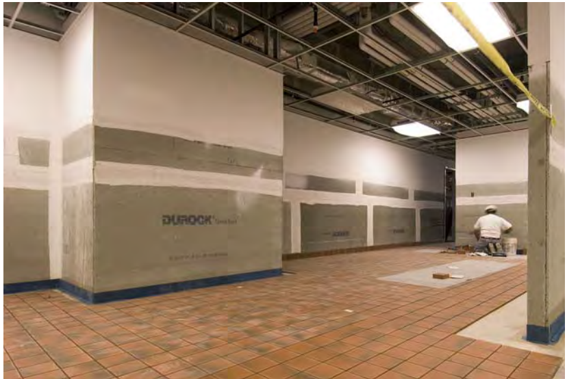
A mason (far right) completes a section of floor tile in the CVC Food Service Area.
