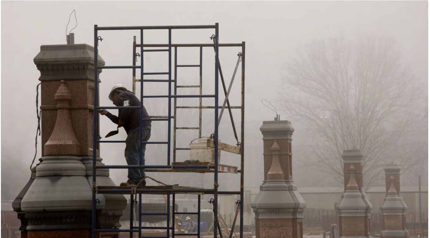
A worker applies grout to a joint between two of the granite blocks that make up one of six historic lanterns on the East Front Plaza.
