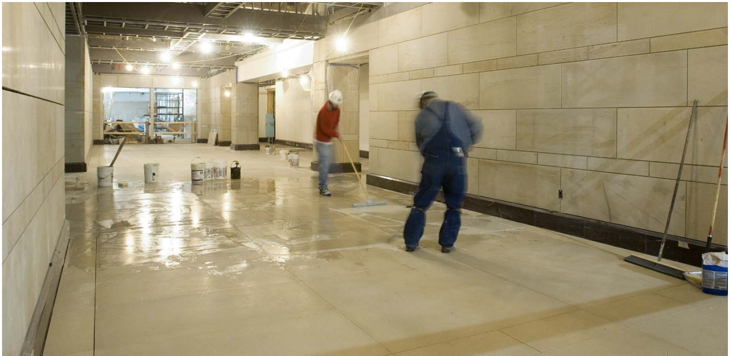
Before grouting, workers apply a liquid stone filler between dolomite floor stones in a corridor at the south end of the Great Hall.
