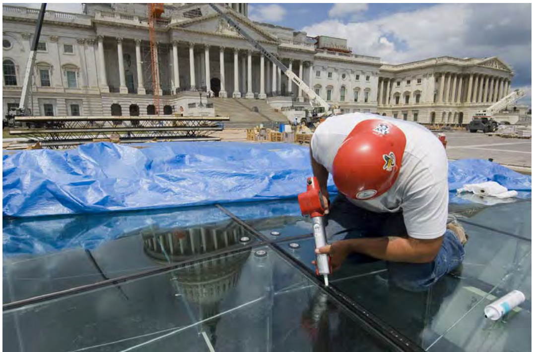
A CVC worker seals the joint between two of the glass panels of a skylight above the Great Hall.
