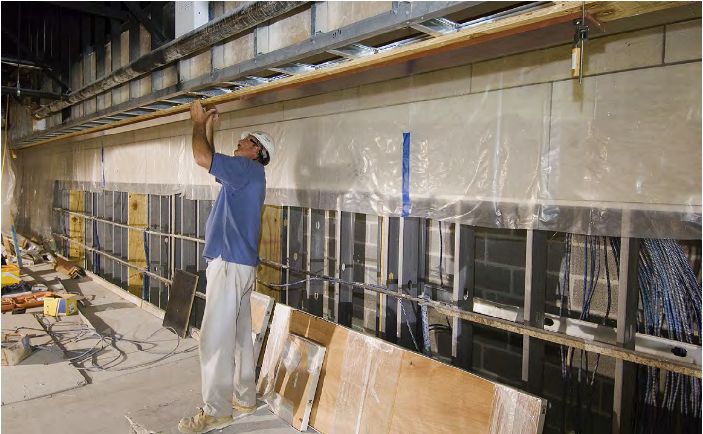
A millworker installs wood finishing trim to a ceiling soffit inside the South Orientation Theater. The trim is the first woodwork in the CVC.
