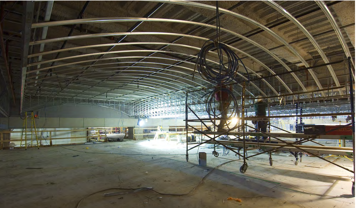
On a platform elevated 25 feet above the floor, workers continue assembling the metal framework for one of three barrel-vaulted ceiling alcoves in the Great Hall. Eventually, large light fixtures will hang below the ceiling and bounce light off a white plaster ceiling finish.
