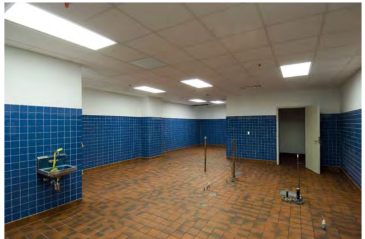
The kitchen of the CVC's new dining facility has been cleared and cleaned and is ready to receive kitchen equipment including, stoves, grills, dishwashers, sinks and other food service elements.
