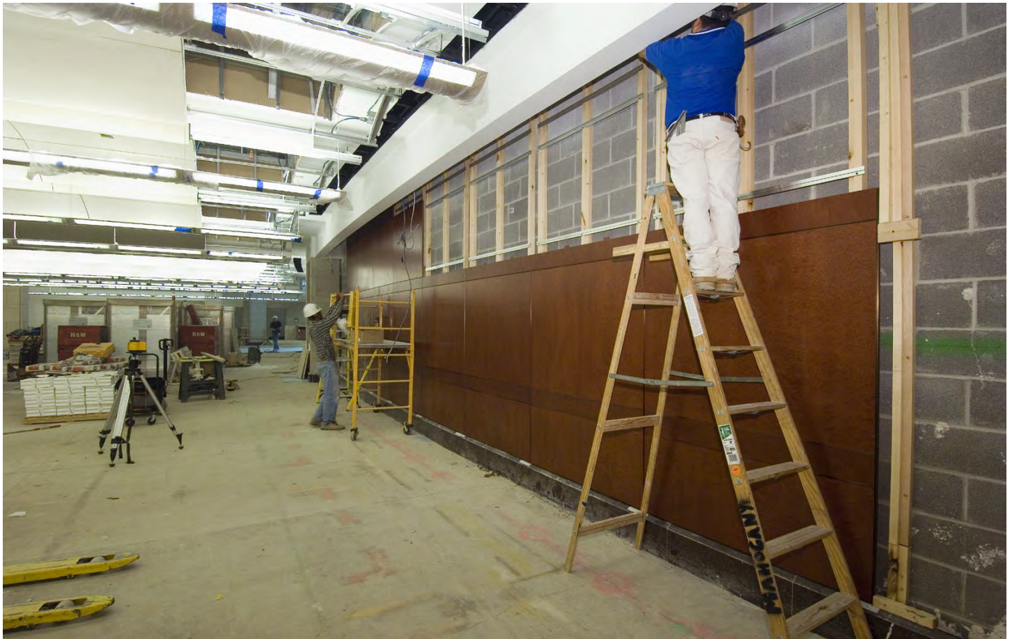
Inside the CVC's Food Service Area, carpenters install mahogany panels to a wall adjacent to the primary visitor seating zone.
