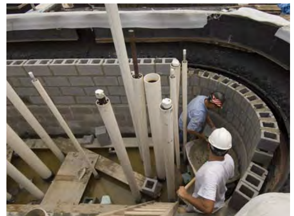
Above: Workers set masonry blocks to the inside of one of two historic fountains on the CVC plaza. The fountains will create a mist that according to the original designer, Frederick Law Olmsted, would “generate a rainbow that would frame the Capitol Dome.”
