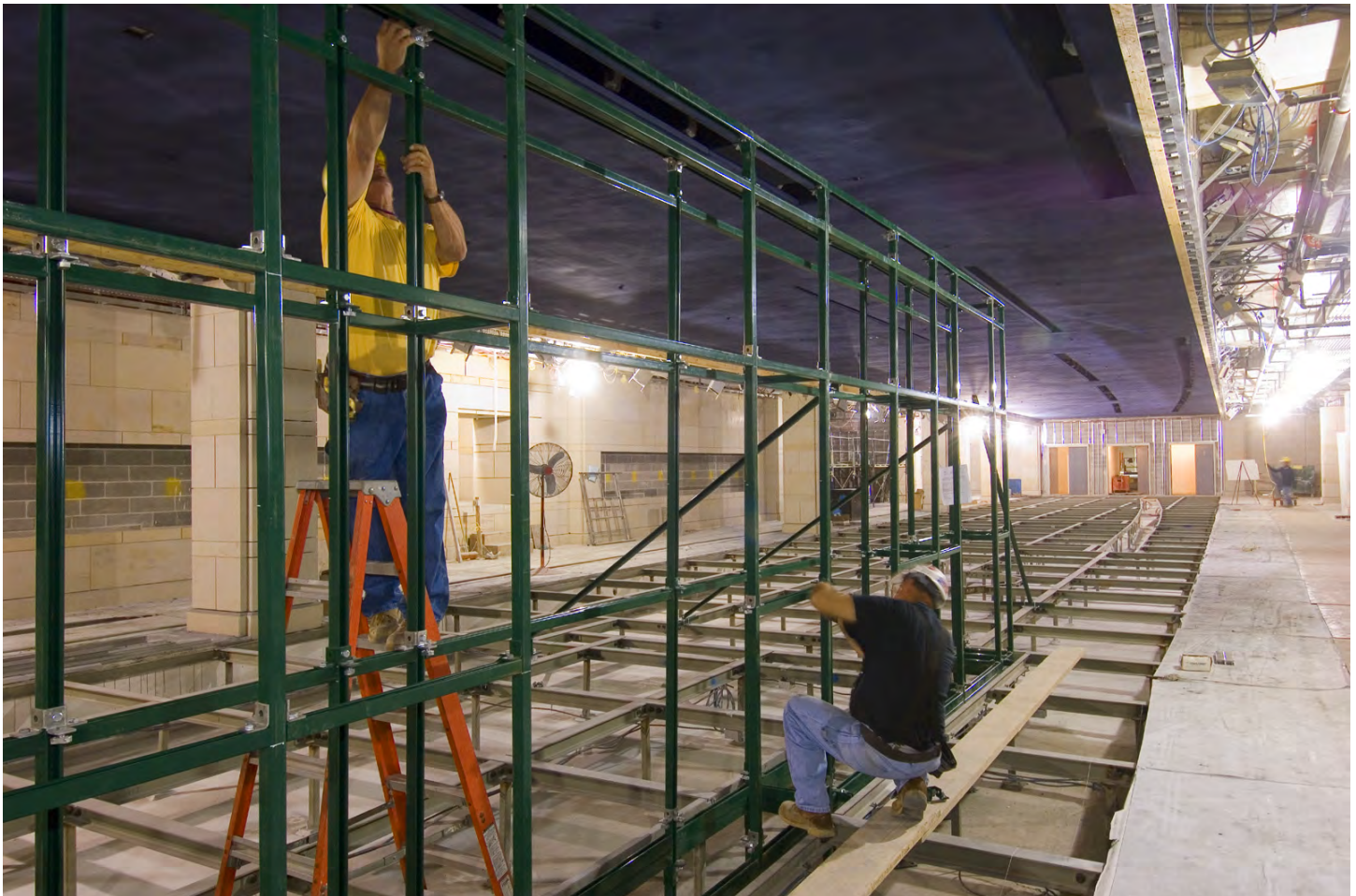
Workers install the steel framework that will support a curving marble wall in the Exhibition Hall in the Capitol Visitor Center.
