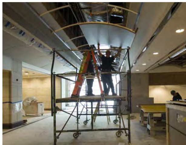
Workers install curved acoustic fabric ceiling panels in the Food Service area.
