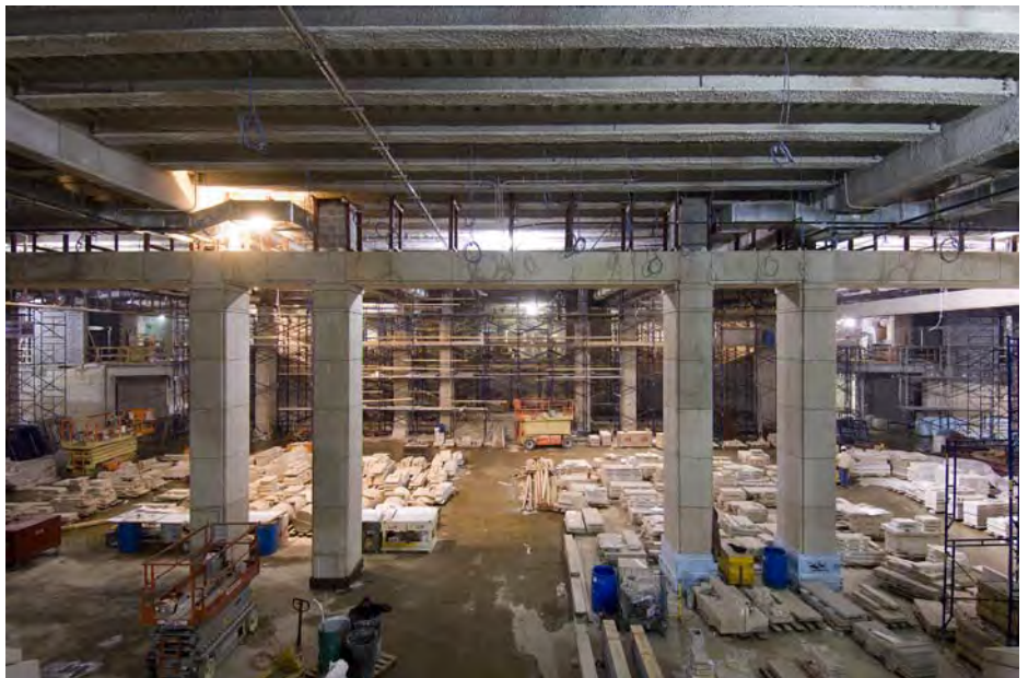
A view of the Great Hall looking east. Scaffolding will begin to rise throughout the 20,000-square-foot Hall as stone work is now complete on all 16 columns and connecting soffits.
