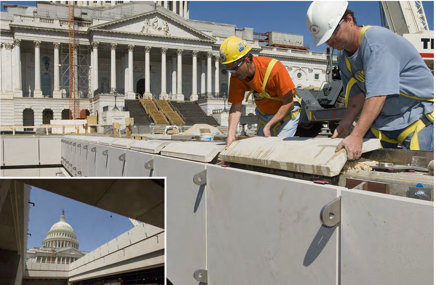
Large photo: Masons set capstones along the perimeter of the south skylight above the Great Hall. Inset: From the upper level of the Capitol Visitor Center, a view of the Capitol is framed by the south skylight opening above the Great Hall. Skylight installation begins this week.
