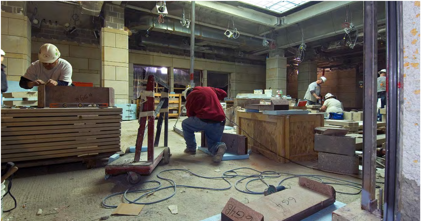
Masons execute some final cuts on Tennessee Marble base stone to be installed in the upper level lobby outside the Orientation Theaters.
