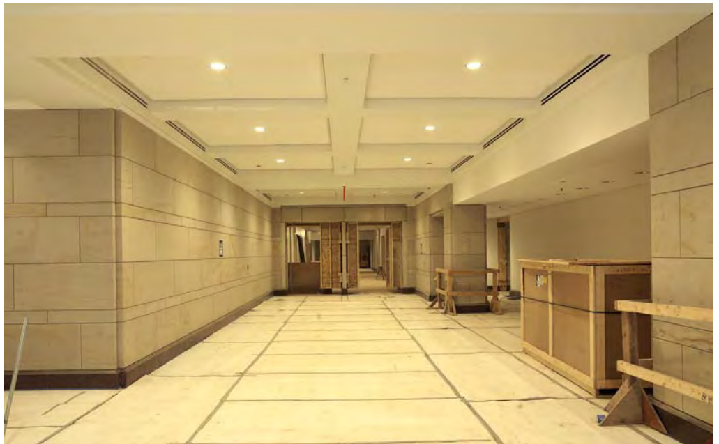
Ceiling panel installation is nearly complete in a south side corridor adjacent to the Great Hall.
