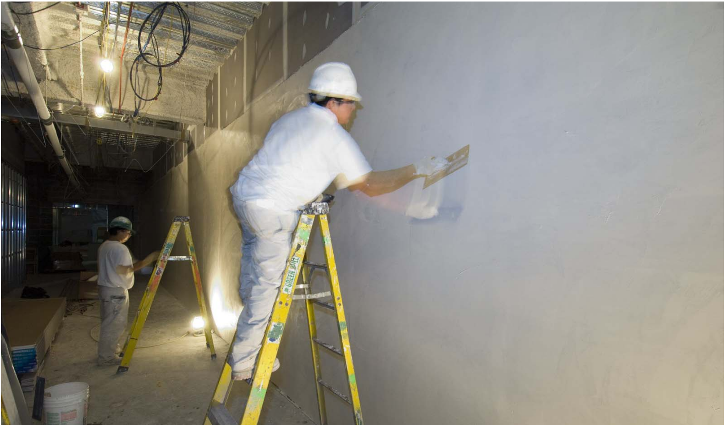
Workers apply plaster to drywall in House Expansion Space. Overall, House and Senate Expansion space encompass 170,000 square feet.
