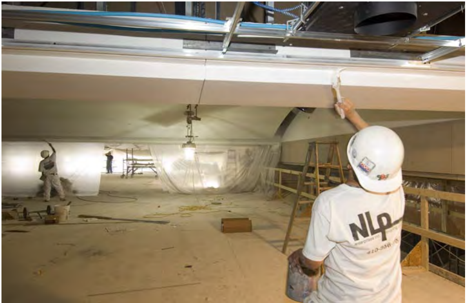
Painters complete the final touches on the soffits between the barrel-shaped ceiling vaults above the Great Hall. Crews are expected to begin dismantling the scaffolding in the Great Hall late next week, clearing the way for stone masons to begin installing 20,000 square feet of floor stone.
