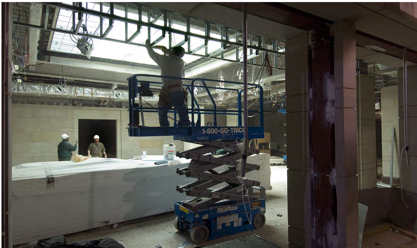
A worker installs ceiling framing around a skylight near the south Orientation Theater. Upon leaving the theater, visitors will have an unprecedented view of the Capitol Dome, which, from that location, towers to height of 305 feet to the top of the statue of Freedom.
