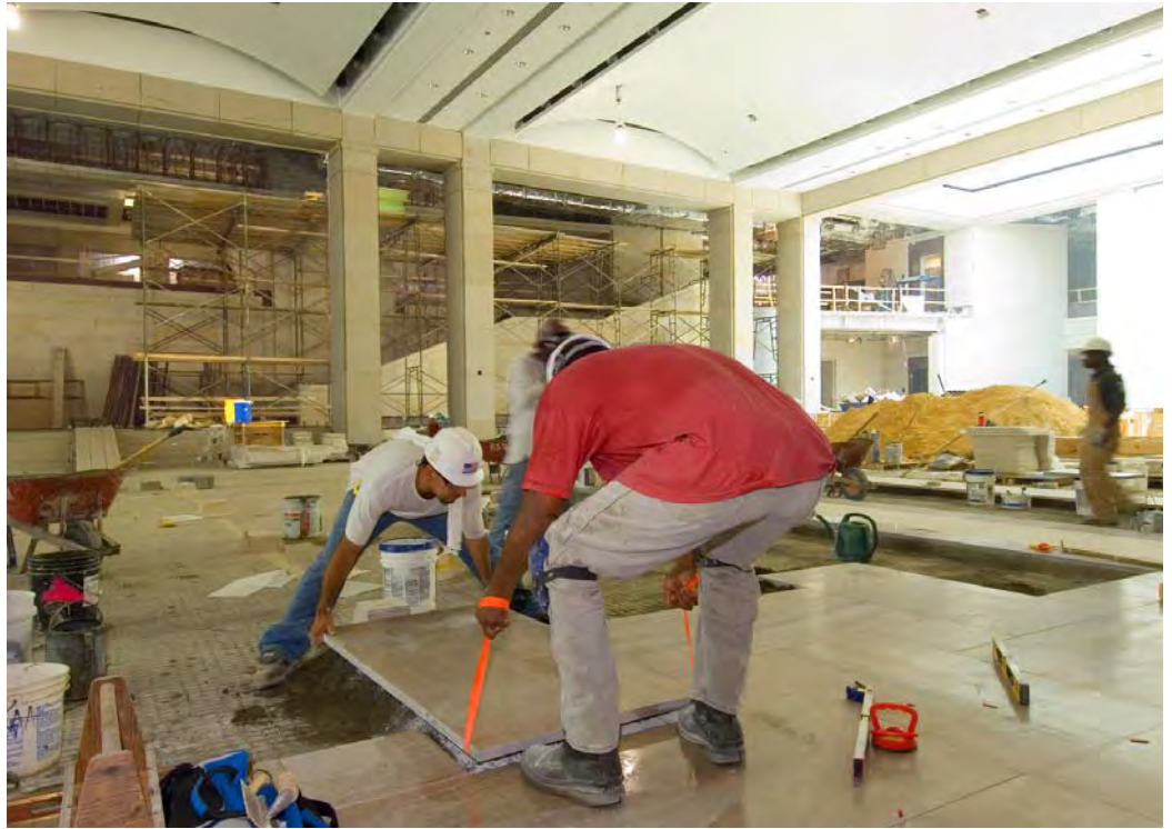
Masons set a block of Tennessee Marble in the center of the Great Hall. A mockup of the stonework has been approved by the project architect and masons are now working out to all four corners of the Great Hall, an area that encompasses 20,000 square feet, nearly three times the floor space of the Capitol's Rotunda.
