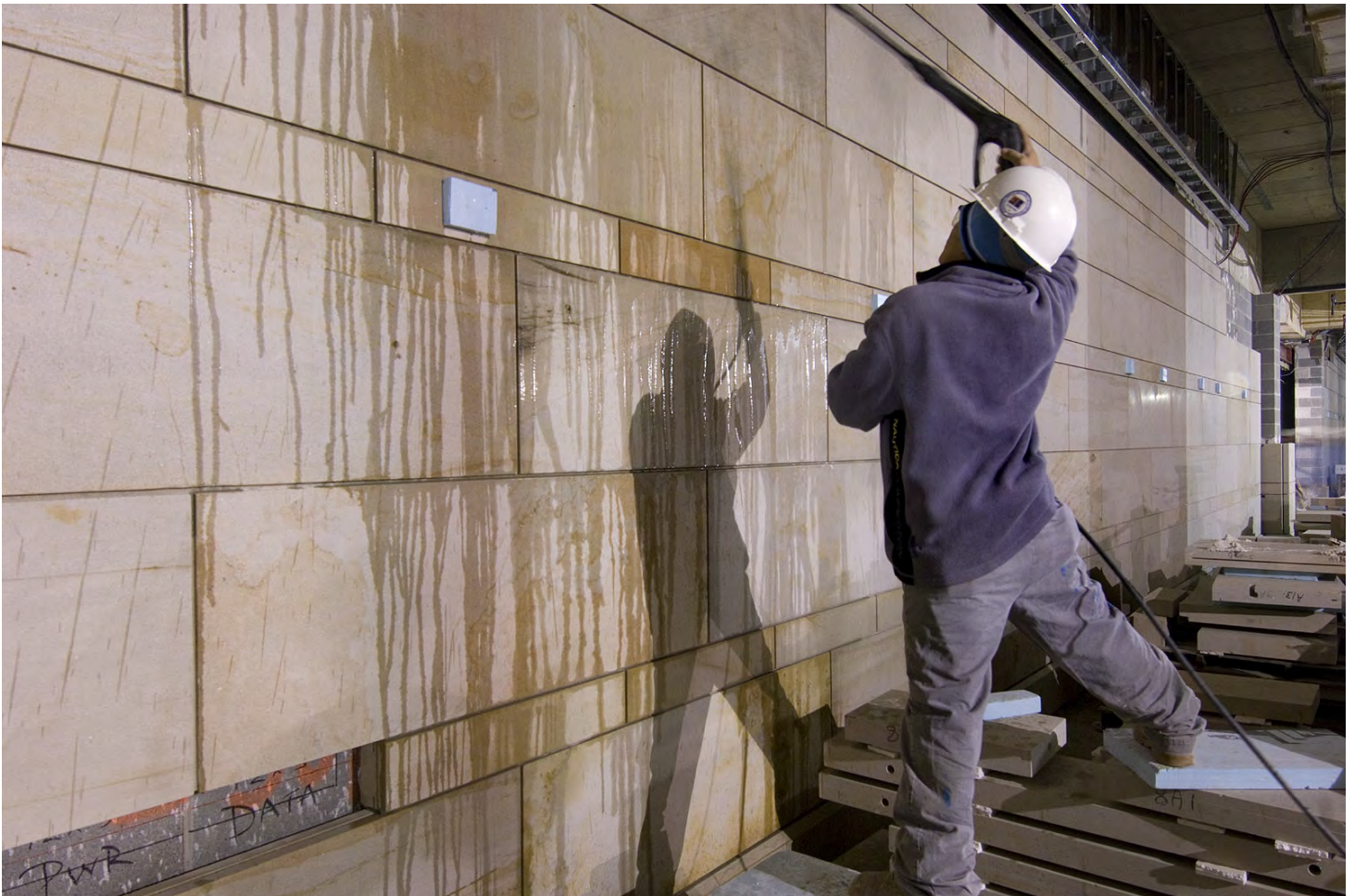
A worker uses a power washer to clean a sandstone wall in the CVC Exhibition Hall. Floor stone installation will begin in the facility next week.
