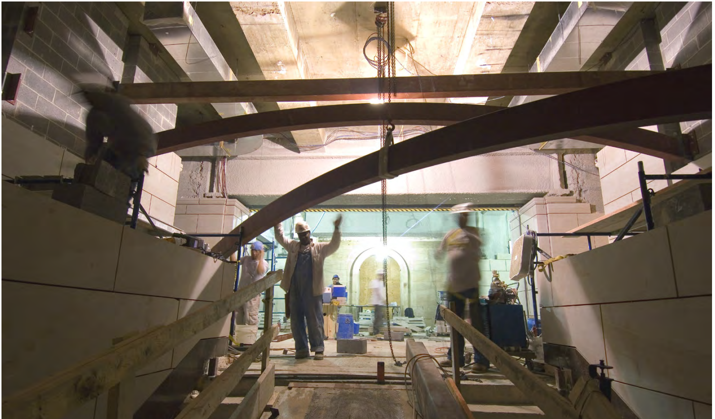
CVC workers position a steel beam arch in the East Front Extension of the Capitol. The beam is part of the steel framework that will span two escalators and the main staircase that connect the CVC to the Capitol. The framework will support blocks of sandstone that will cover much of the ceiling.
