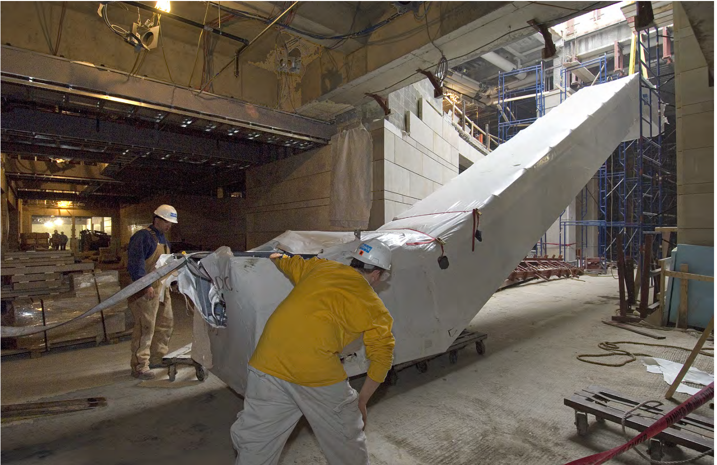
Capitol Visitor Center workers guide an escalator truss (mechanical support system) through a skylight in the Great Hall. The escalator will be situated at the south end of the Great Hall. Overall, the Visitor Center includes six escalator banks and 23 elevators.
