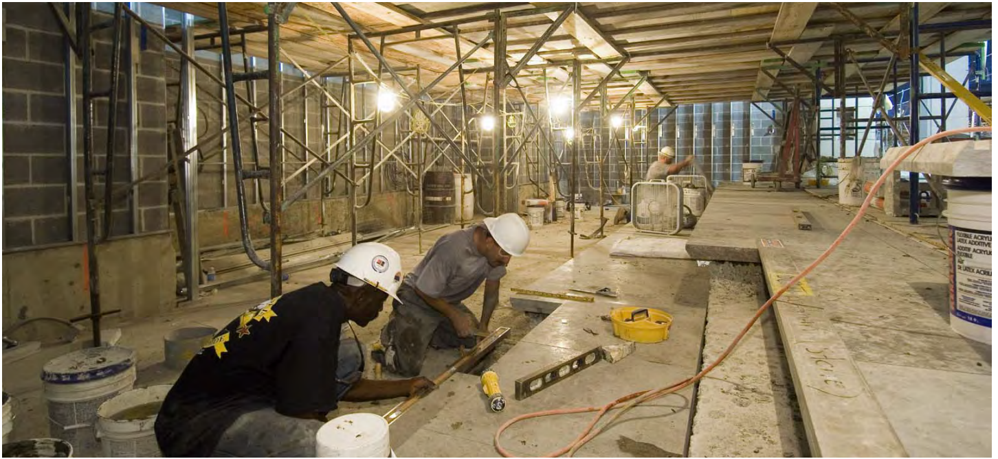
Masons set the stepping stones for the Virtual Senate Theater in the CVC's Exhibition Hall.
