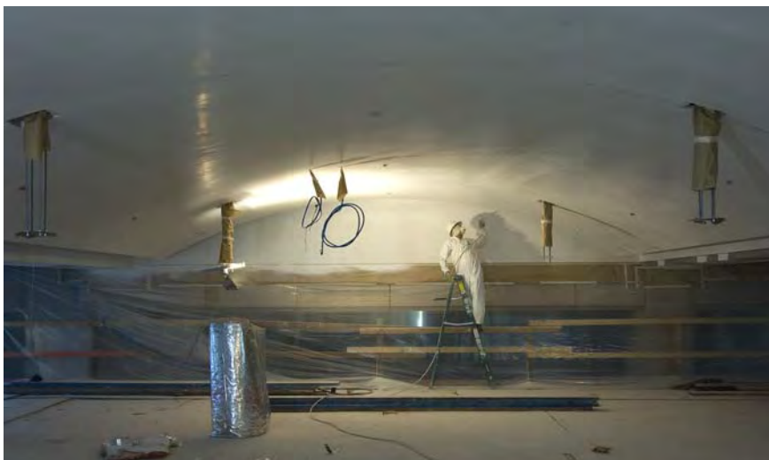
A worker applies the first coat of paint to a plaster ceiling above the Great Hall.
