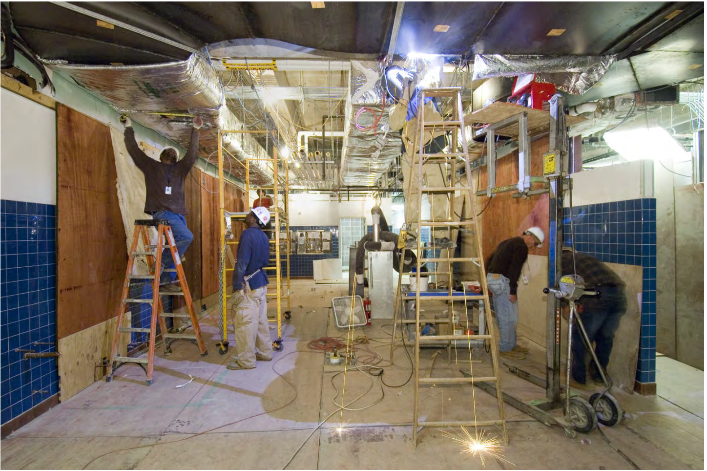
Workers make adjustments to a very complex system of air duct in the kitchen of the CVC's Food Service Area.
