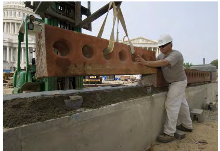
A mason sets historic stone to the seatwall around the Senate Egg.
