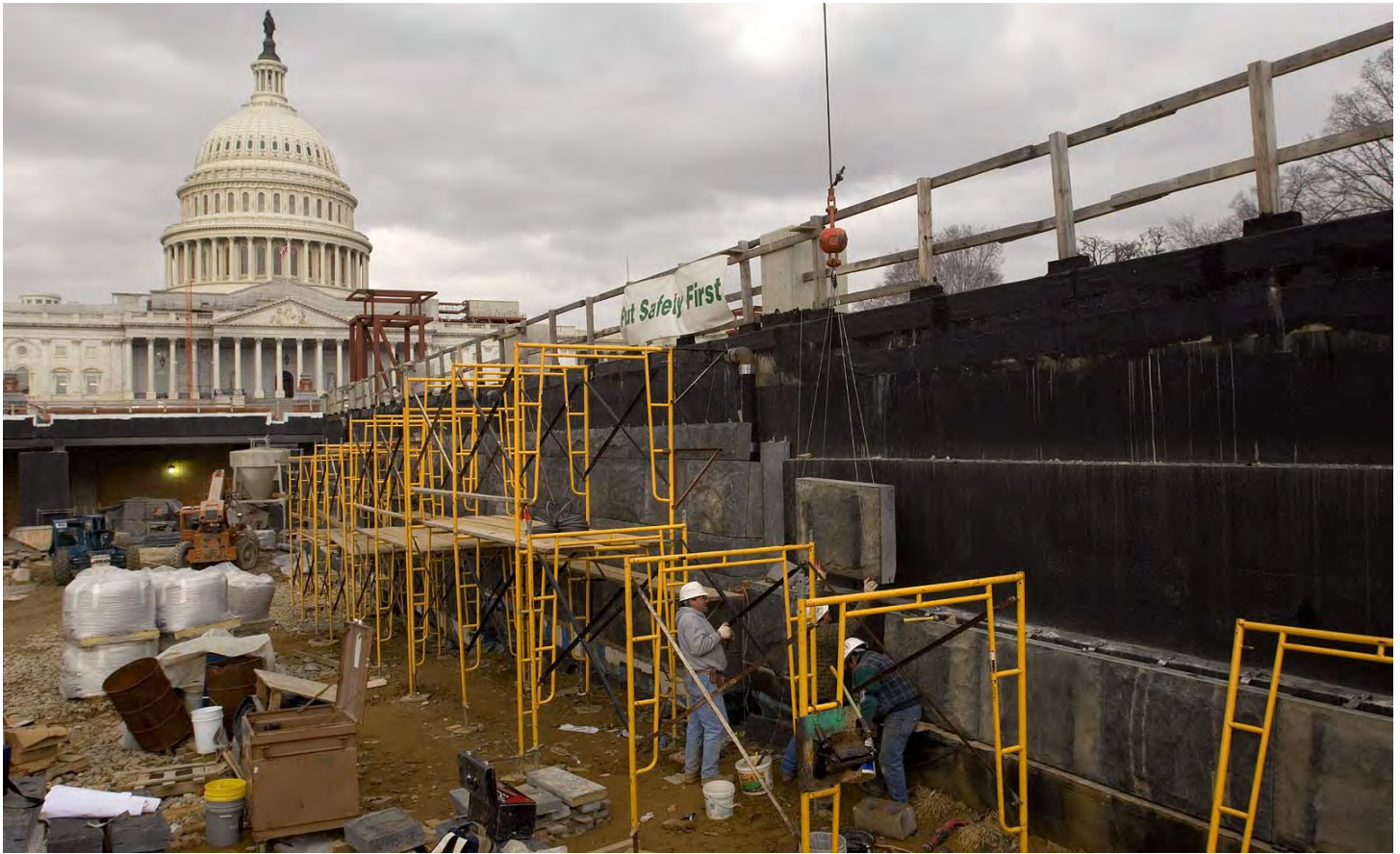
Stone masons set a rough-cut granite block to the south exterior wall of the Congressional Auditorium. The wall and adjacent concrete work need to be completed early this spring to clear the way for the planting of two rows of Tulip Poplar trees that will line a stepped path leading to the CVC entrance.
