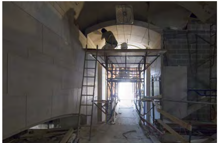
A mason applies grout between stones in the East Front transition zone, in an area that use to serve as a carriageway below the East Front center steps.
