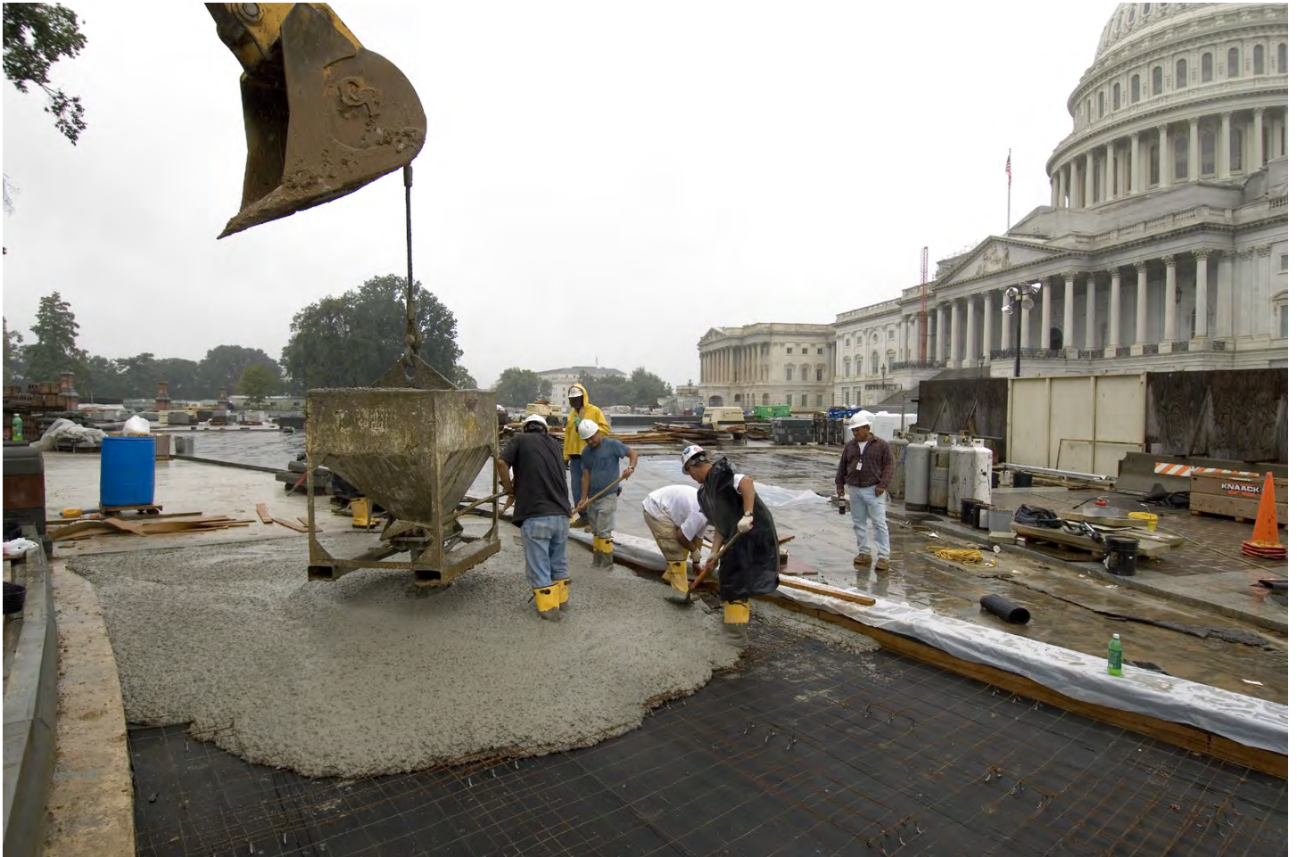
Workers spread out newly poured concrete for the foundation of a sidewalk around the Senate-side seat wall.
