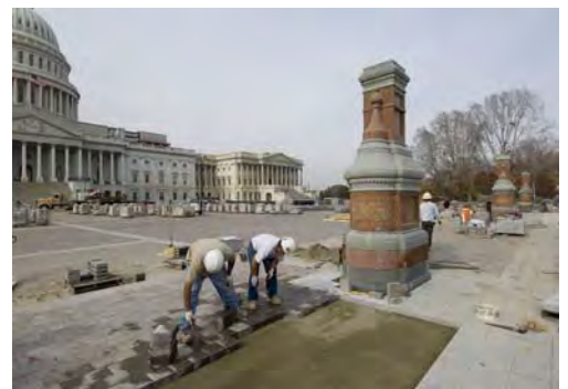
Masons have resumed setting pavers around the historic Olmsted lanterns on the East Front Plaza.
