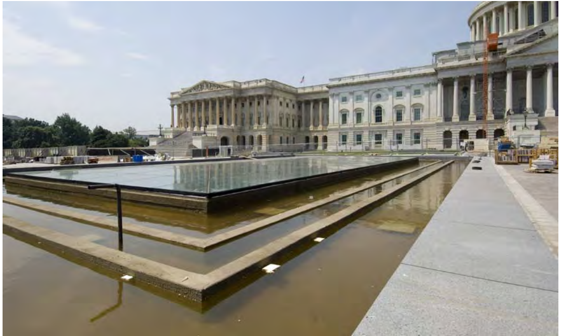
A pool of water sits within an 8-foot-wide basin surrounding one of the two large Great Hall skylights to test the waterproofing membrane within the basin. Eventually, a pool of water will slowly revolve around a black granite slab that will rest on the pedestal walls visible in the center of the basin.
