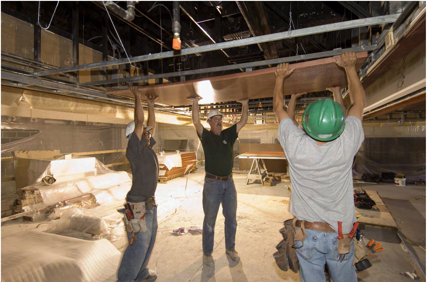
Workers position a wood acoustic ceiling panel to the ceiling grid in the North Orientation Theater.
