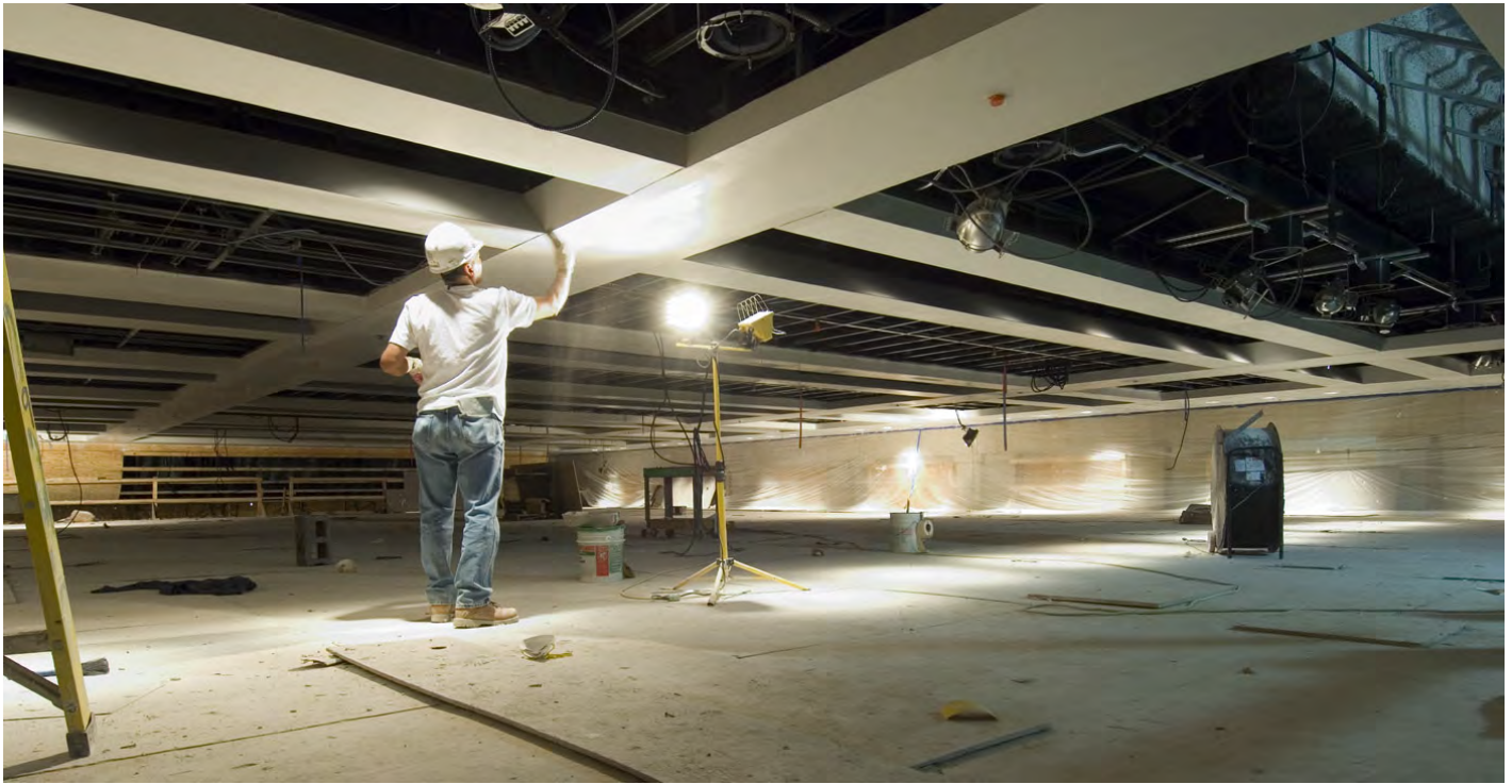
A worker applies plaster to the ceiling framework above the Congressional Auditorium. Painters are expected to finish the ceiling next week.
