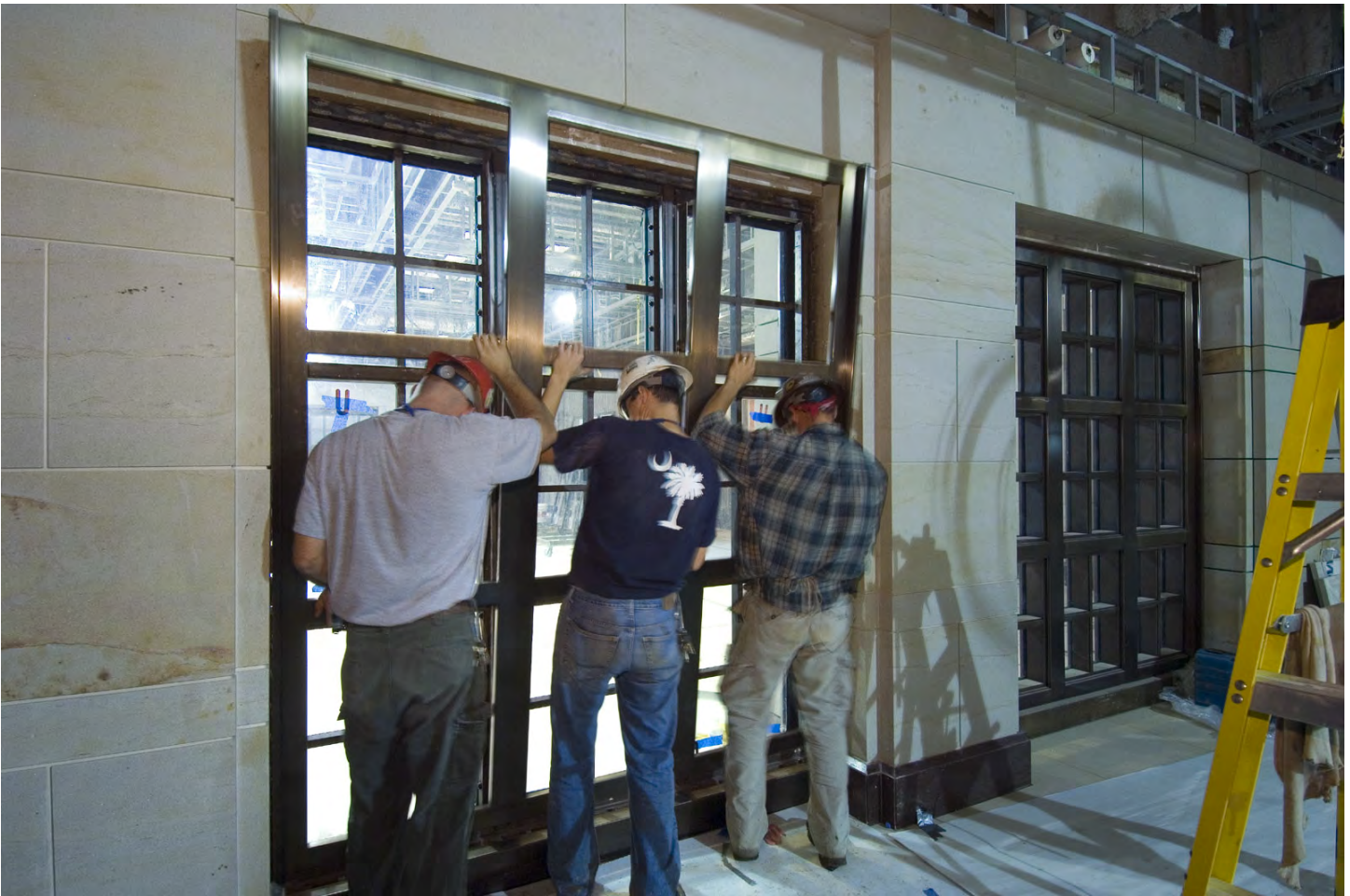
Workers install a bronze frame to a steel window structure in the CVC entrance zone.
