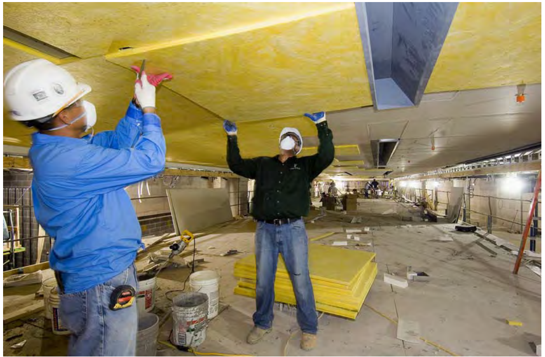
Workers install insulation board to the ceiling of the CVC Exhibition Hall. This work will be completed this week and plaster work is expected to begin early next week.
