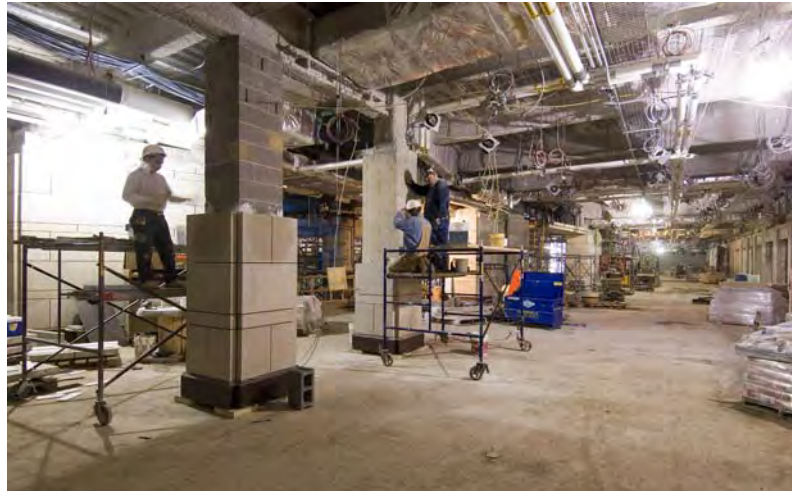
Masons are nearing completion of stone installation in the upper level east lobby that looks over the Great Hall. Several mason teams will then move to the other side of the Great hall to work in the East Front transition zone between the CVC and the Capitol Building.
