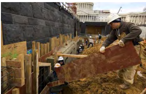
Along the north wall of the Congressional Auditorium, workers assemble formwork for a concrete foundation that will support a stepped walkway leading to the CVC entrance.
