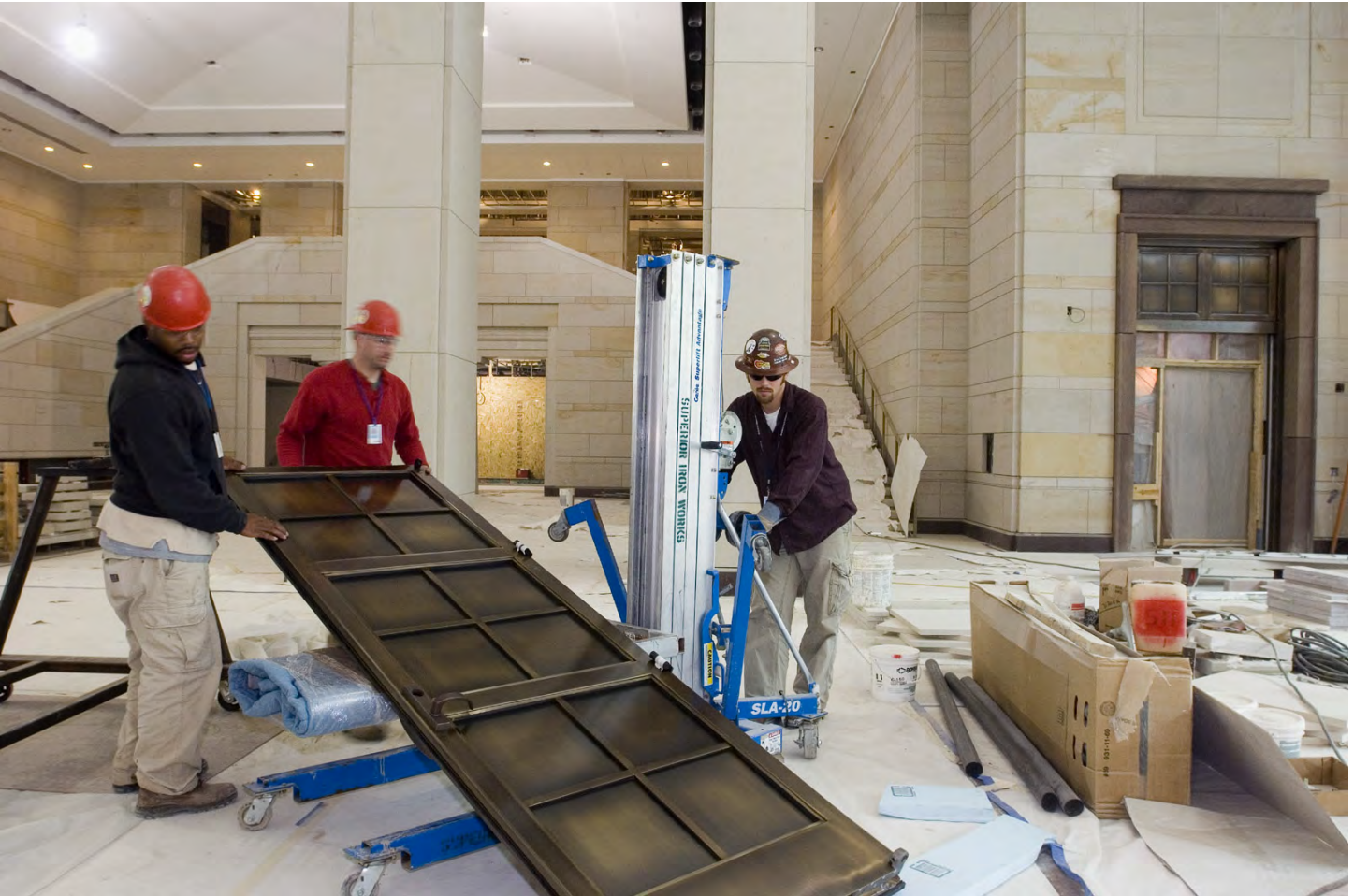
A crew raises one of the two bronze doors for the North Orientation Theater visitor entrance. The entrance threshold is framed with burgundy sandstone (right of photo) to match similar stone work around both of the north and south entrances of the Capitol Rotunda.
