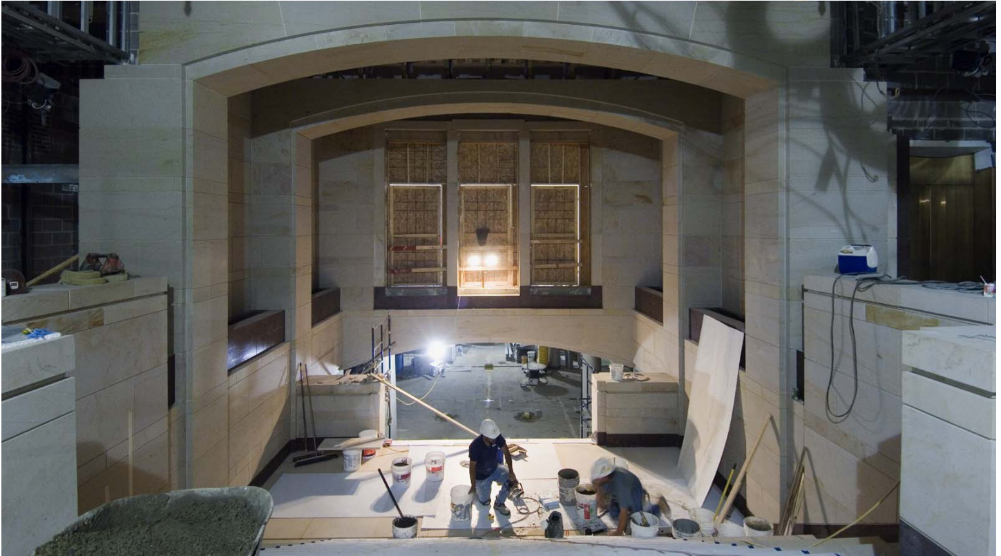
Masons set stone at the base of a staircase leading to the entrance of a new Congressional Auditorium located below the East Capitol Street Extension.
