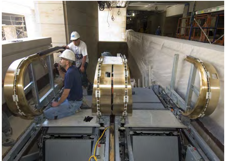
Workers assemble a portion of the escalators on the south side of the Great Hall.
